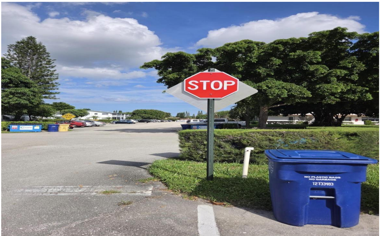
CANTERBURY A- FADED STOP SIGN REPLACED BY HANDYMAN JOSE.
