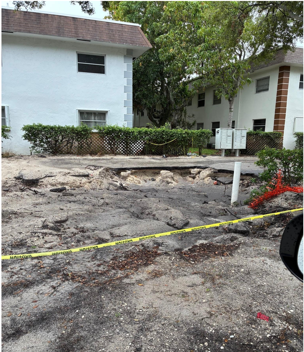
STRATFORD A- THIS CRATER CONTINUES TO WIDEN. SECTIONS OF UNDERMINED ASPHALT ROAD HAVE COLLAPSED. REPAIR WORK WILL HAPPEN SOON.
