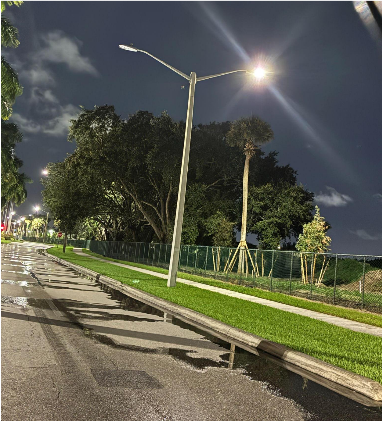
CENTURY BOULEVARD- DARK STREETLIGHT, DISCOVERED 8/30. A REQUEST FOR REPAIR WAS SENT TO FPL, TICKET #48548.
