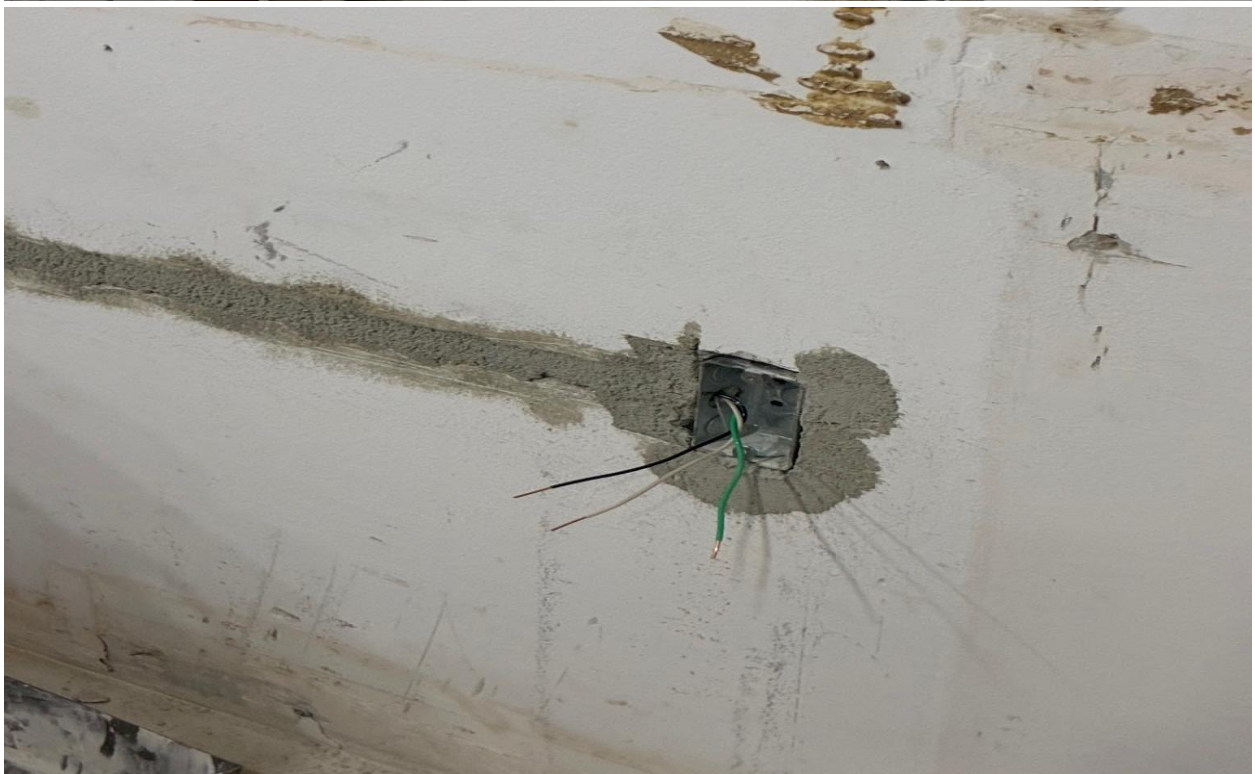
121 WELLINGTON G- INSTALLATION OF OUTLETS, DAMAGE TO COMMON ELEMENT WALL.
