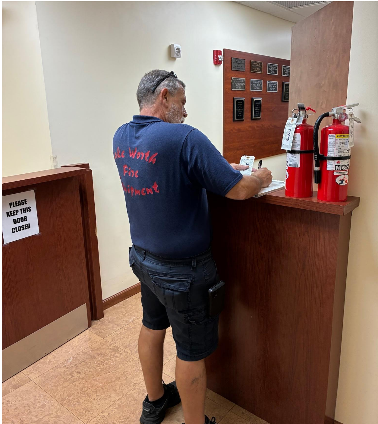
UCO OFFICE- ON 8/24, LAKE WORTH FIRE EQUIPMENT INSPECTED AND SERVICED FIRE EXTINGUISHERS AT THE FIVE BUILDINGS OWNED BY UCO.
