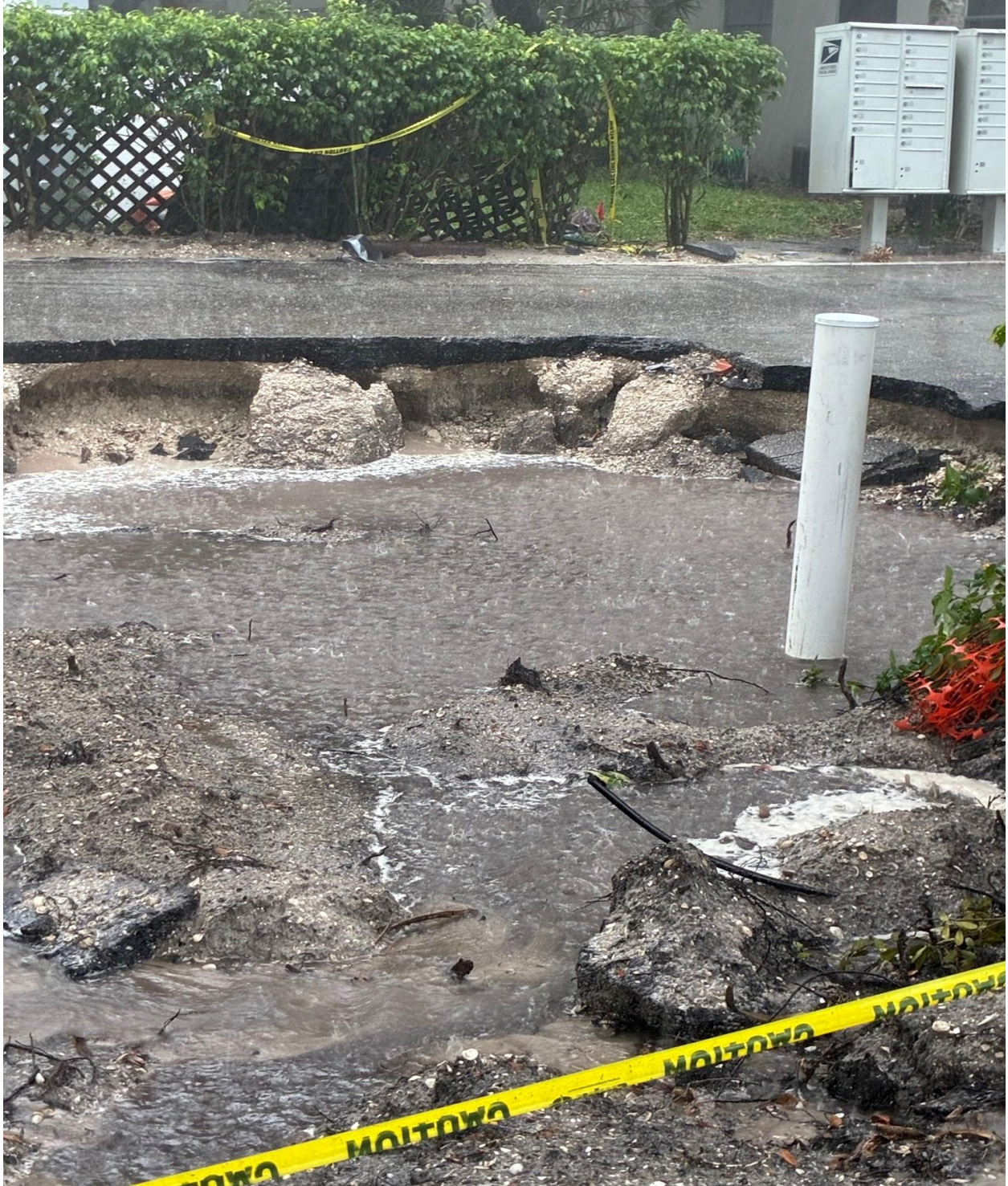
STRATFORD A- LAST WEEK'S TORRENTIAL RAINS ARE WASHING OUT THIS CRATER AND UNDERMINING THE ROAD. THIS SITUATION HAS BECOME CRITICAL.
