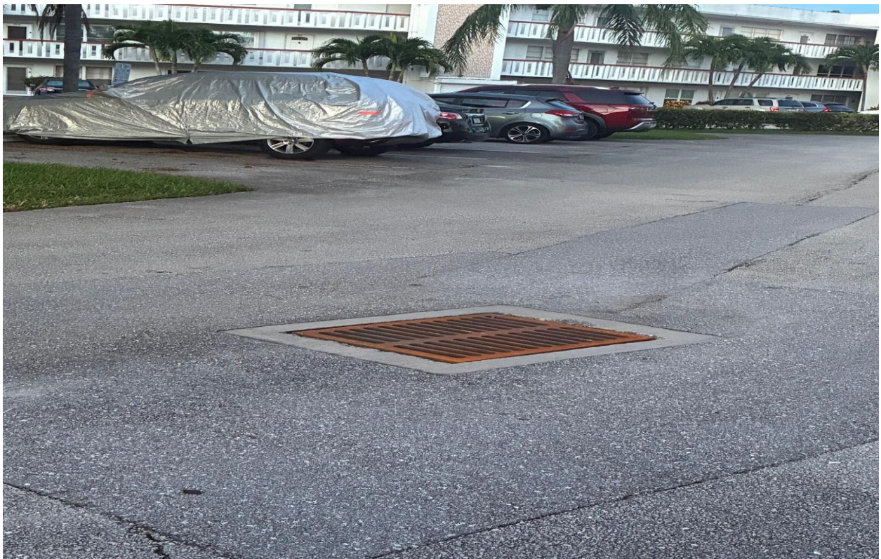
WELLINGTON CIRCLE- THIS CRACKED STORM DRAIN GRATE WAS REPLACED BY FEDERAL MAINTENANCE ON 8/4.
