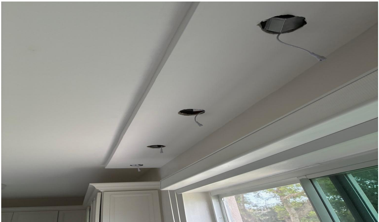
201 GREENBRIER B- RECESSED LIGHTING BEING INSTALLED. NO PERMIT. NO GOOD.
