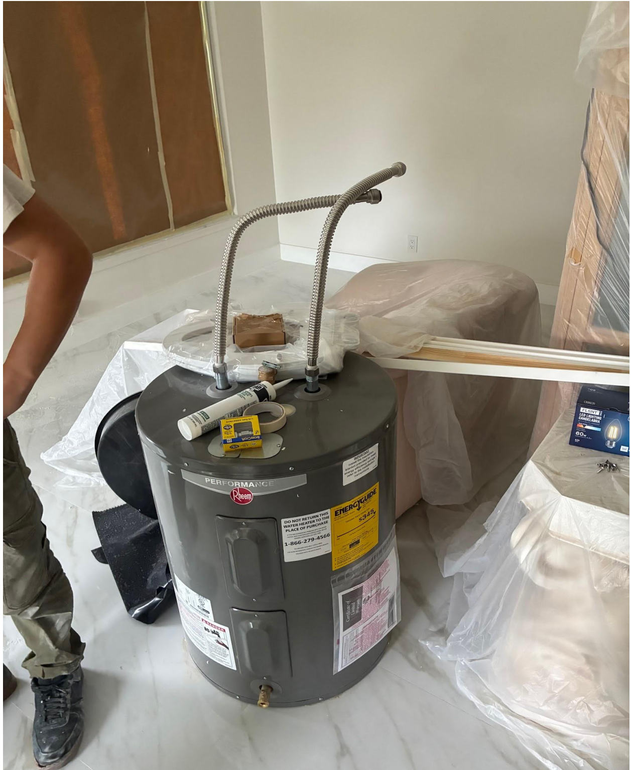
201 GREENBRIER C- HOT WATER HEATER WAITING TO BE INSTALLED. NO PERMIT. NO GOOD.
