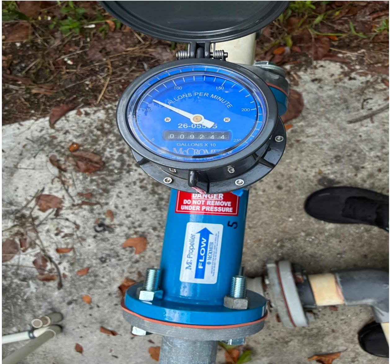
STRATFORD SECTION- NEW IRRIGATION FLOWMETER INSTALLED BY CHABOT IRRIGATION.
