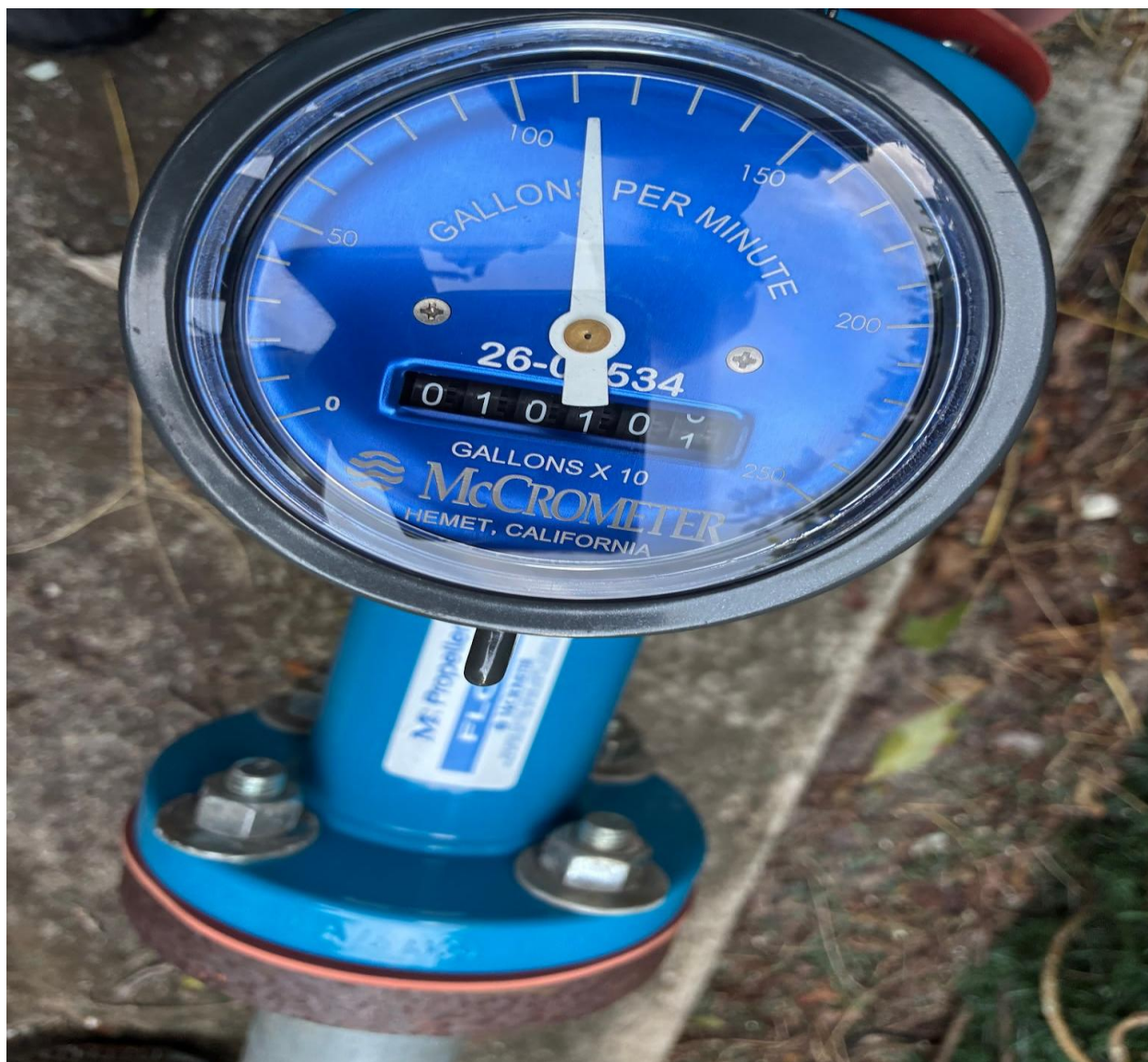
ANDOVER SECTION- NEW IRRIGATION FLOWMETER INSTALLED BY CHABOT IRRIGATION.
