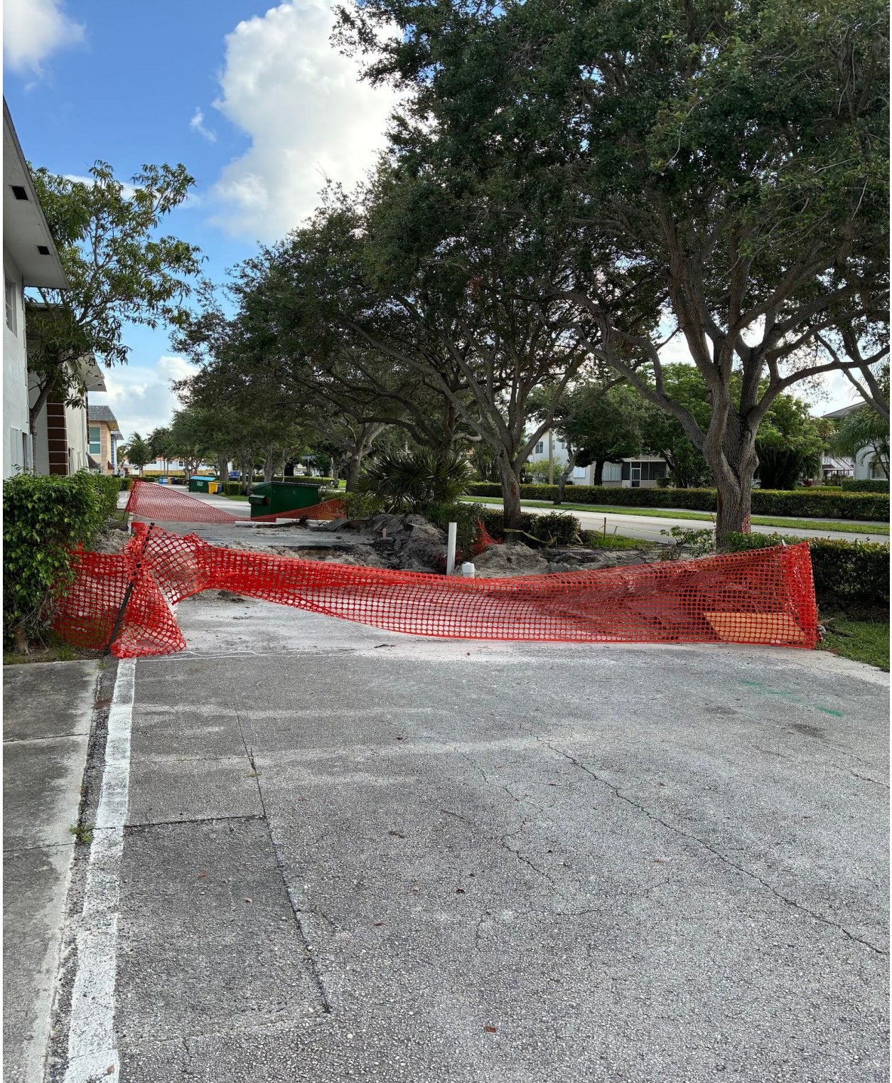
STRATFORD SECTION- THIS SECTION OF ROAD HAS BEEN BUSTED UP AND FENCED OFF FOR MONTHS.
