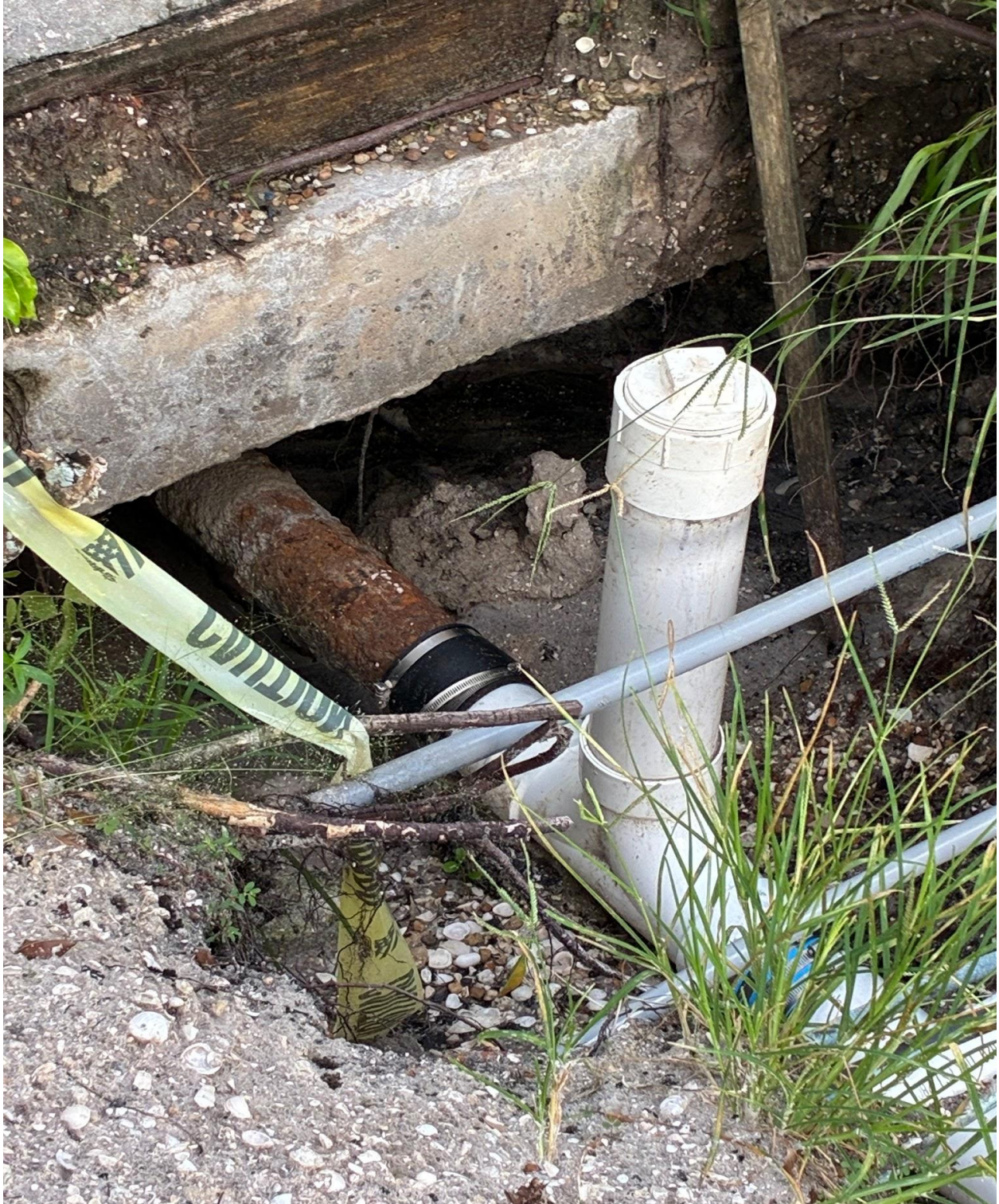
STRATFORD A- THIS IS WHERE THE NEW PVC PIPE WAS CONNECTED TO THE ORIGINAL CAST IRON PIPE. FIFTY-SIX YEAR OLD CAST IRON PIPE IS LIKELY TO BE BRITTLE AND CRACKED.
