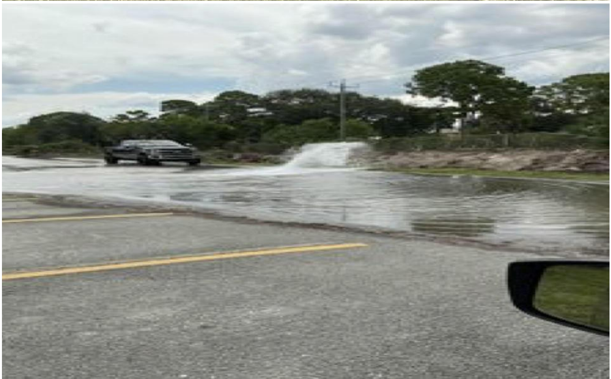
NORTH CANAL- OUR CONTRACTOR CRACKED A WATER MAIN FIRST DAY. PBC WATER MADE THE REPAIR.
