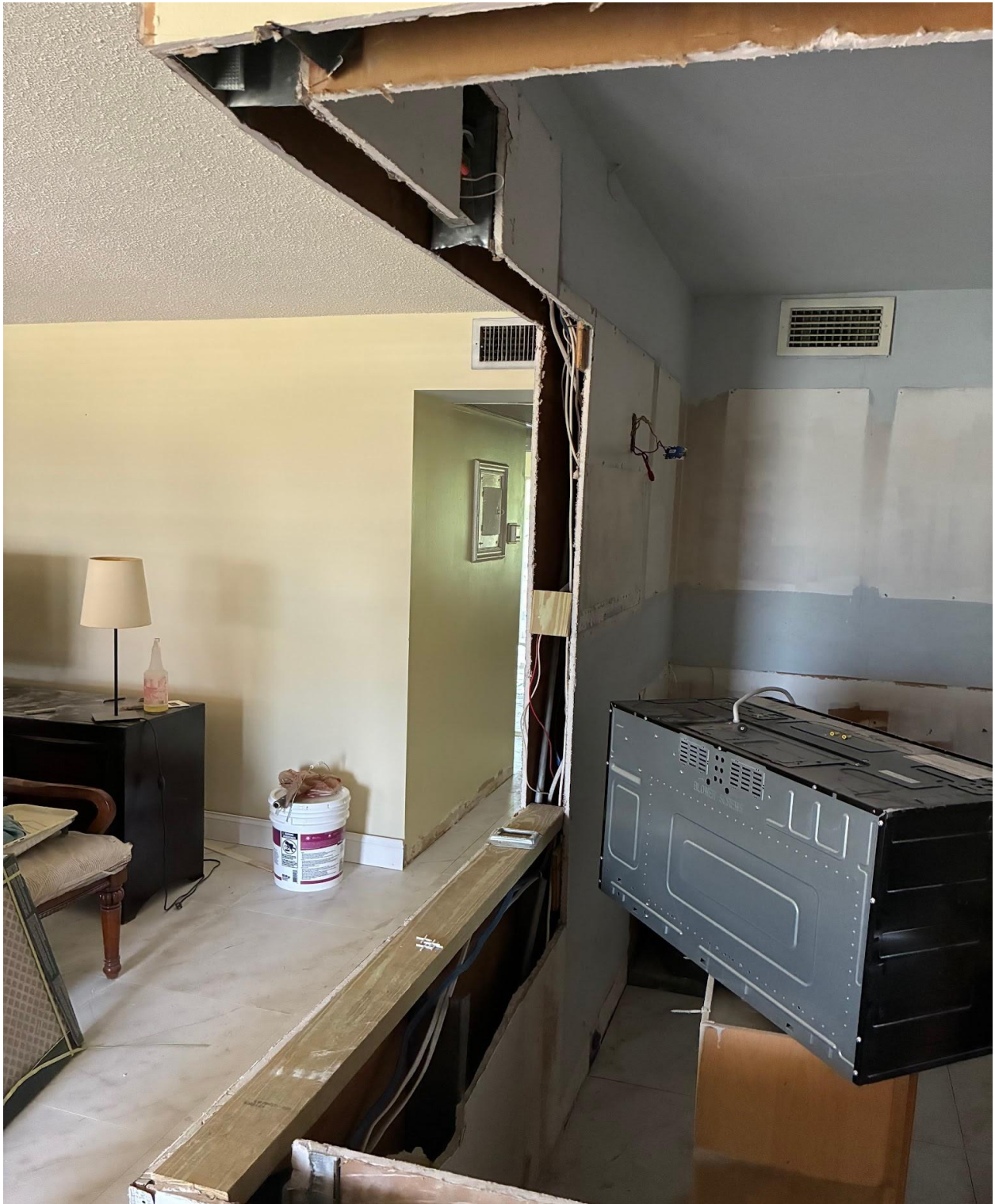
226 DORCHESTER J- INTERIOR WALLS REMOVED. NO PERMIT. NO PRIOR PERMISSION FROM THE BOARD. NO GOOD.
