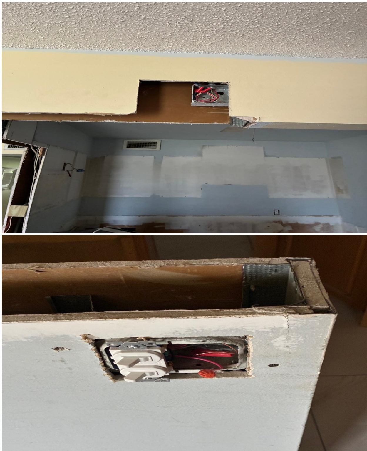
226 DORCHESTER J- UNPERMITTED, NON-CODE COMPLIANT ELECTRICAL WORK.
