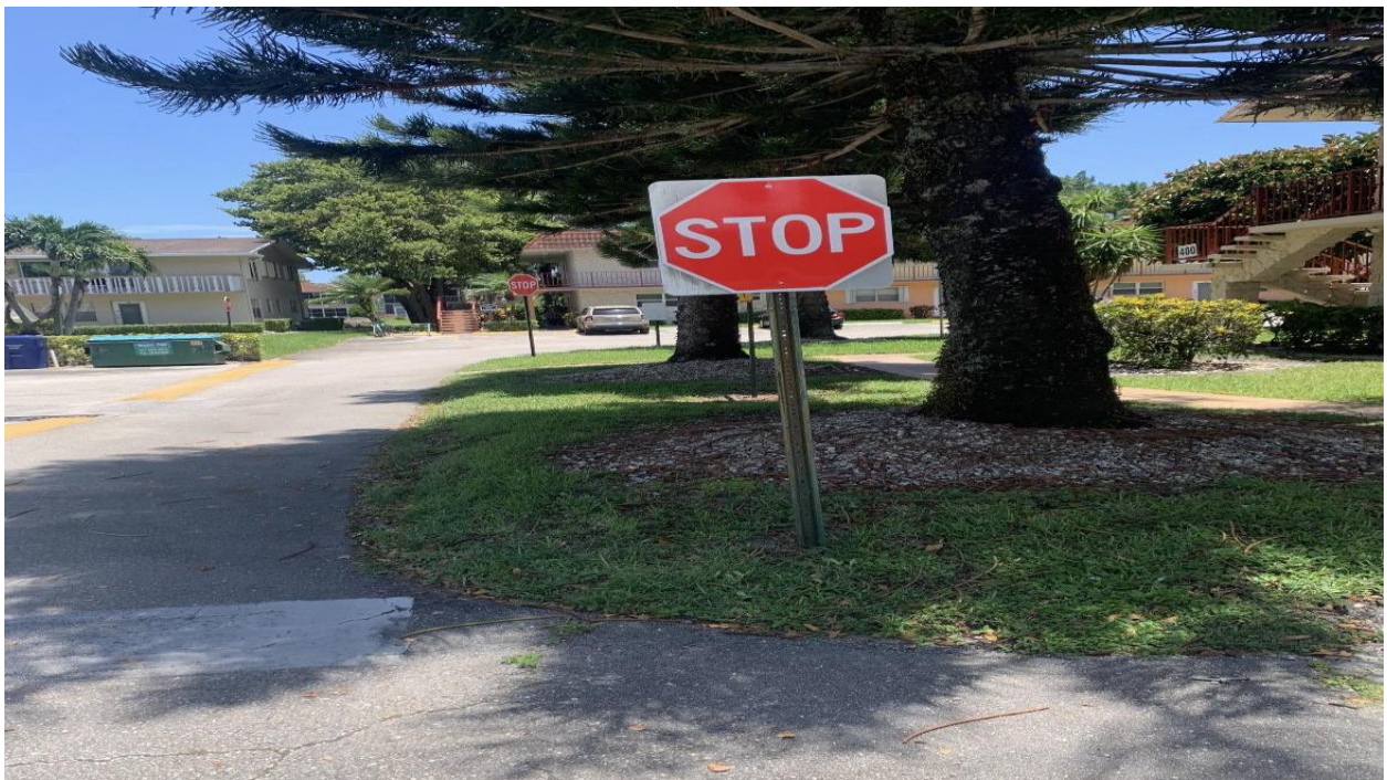
OXFORD SECTION- FADED STOP SIGN REPLACED BY HANDYMAN JOSE.
