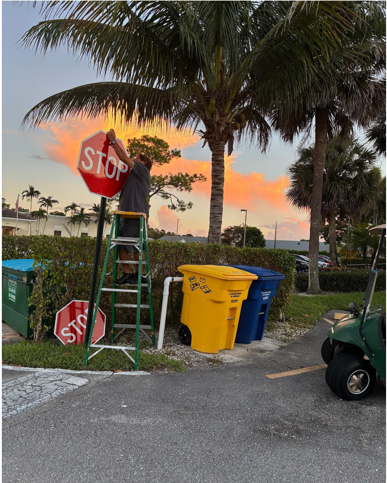
HASTINGS SECTION- FADED STOP SIGN REPLACED BY HANDYMAN JOSE.
