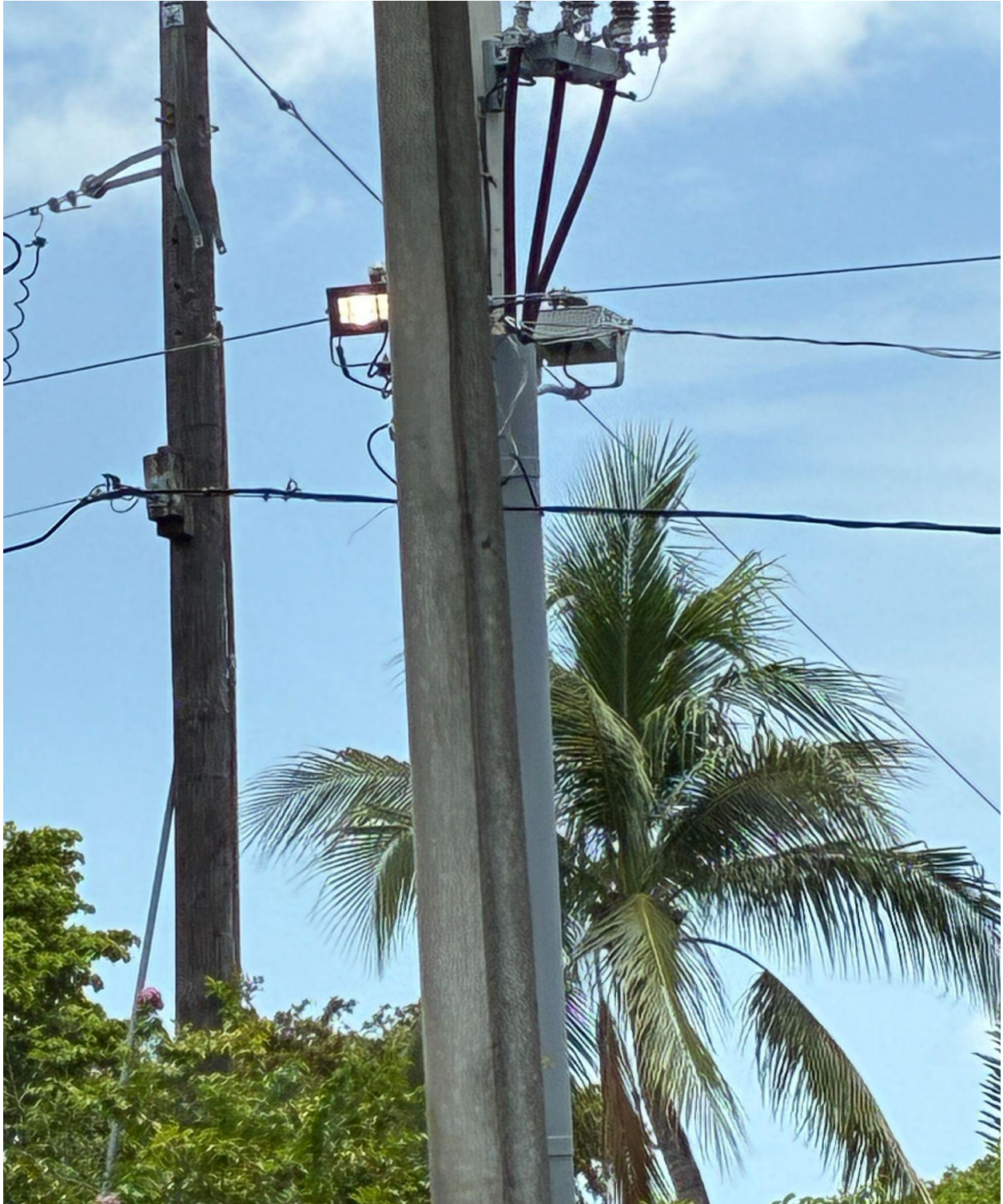
UCO OFFICE- DAYBURNER FLOODLIGHT. A REQUEST FOR REPAIR WAS SENT TO FPL, TICKET #46661.
