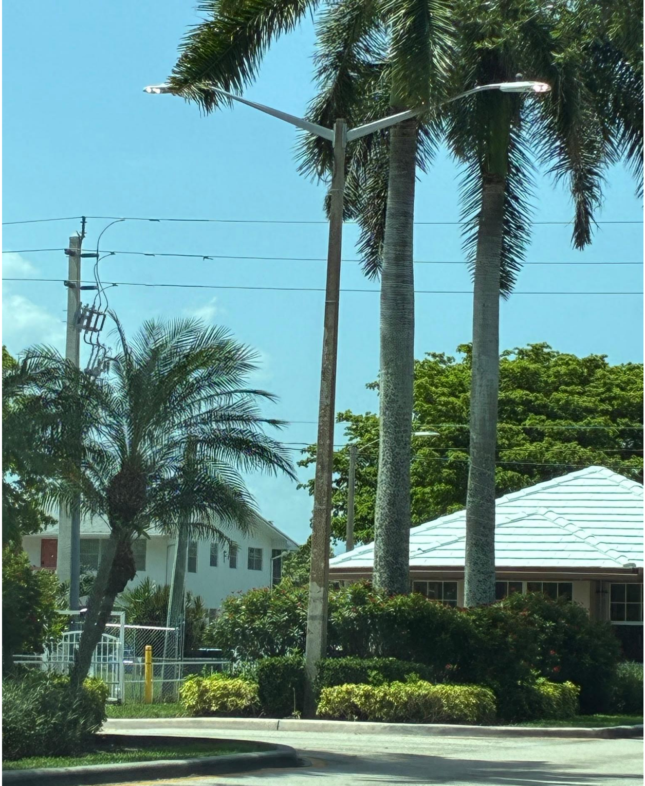
WEST DRIVE- DOUBLE DAYBURNER. REQUEST FOR REPAIR SENT TO FPL, TICKET #46721.
