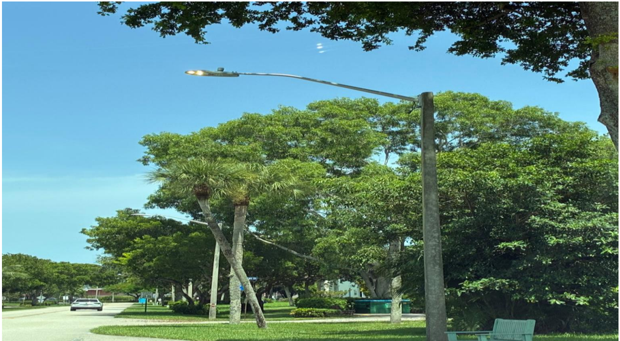
SOUTH DRIVE, BEDFORD SECTION- TWO DAYBURNERS. REQUEST FOR REPAIRS SENT TO FPL, TICKET #46723 .
