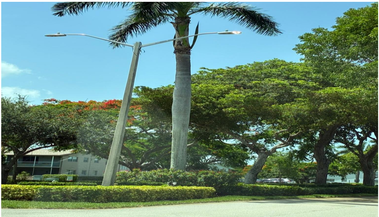
WEST DRIVE- DAYBURNERS. REQUEST FOR REPAIR SENT TO FPL, TICKET #46725.
