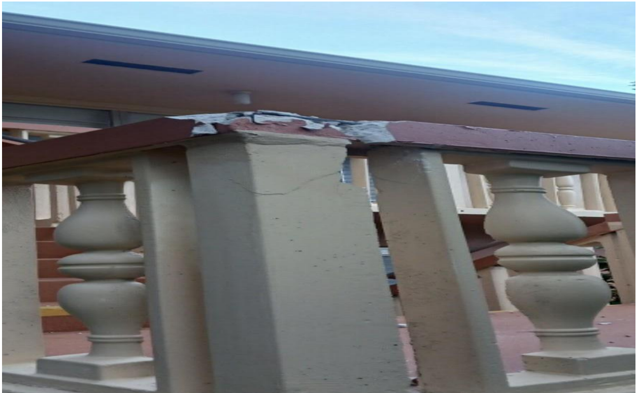
SALISBURY I- ON 7/3, LIGHTNING STRUCK THIS STAIRCASE, CAUSING MINOR DAMAGE.
