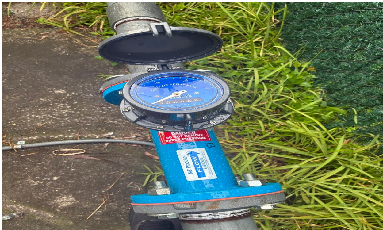
SOUTHAMPTON, WELLINGTON SECTIONS- NEW FLOWMETERS INSTALLED BY CHABOT IRRIGATION.
