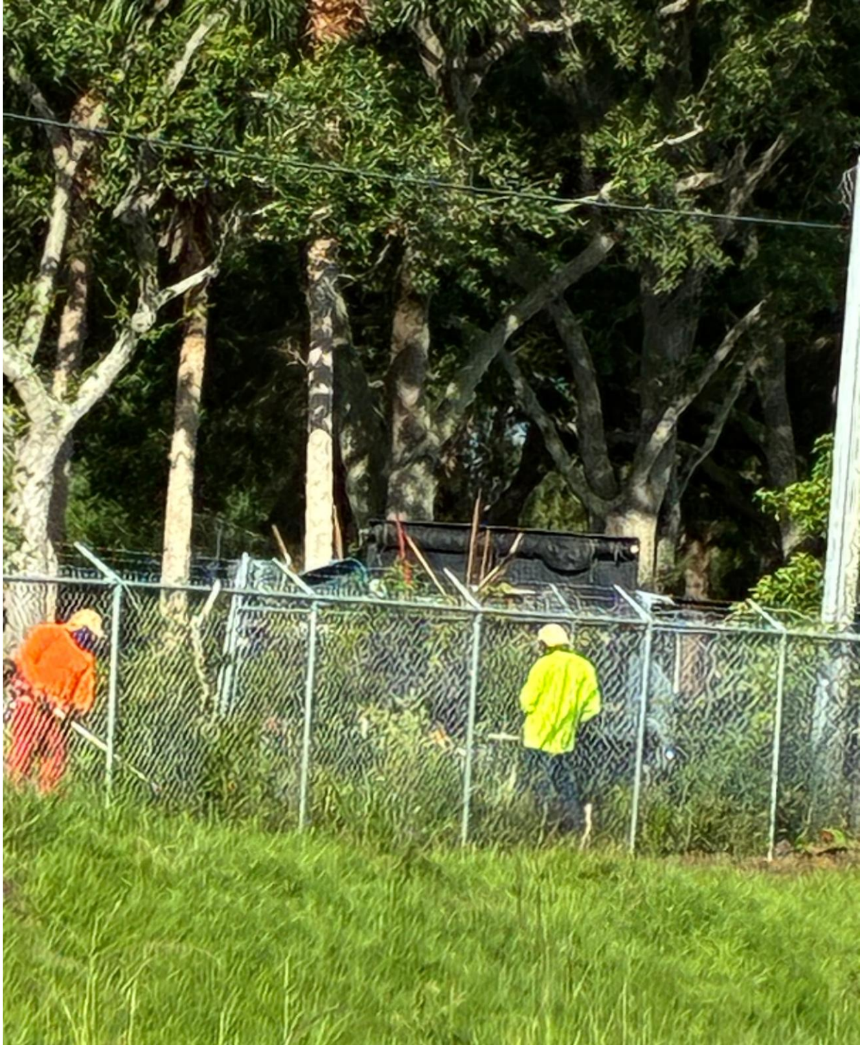
SOUTH CANAL- SEACREST IS CLEARING BRUSH ALONG THE FENCE LINE SO THAT BUDGET FENCE CAN WORK THIS WEEK.
