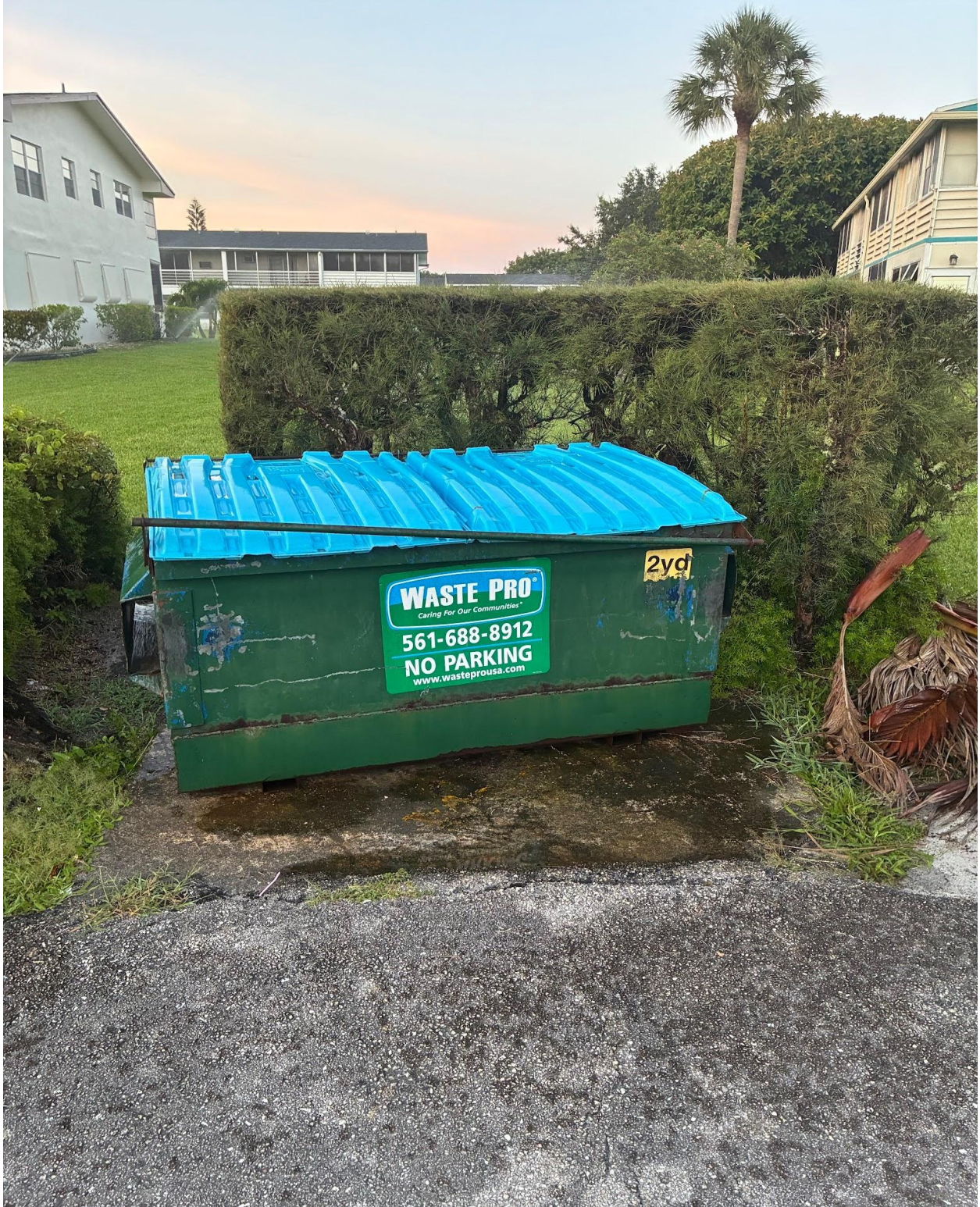
CAMDEN H/I- DUMPSTER WITH BUSTED RACCOON BAR. A REQUEST FOR REPAIR WAS SENT TO WASTE PRO.
