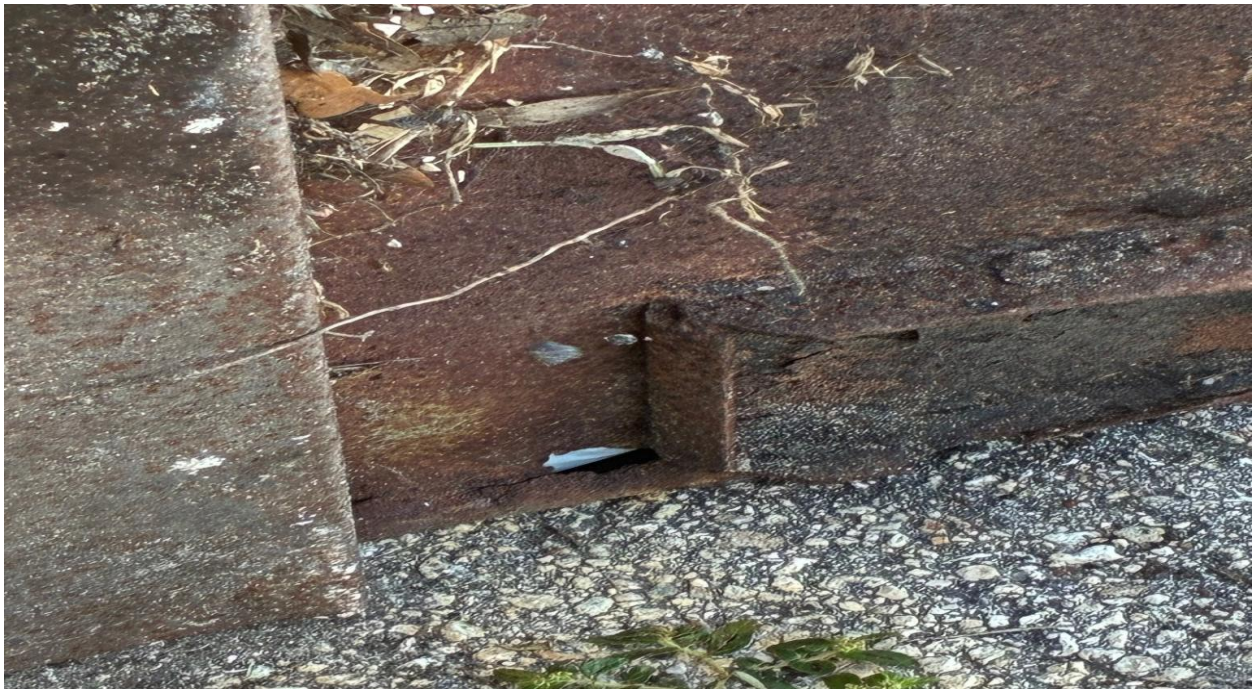
CHATHAM A- RUSTED OUT DUMPSTER. A REQUEST FOR REPLACEMENT WAS SENT TO WASTE PRO.
