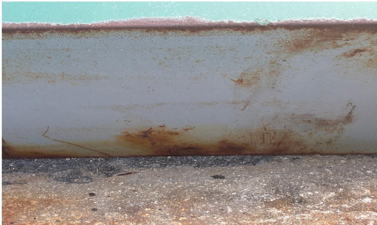
CHATHAM Q/R- RUSTED OUT DUMPSTER. A REQUEST FOR REPLACEMENT WAS SENT TO WASTE PRO.
