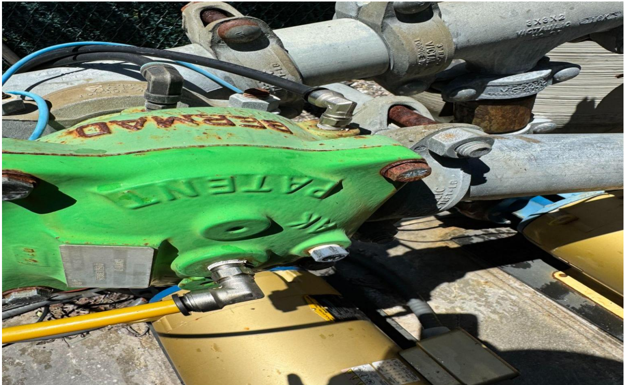
SOUTH DRIVE IRRIGATION PUMP STATION- ON 5/7, CHABOT IRRIGATION REPLACED PVC FITTINGS WITH BRASS FITTINGS, THIS IS PREVENTATIVE MAINTENANCE.
