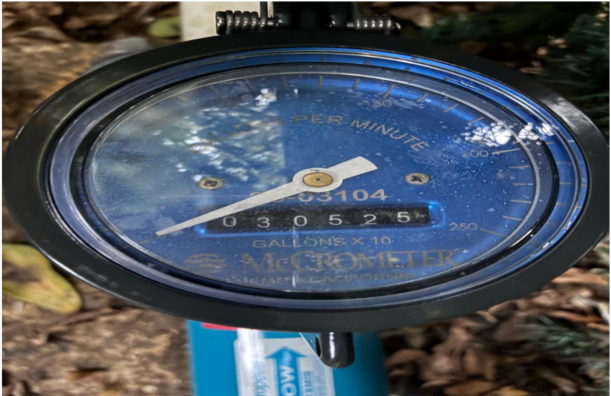
SHEFFIELD B/C- NEW IRRIGATION FLOWMETER INSTALLED BY CHABOT IRRIGATION.
