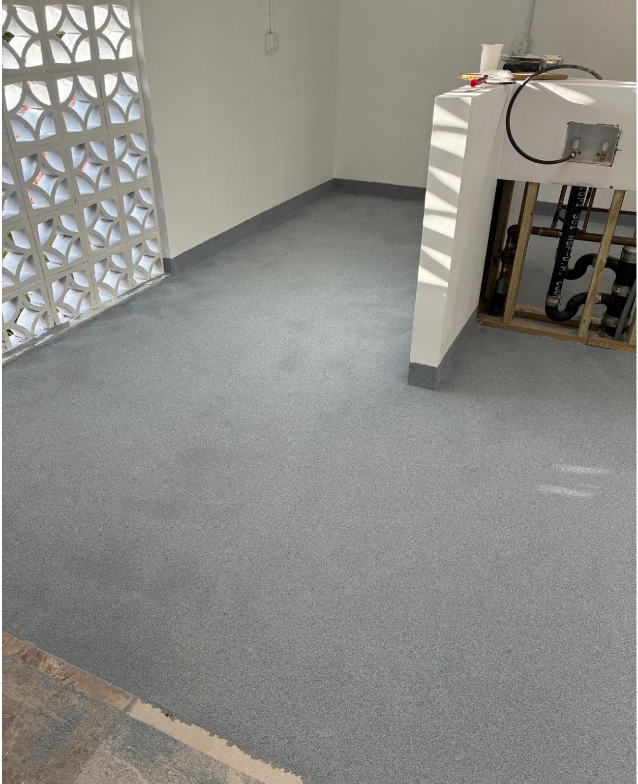
PLYMOUTH LAUNDRY- SECOND COAT FOR NEW EPOXY FLOOR WAS PUT DOWN LAST WEEK. FINAL SEALING COAT IS NEXT.
