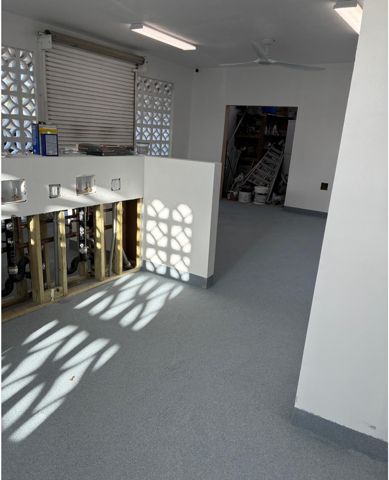
PLYMOUTH LAUNDRY- SECOND COAT FOR NEW EPOXY FLOOR WAS PUT DOWN LAST WEEK. FINAL SEALING COAT IS NEXT.
