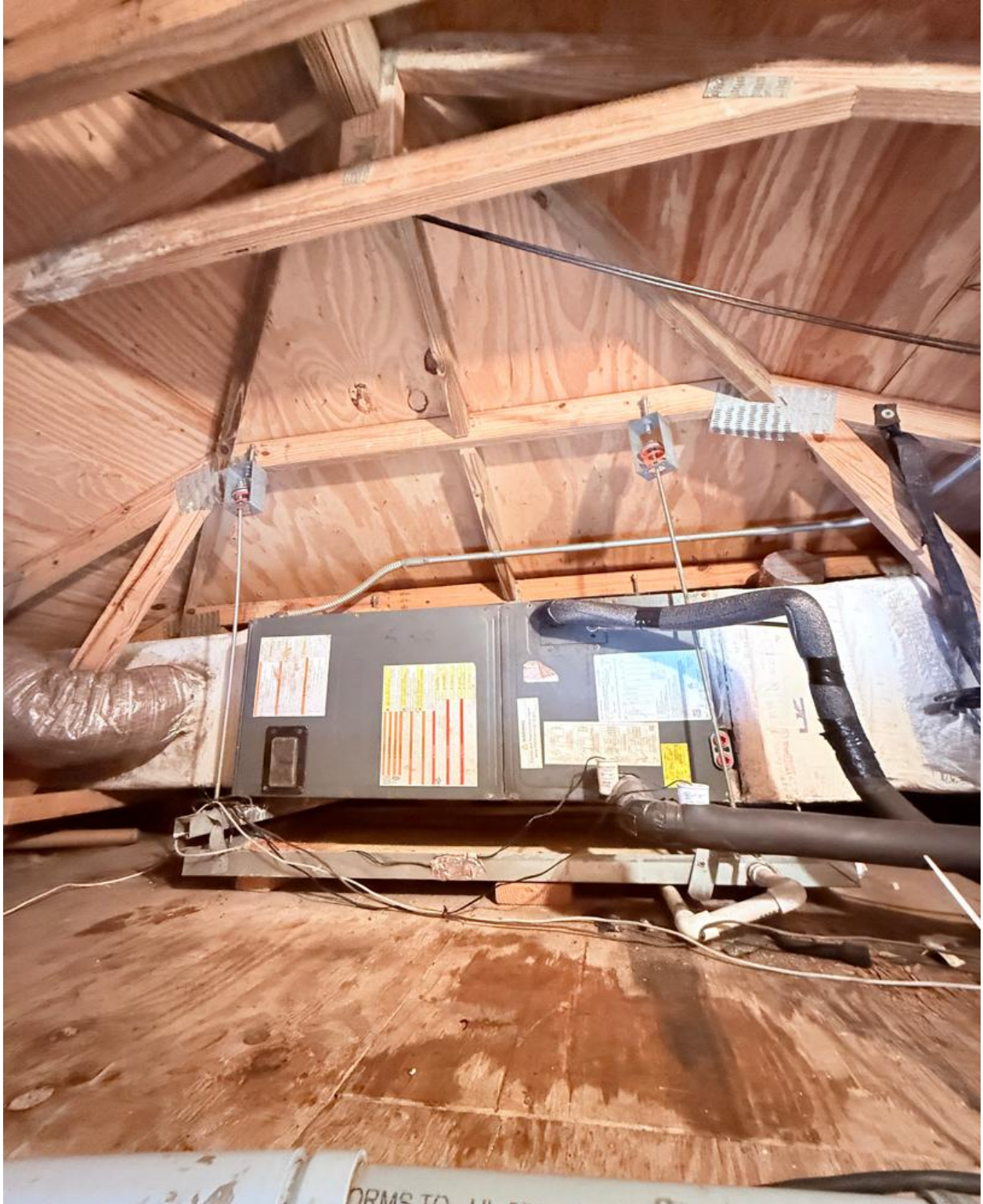
OKEECHOBEE BOULEVARD- AIR HANDLER UNITS IN GUARDHOUSE ATTICS WERE SERVICED. NICE TO SEE THAT THE ATTICS ARE CLEAN AND DRY.
