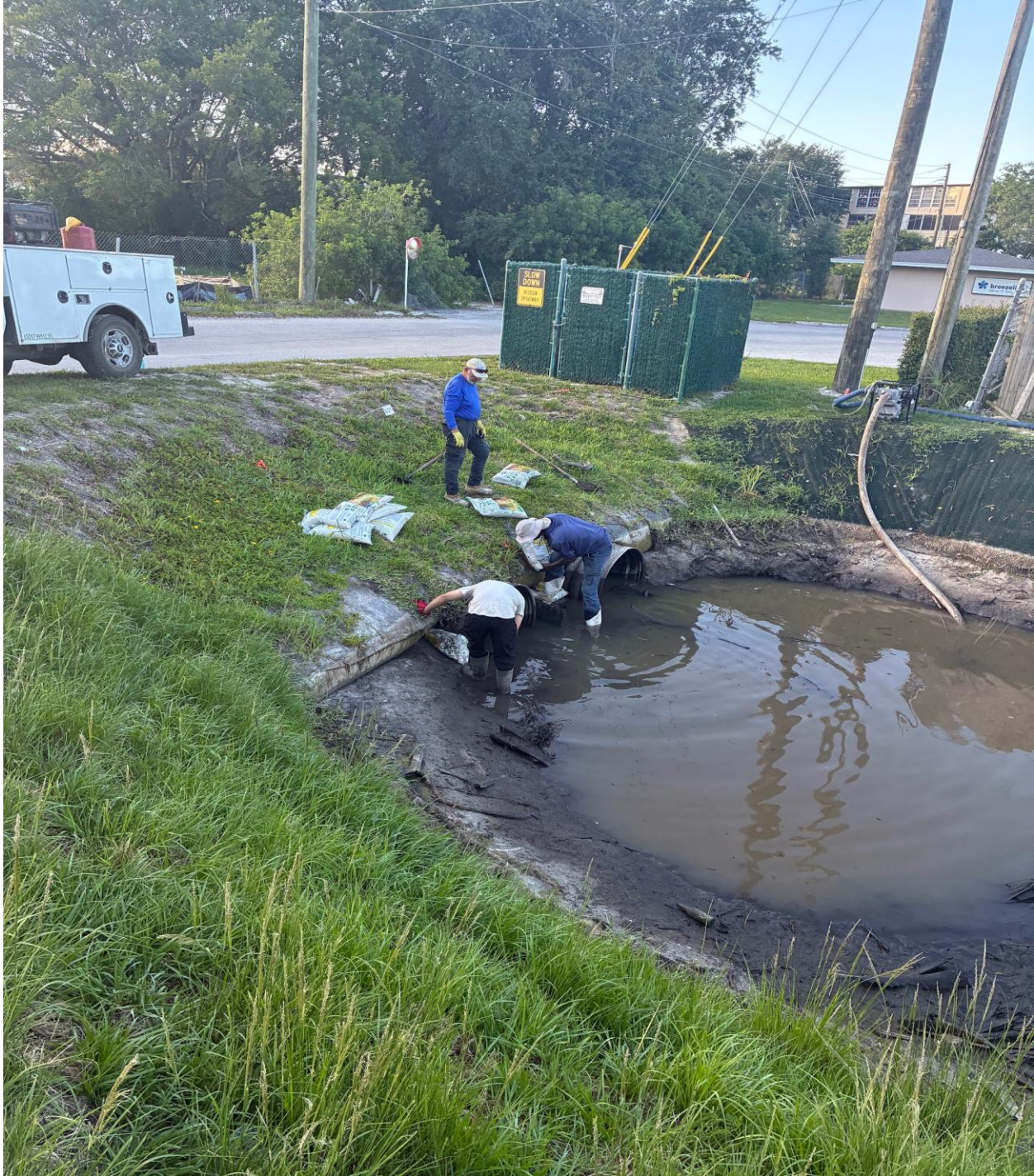
FAIRWAY STREET- THESE ARE THE TWO UNDERGROUND PIPES THAT CONNECT THE REFLECTION BAY LAKE TO OUR SOUTH CANAL. THESE MEN WERE STABILIZING THE PIPES WITH SANDBAGS ON 5/16.
