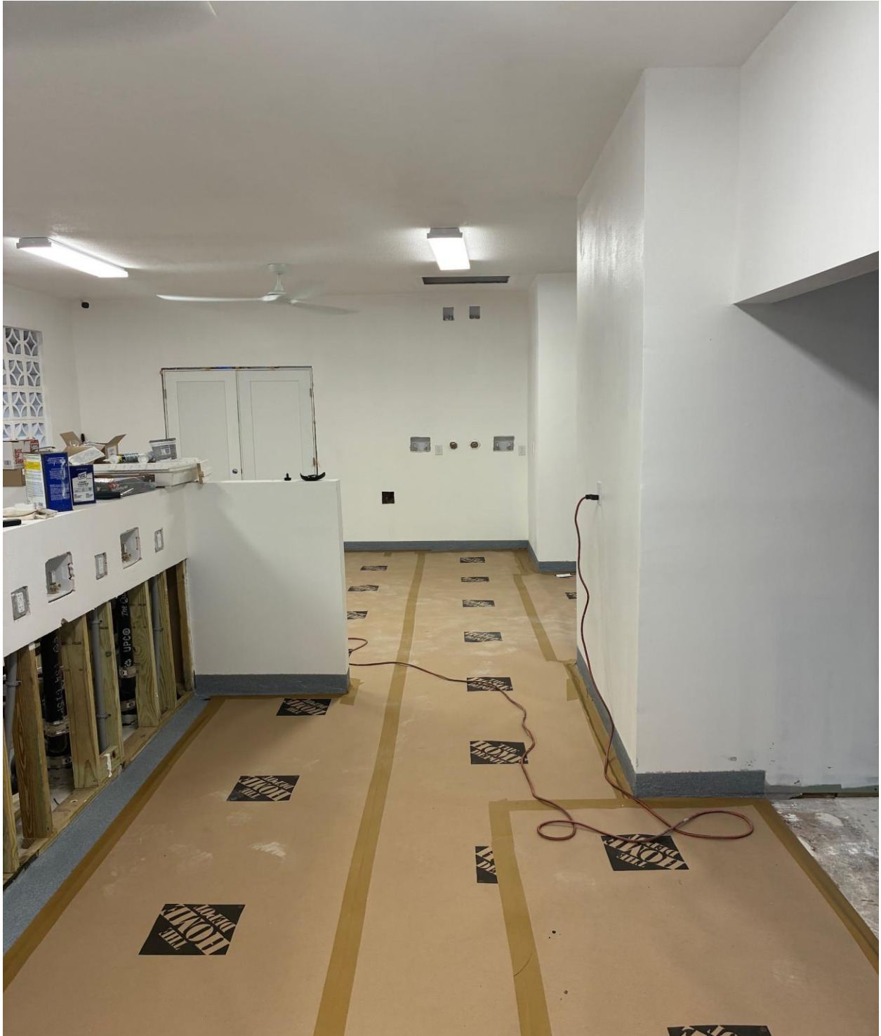
PLYMOUTH LAUNDRY- FINISH CARPENTRY WORK CONTINUES. OUR NEW EPOXY FLOOR WAS COVERED WITH CARDBOARD TO KEEP IT FROM BEING SCUFFED.
