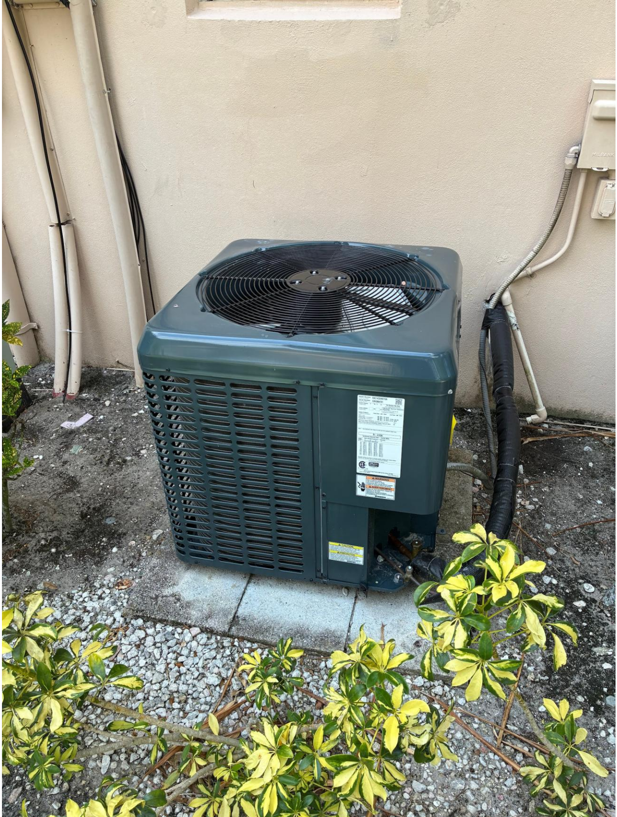
4 SALISBURY A- NEW HVAC INSTALLATION, NO PERMIT.
