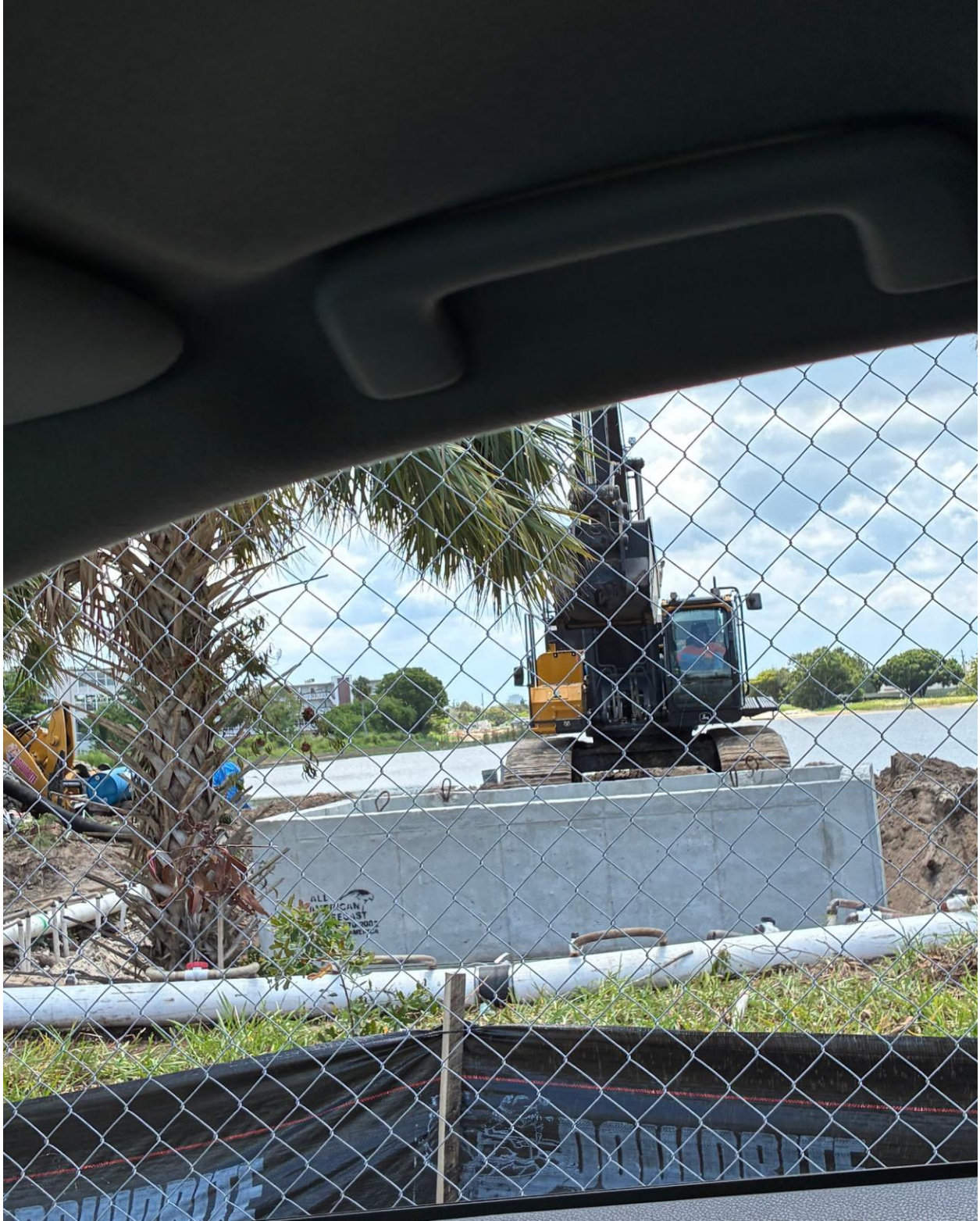
FAIRWAY STREET- THIS IS WHERE THE REFLECTION BAY LAKE CONNECTS WITH CV SOUTH CANAL, THROUGH TWO 54 INCH UNDERGROUND PIPES RUNNING UNDER FAIRWAY STREET.
