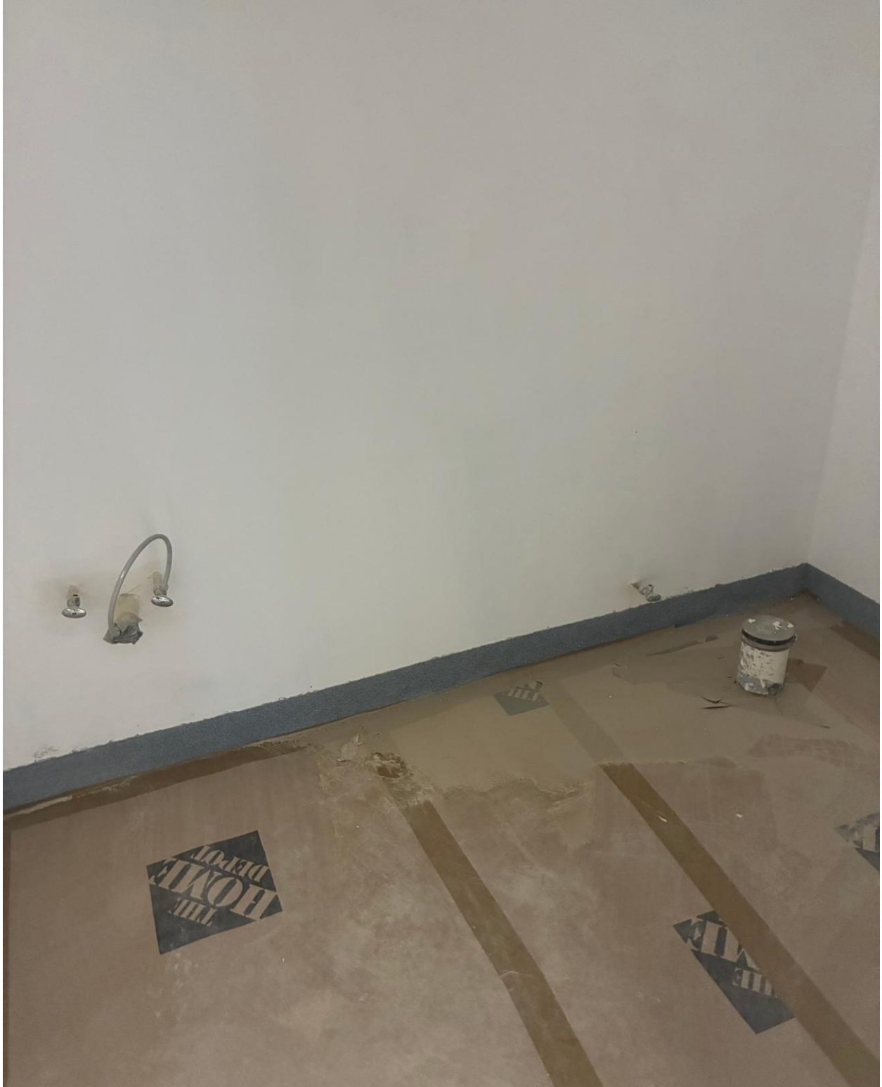
PLYMOUTH LAUNDRY- OUR NEW ADA COMPLIANT REST ROOM IS READY FOR SINK AND TOILET INSTALLATION.
