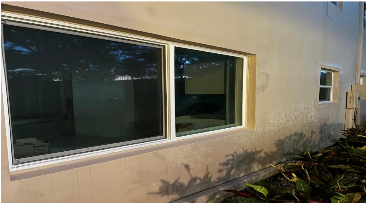
4 SALISBURY A- NEW WINDOWS AND DOOR INSTALLED, NO PERMITS APPLIED FOR OR ISSUED. NO PERMIT IN FRONT WINDOW.
