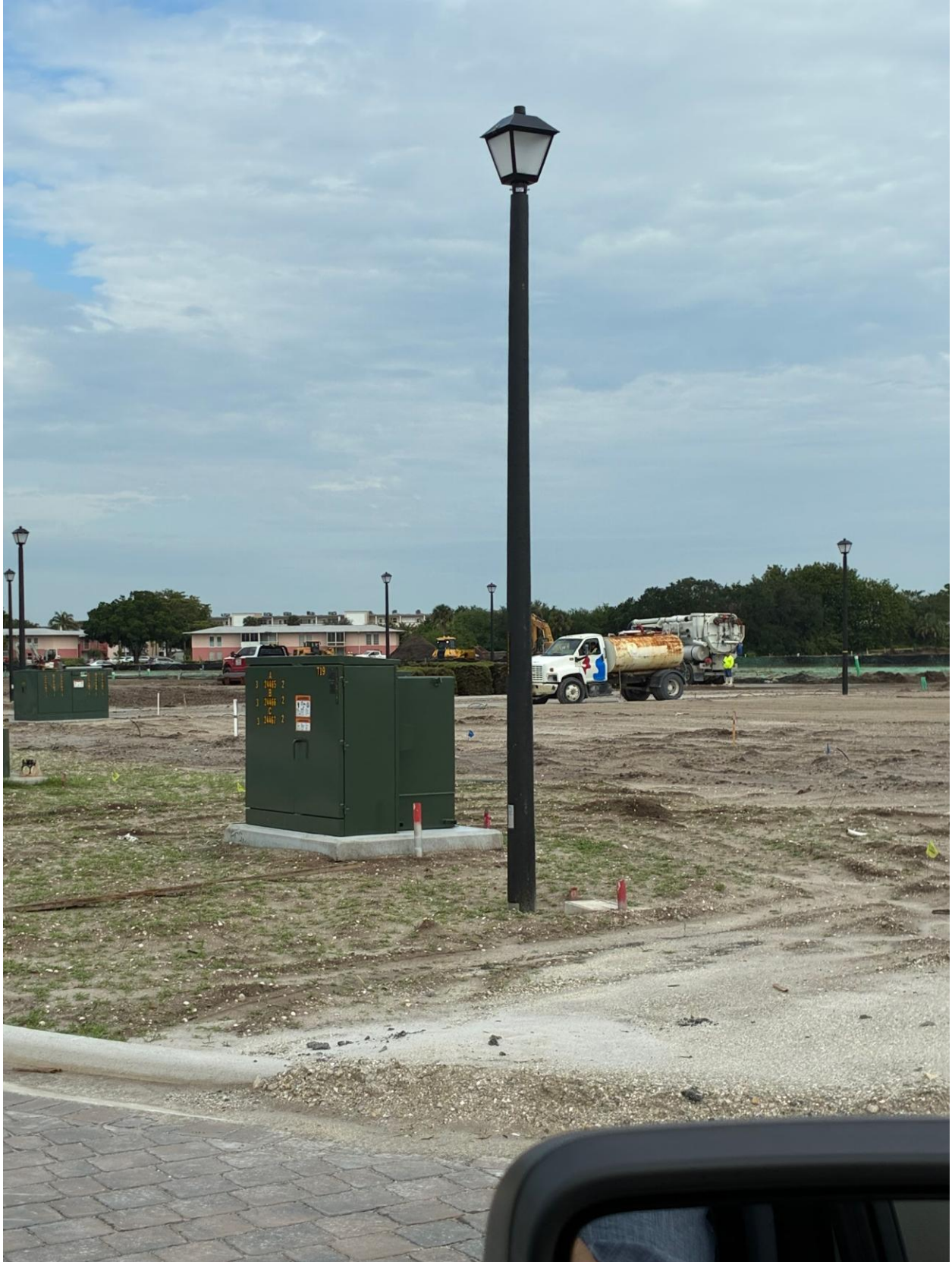
REFLECTION BAY- ELECTRIC TRANSFORMERS, STREETLIGHTS.
