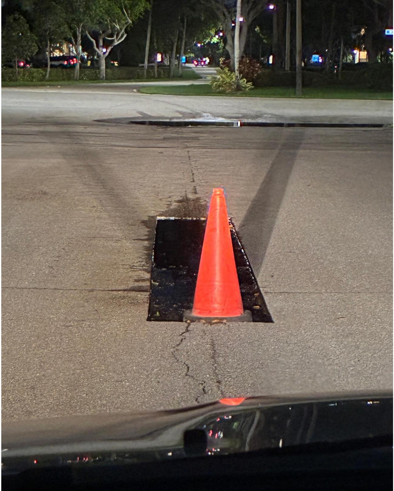
CAMDEN/WINDSOR SECTION- DETERIORATED SECTION OF ROAD SAW CUT AND COMPACTED, READY FOR NEW ASPHALT.
