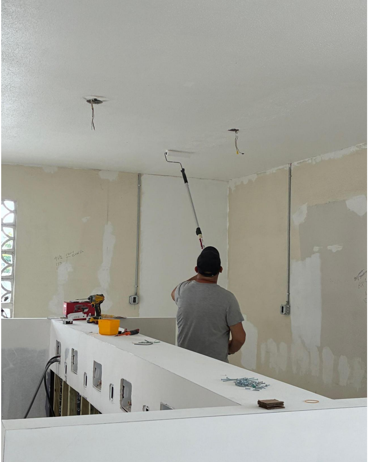
PLYMOUTH LAUNDRY- LAST WEEK, WALLS AND CEILINGS WERE PAINTED, FLOORS WERE PREPPED FOR EPOXY COATING.
