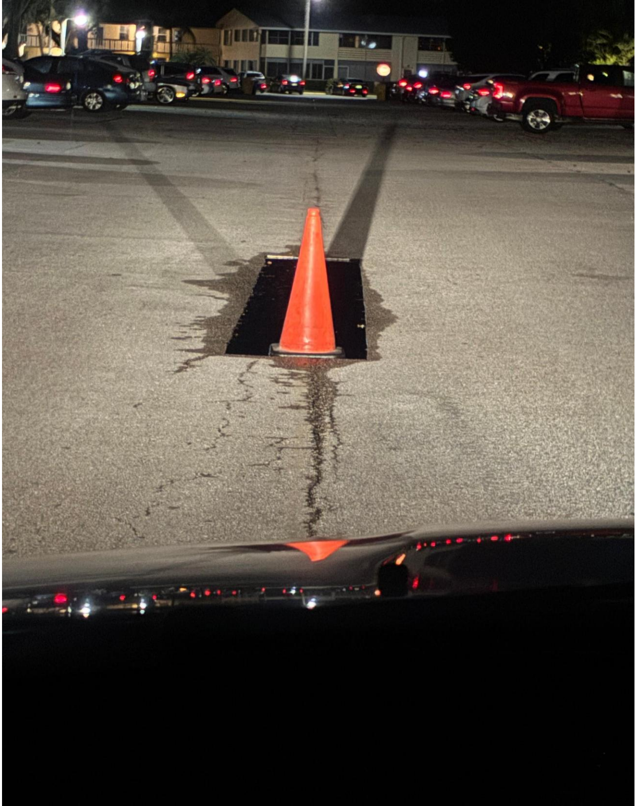
CAMDEN/WINDSOR SECTION- DETERIORATED SECTION OF ROAD SAW CUT AND COMPACTED, READY FOR NEW ASPHALT.
