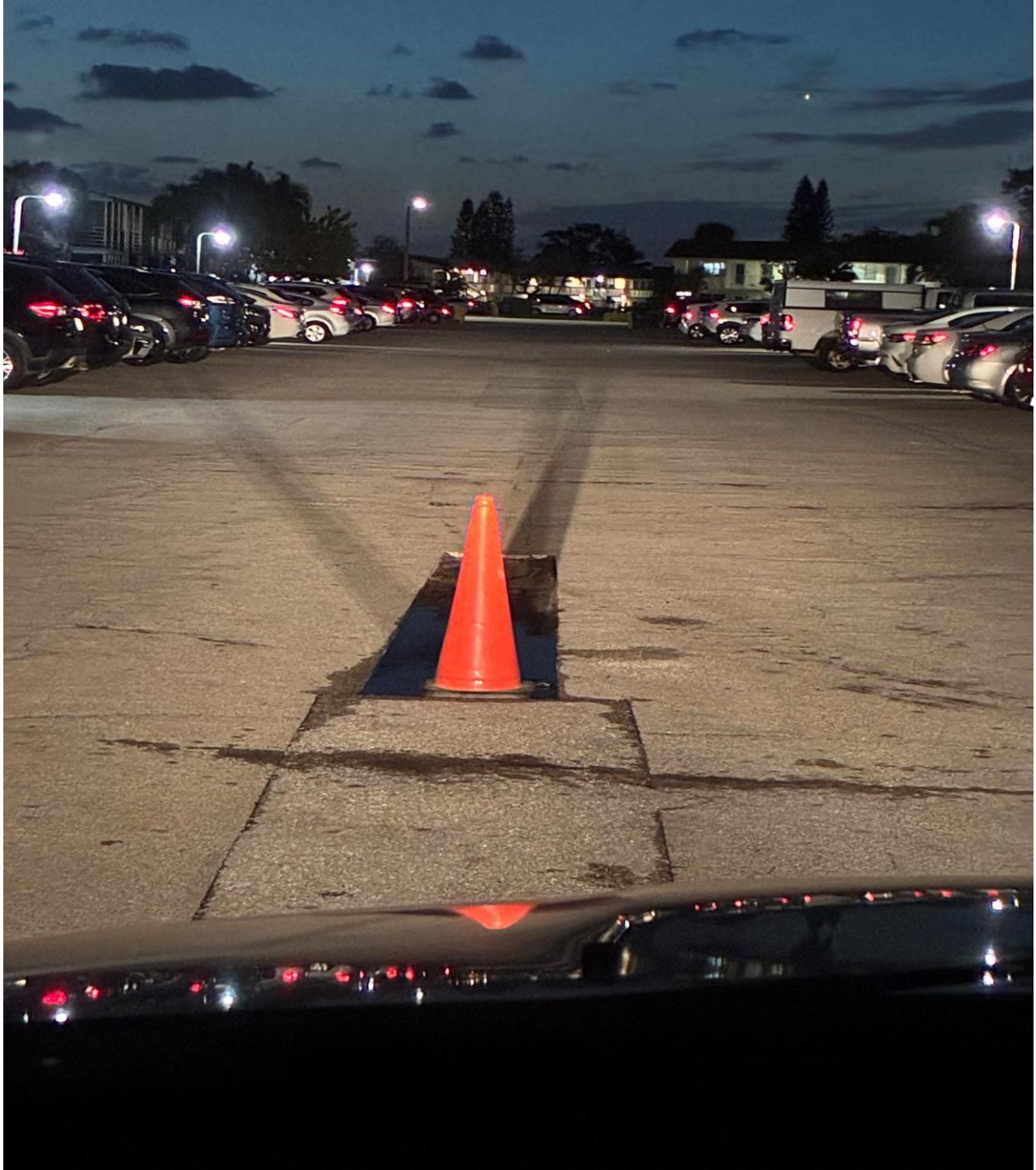
CAMDEN/WINDSOR SECTION- DETERIORATED SECTION OF ROAD SAW CUT AND COMPACTED, READY FOR NEW ASPHALT.
