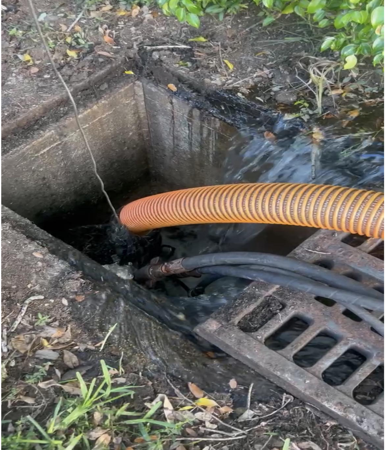
CV MEDICAL BUILDING- ANCHOR MARINE CLEARED THIS DRAIN ON 4/23.
