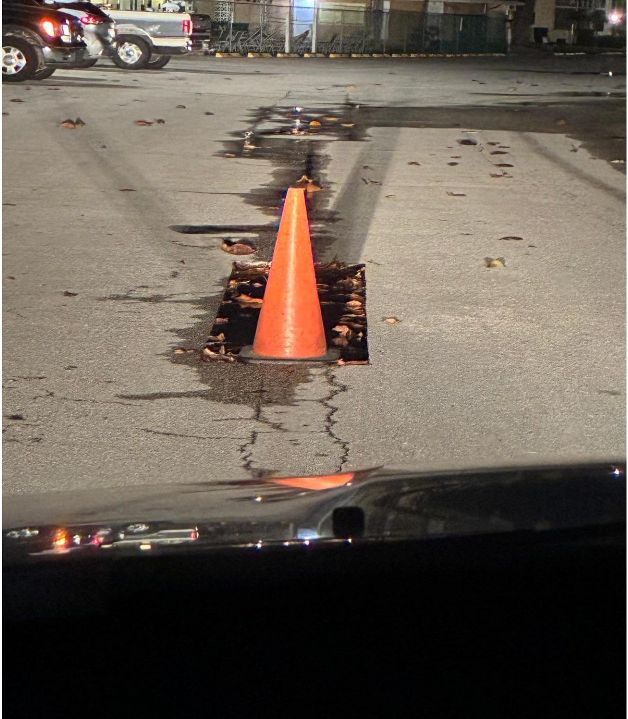
CAMDEN/WINDSOR SECTION- DETERIORATED SECTION OF ROAD SAW CUT AND COMPACTED, READY FOR NEW ASPHALT.
