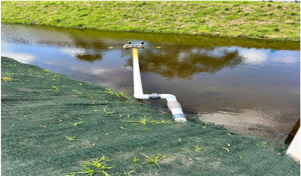
SOUTH CANAL- ON 4/23, CHABOT IRRIGATION RE-PLUMBED THE INTAKE PIPE FOR THE SOUTHAMPTON IRRIGATION PUMP STATION.
