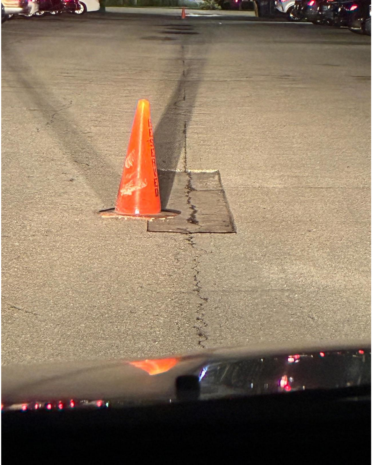
CAMDEN/WINDSOR SECTION- DETERIORATED SECTION OF ROAD SAW CUT AND COMPACTED, READY FOR NEW ASPHALT.
