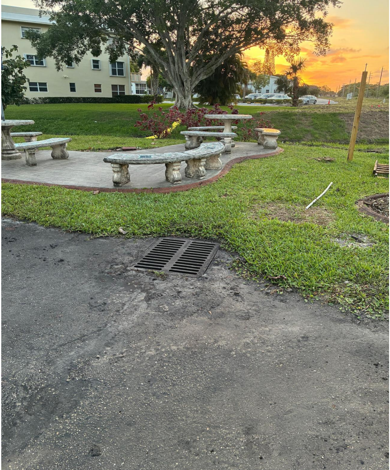
WELLINGTON M- THIS STORM DRAIN CATCH BASIN, WHICH WAS CLOGGED, WAS CLEARED BY SHENANDOAH CONSTRUCTION ON 3/20.
