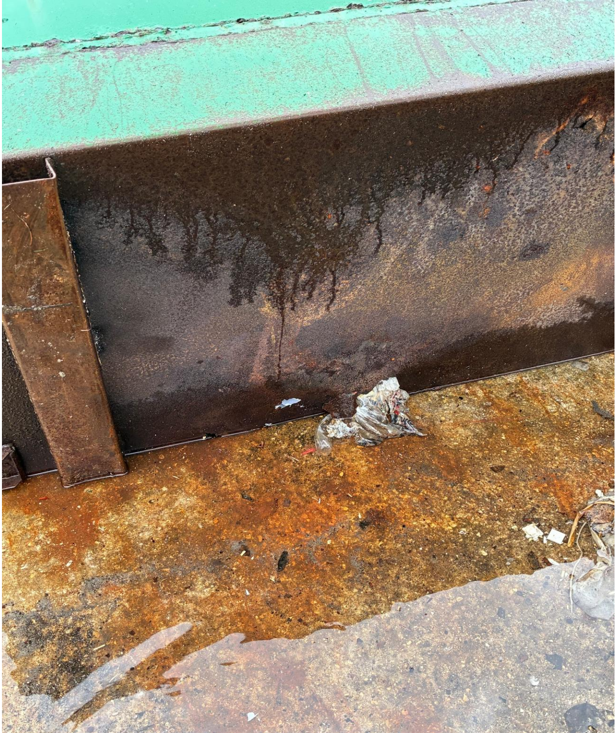
NORWICH I/N- HOLEY DUMPSTER. A REQUEST FOR REPLACEMENT WAS SENT TO WASTE PRO.
