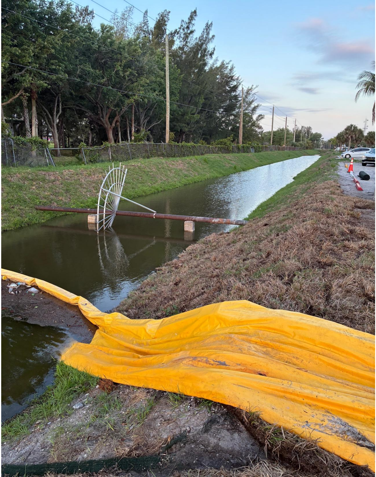
SOUTH CANAL- THE WASHED-OUT BANK NEAR WELLINGTON M WAS REPAIRED ON 3/30.
