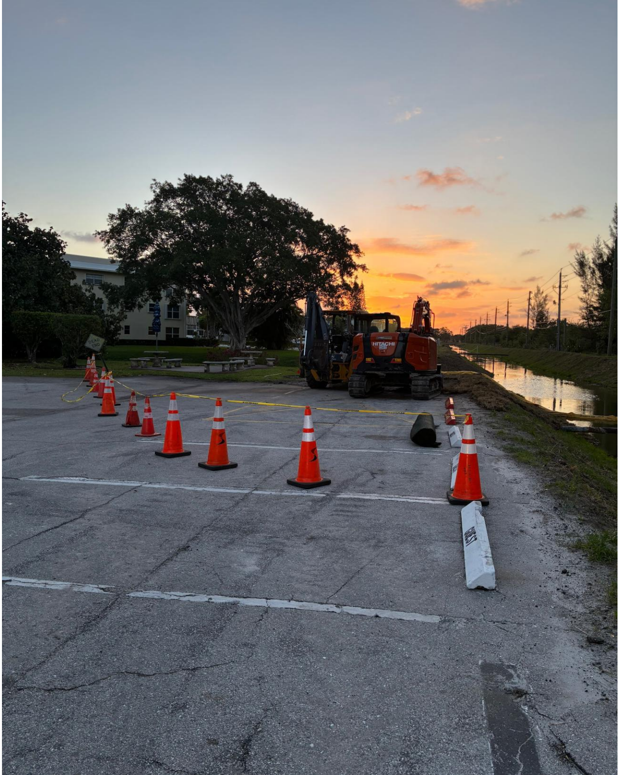
WELLINGTON M- THE CANAL BANK WASHOUT AREA WAS CORDONED OFF BY ST. MORITZ SECURITY ON 3/29.
