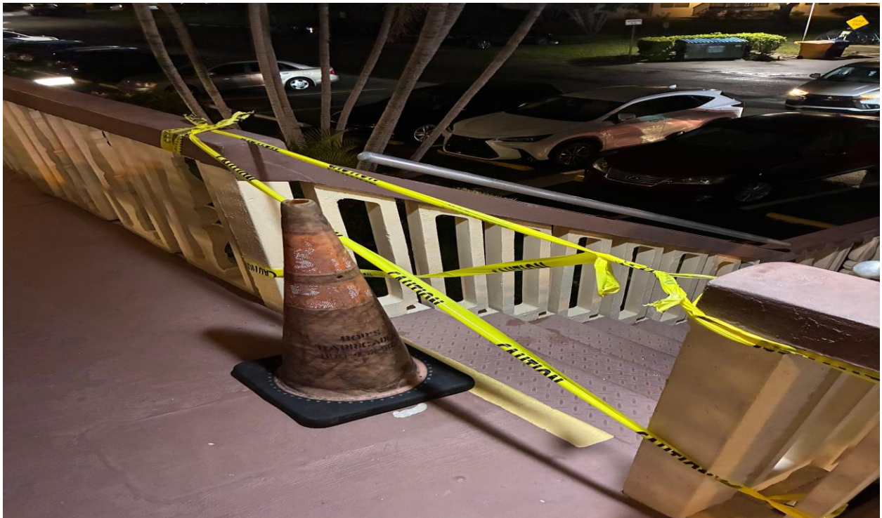
NORTHAMPTON M- THE DAMAGED STAIRCASE WAS CLOSED OFF TOP AND BOTTOM BY ST. MORITZ SECURITY.
