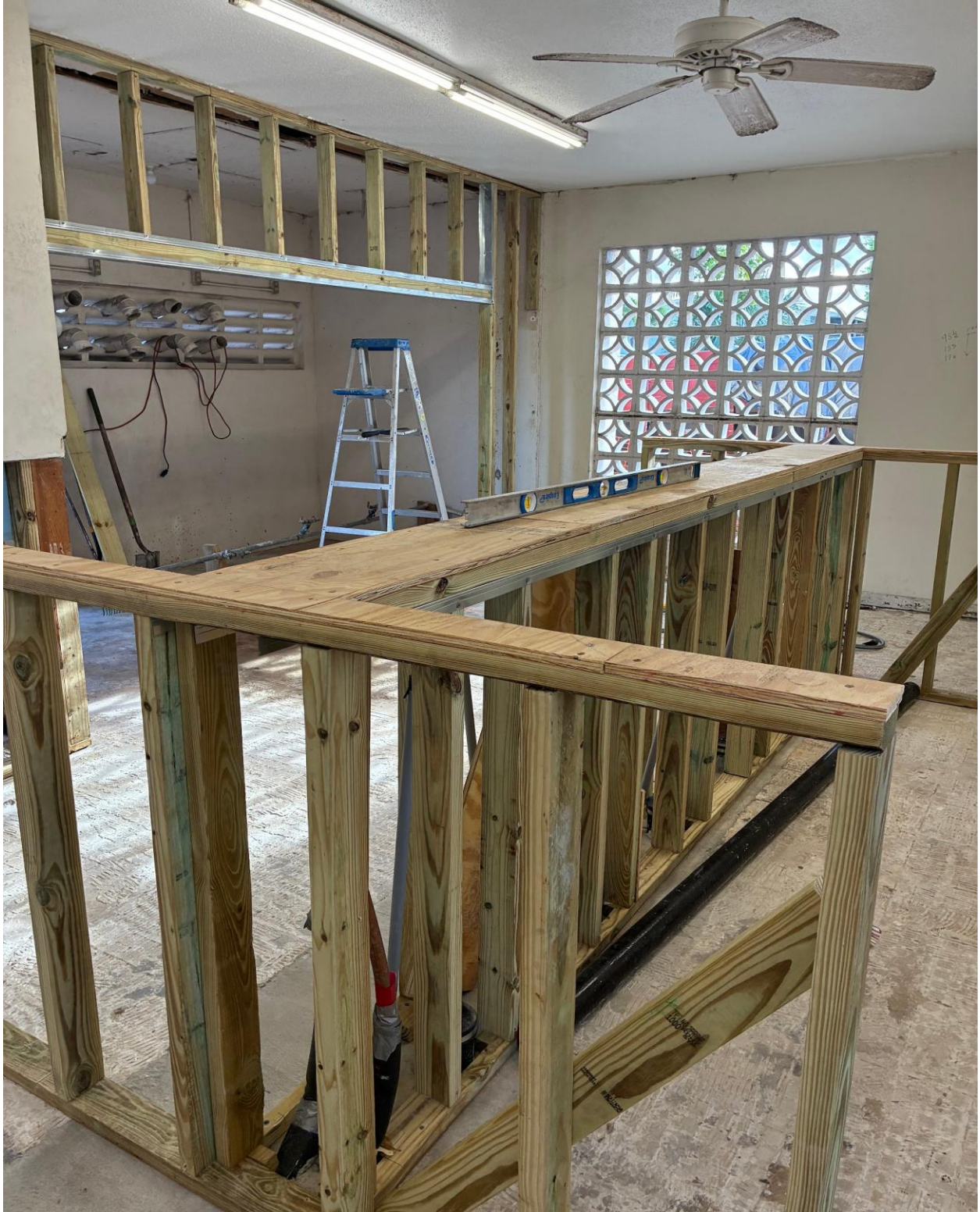
PLYMOUTH LAUNDRY- THIS FRAMING IS FOR A LOW WALL THAT WILL SURROUND THE WASHERS.
