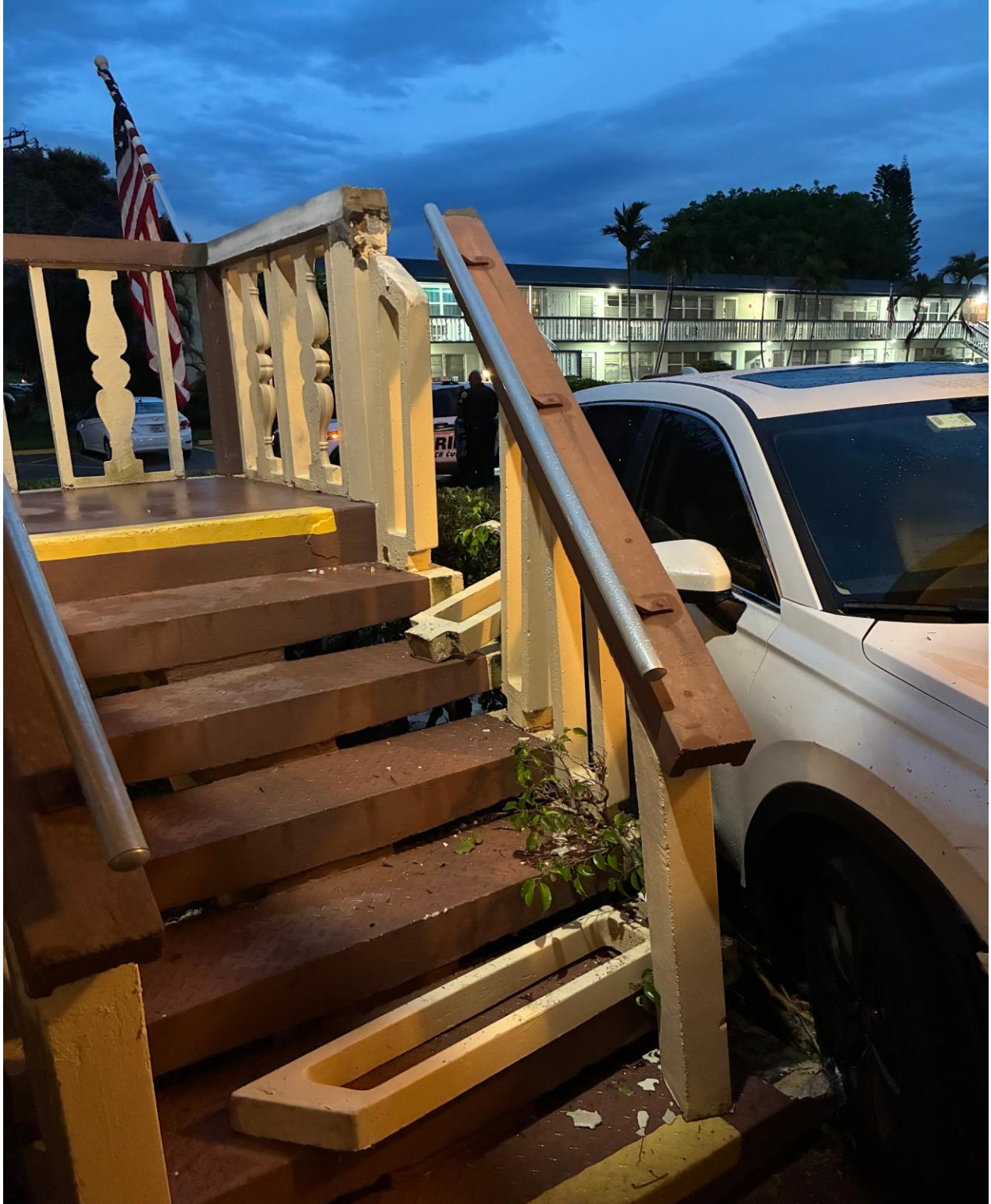
NORTHAMPTON M- THERE WAS MINOR DAMAGE TO THE BUILDING'S SOUTH STAIRCASE.
