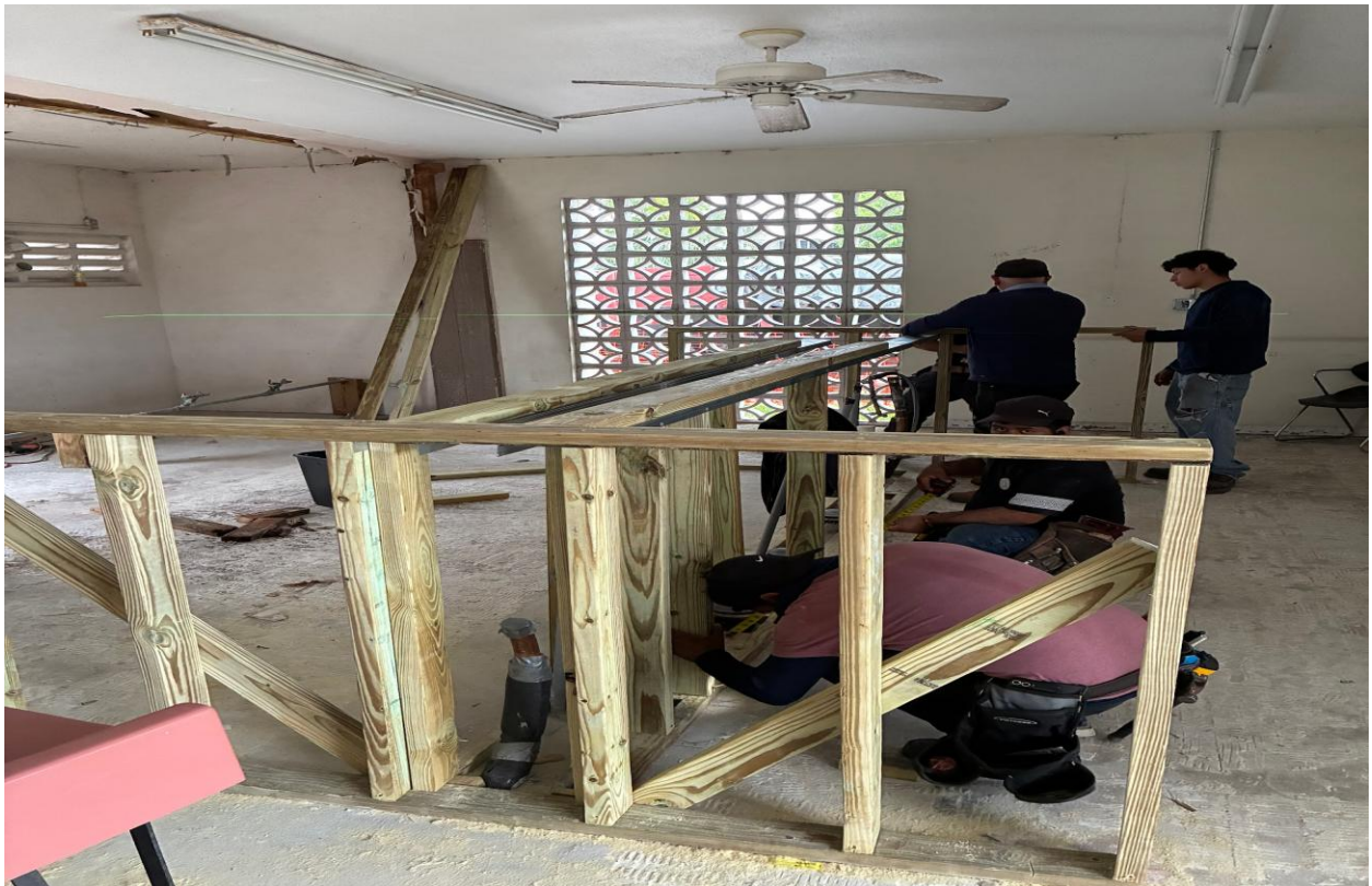
PLYMOUTH LAUNDRY- THIS FRAMING IS FOR A LOW WALL THAT WILL SURROUND THE WASHERS.
