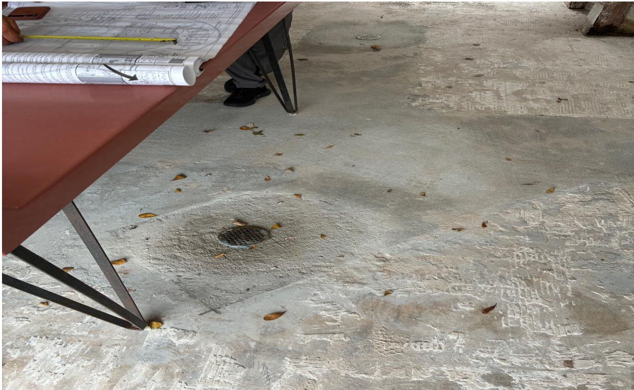
PLYMOUTH LAUNDRY- THESE NEW FLOOR DRAINS ARE CONNECTED TO THE NEW SEWER LINES. THIS WILL HELP WITH WASHER OVERFLOWS AND REDUCE SLIP HAZARDS.
