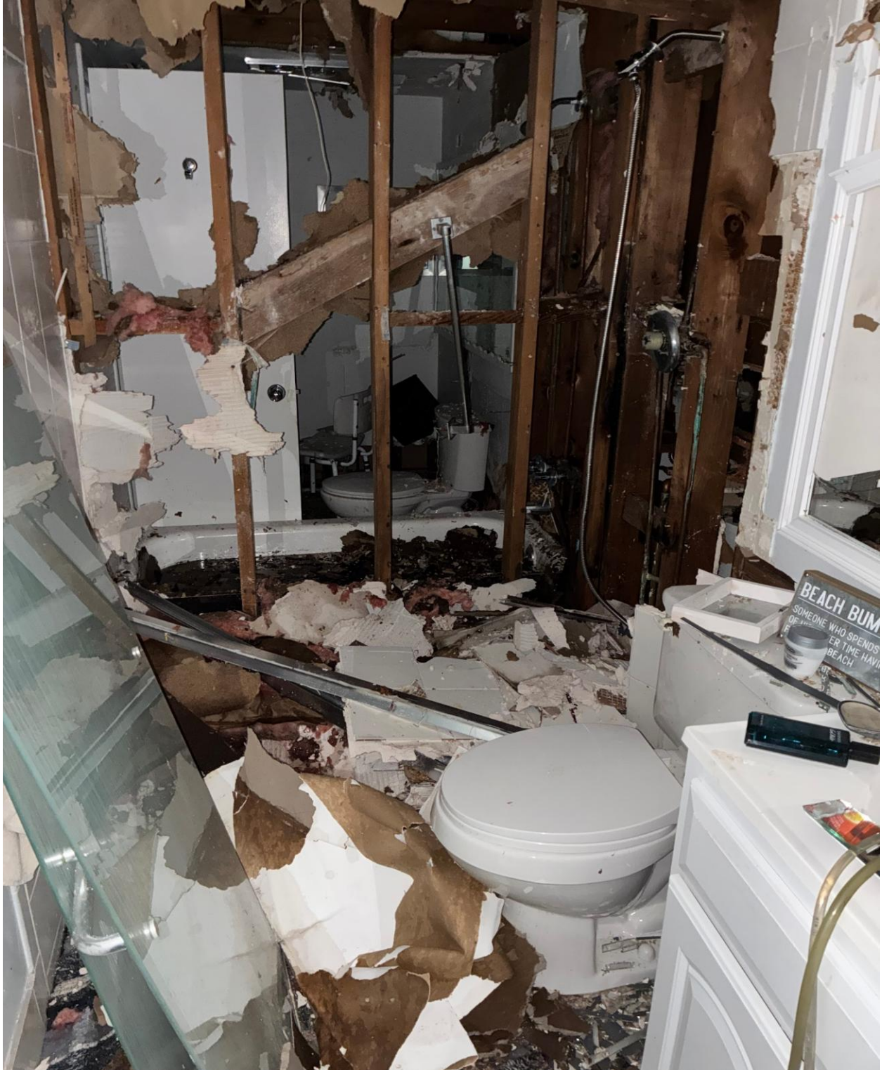
WALTHAM A- TWO UNITS WERE DESTROYED. SERVICEMASTER WORKED OVERNIGHT TO REMOVE STANDING WATER AND THEY ALSO INSTALLED DEHUMIDIFIERS TO LIMIT MOLD GROWTH.
