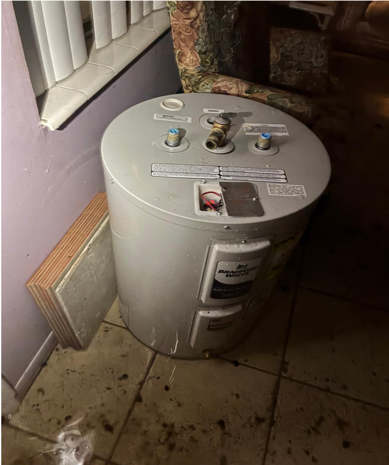
WALTHAM A- THIS HOT WATER HEATER WAS TO BE INSTALLED IN THE OTHER DESTROYED UNIT, BUT THE UNITS BURNED DOWN BEFORE IT COULD BE INSTALLED. ONLY LICENSED PLUMBERS SHOULD BE INSTALLING HOT WATER HEATERS.
