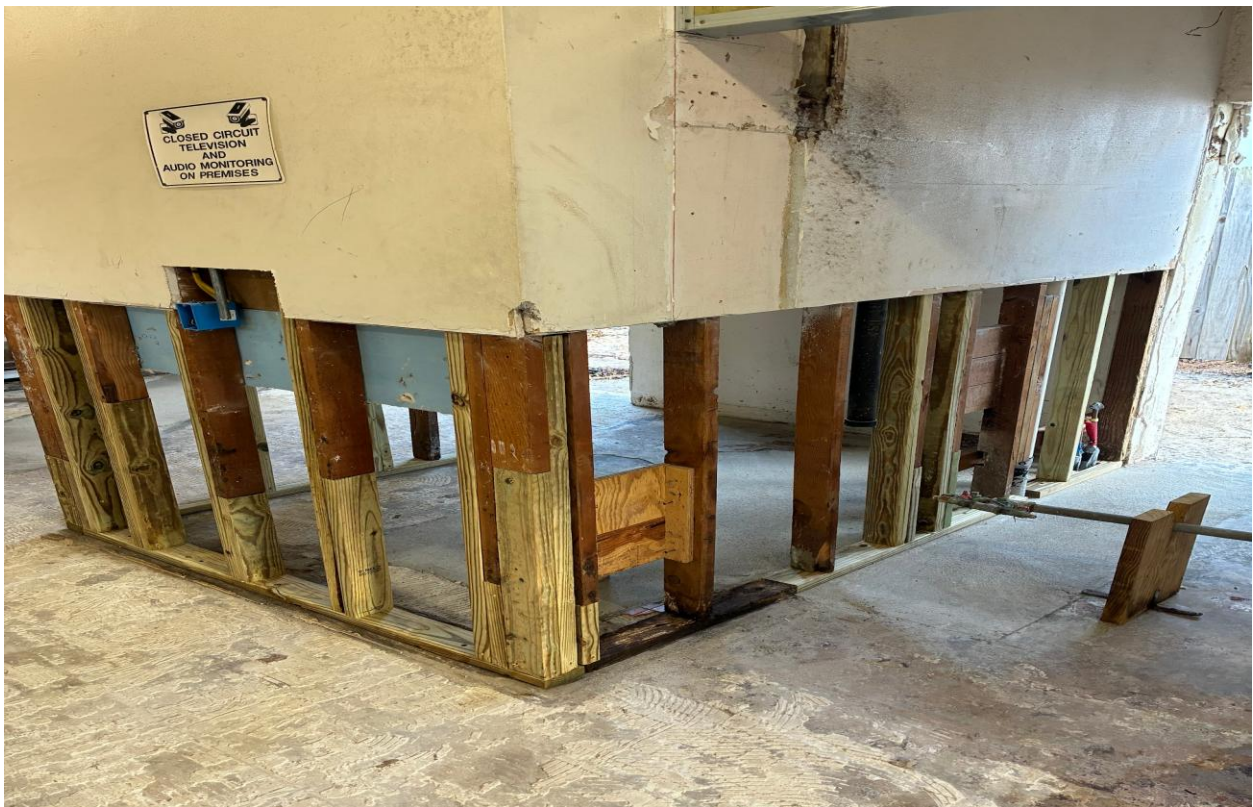
PLYMOUTH LAUNDRY- THE NEW ADA COMPLIANT REST ROOM IS BEING FRAMED OUT.
