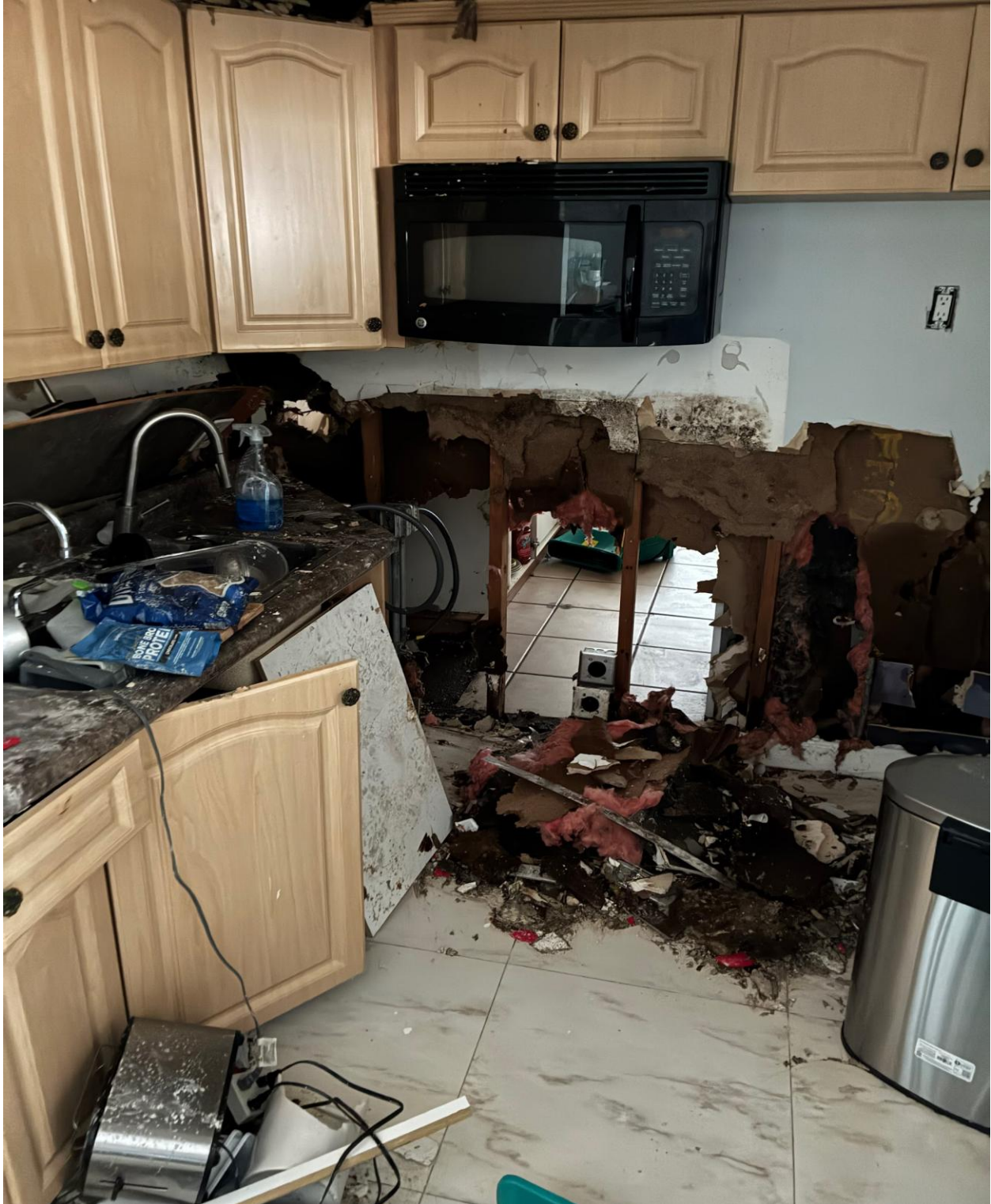
WALTHAM A- TWO UNITS WERE DESTROYED. NO INJURIES.
