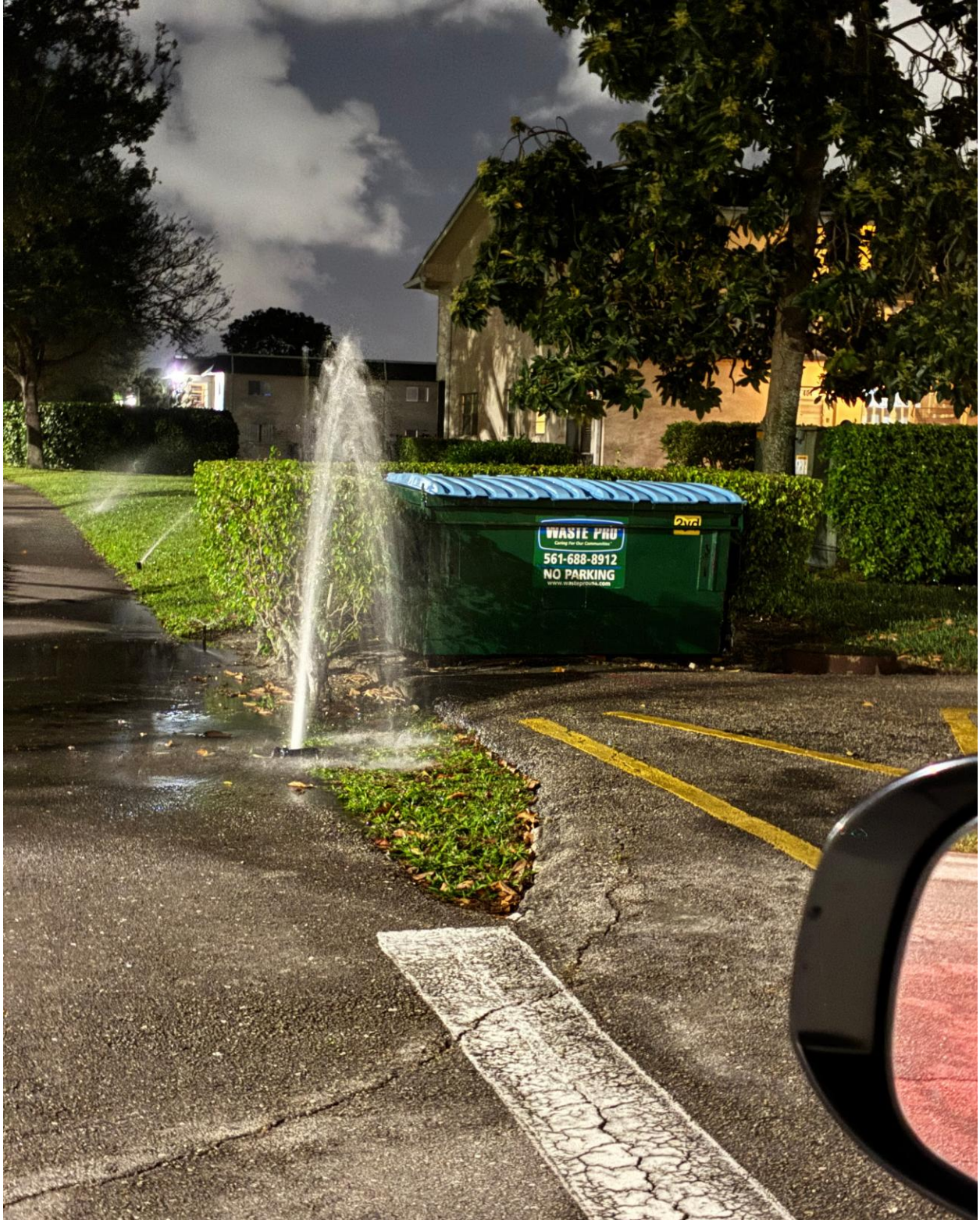
CHATHAM SECTION- IRRIGATION LEAK, DISCOVERED EARLY AM ON 3/7. SEACREST SERVICES HAS BEEN NOTIFIED AND WILL MAKE REPAIRS.
