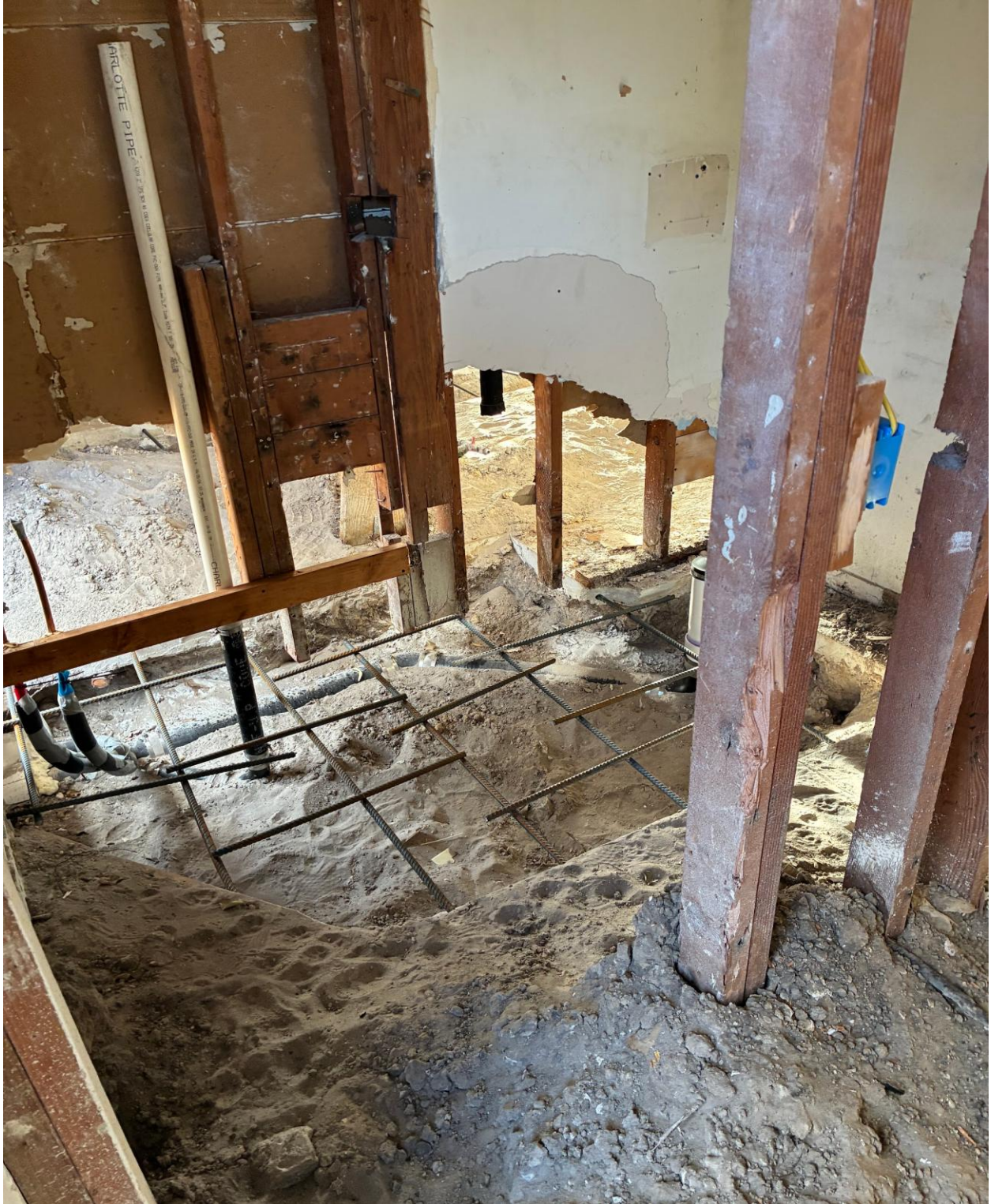
PLYMOUTH LAUNDRY- THIS AREA WILL BE THE NEW ADA COMPLIANT REST ROOM.
