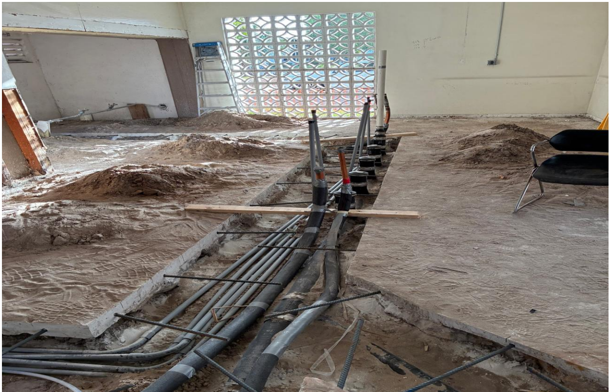
PLYMOUTH LAUNDRY- NEW REBAR INSTALLED, READY FOR INSPECTION, THEN BACKFILL AND NEW CONCRETE.
