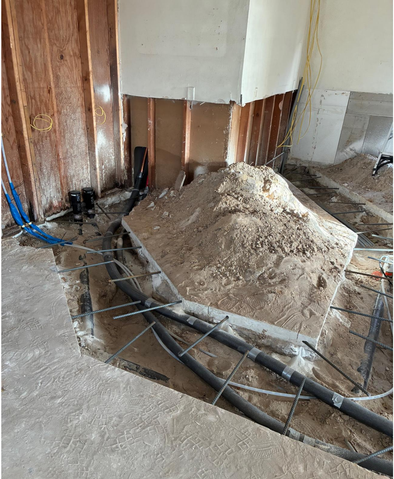
PLYMOUTH LAUNDRY- NEW REBAR INSTALLED, READY FOR INSPECTION, THEN BACKFILL AND NEW CONCRETE.
