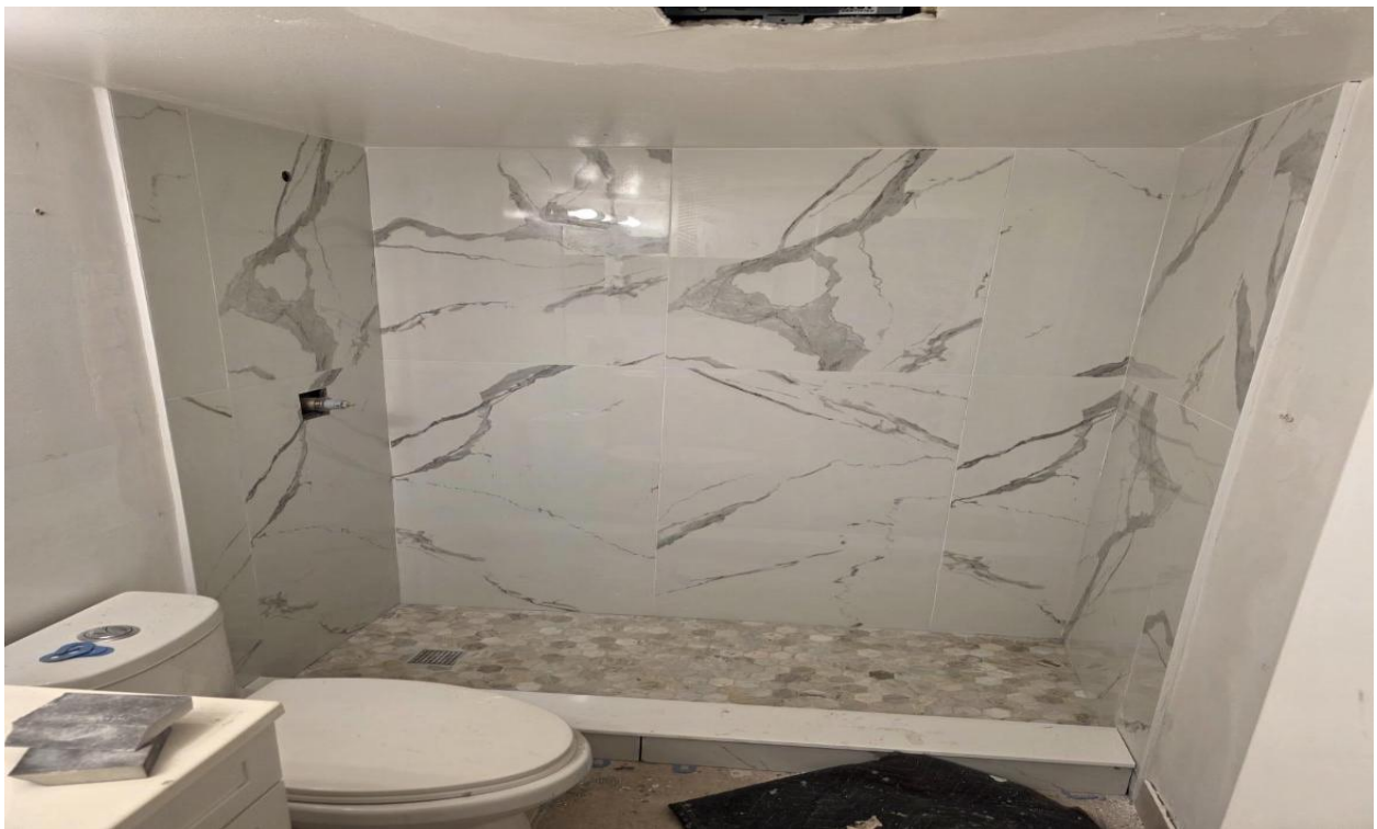
CAMDEN F- UNPERMITTED CONSTRUCTION WORK AT 123 CAMDEN F. REPORTED TO PZB CODE COMPLIANCE, #C-2026-03130021.
