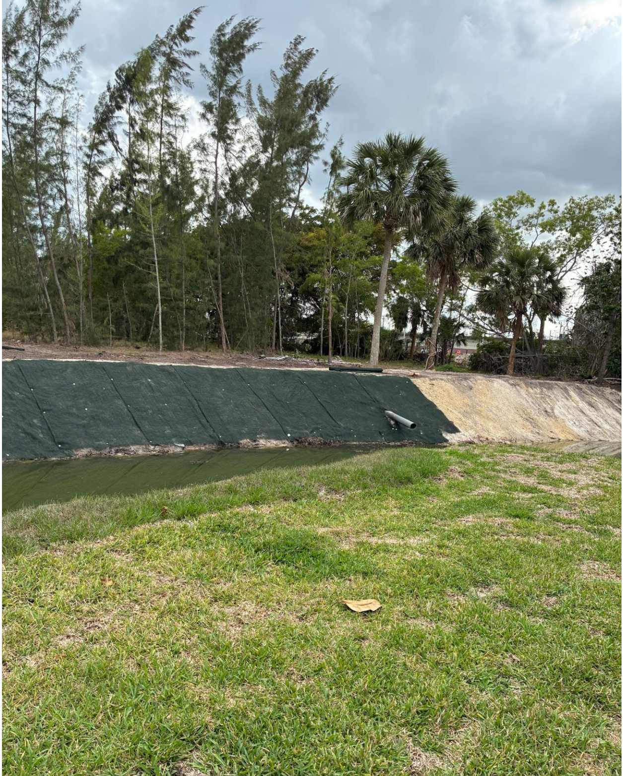
SOUTH CANAL- SHENANDOAH CONSTRUCTION IS WORKING ON THIS SECTION NEAR WINDSOR A.
