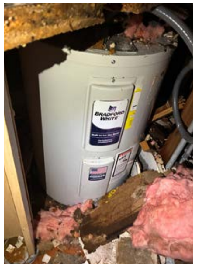
SEVERAL HOURS BEFORE THE FIRE, THIS HOT WATER HEATER WAS INSTALLED BY AN UNLICENSED HANDYMAN.
