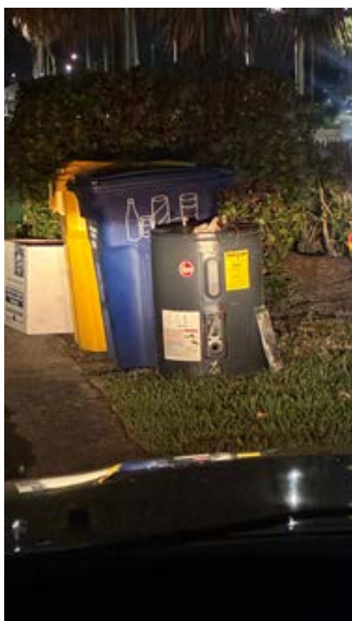
THIS IS THE OLD WATER HEATER, PUT OUT FOR THE TRASH.
