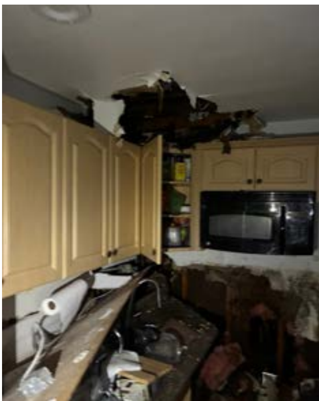
ANDOVER A, THE FIRE STARTED IN THIS KITCHEN, WHEN THE RESIDENT TURNED ON HIS STOVE TO COOK DINNER. AN UNPERMITTED HOT WATER HEATER HAD BEEN INSTALLED EARLIER THAT DAY.
