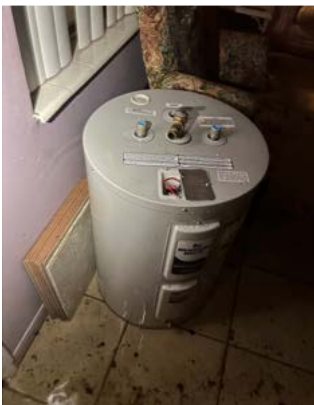
THIS UNINSTALLED HOT WATER HEATER WAS IN THE LIVING ROOM OF THE OTHER UNIT. THE BUILDING CAUGHT FIRE BEFORE IT COULD BE INSTALLED.
