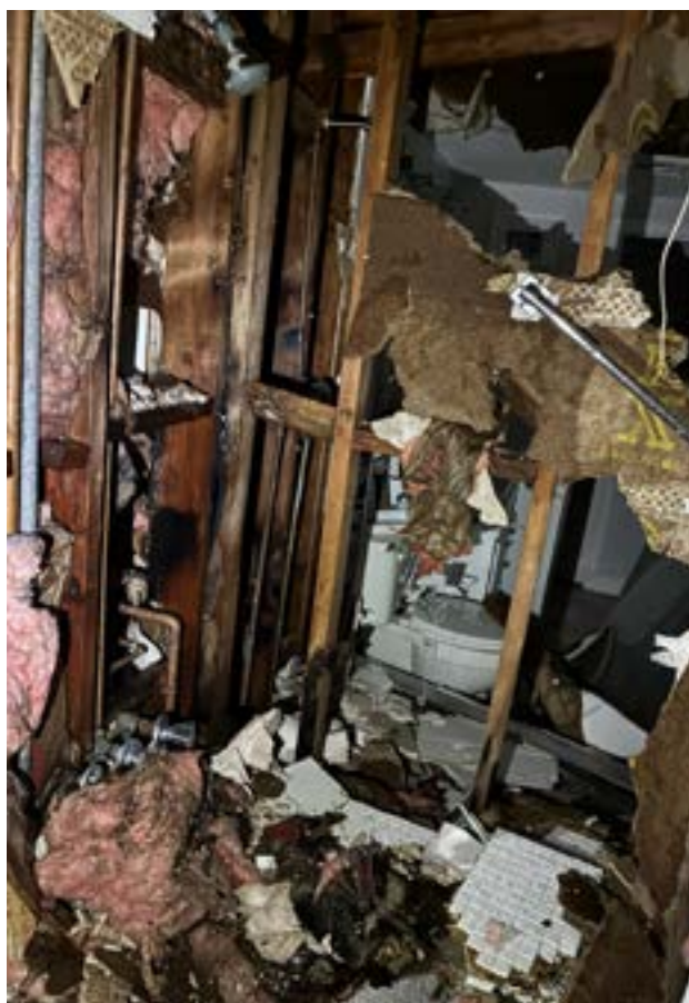
ANDOVER A- TWO UNITS, NEXT DOOR TO EACH OTHER, WERE DESTROYED.
