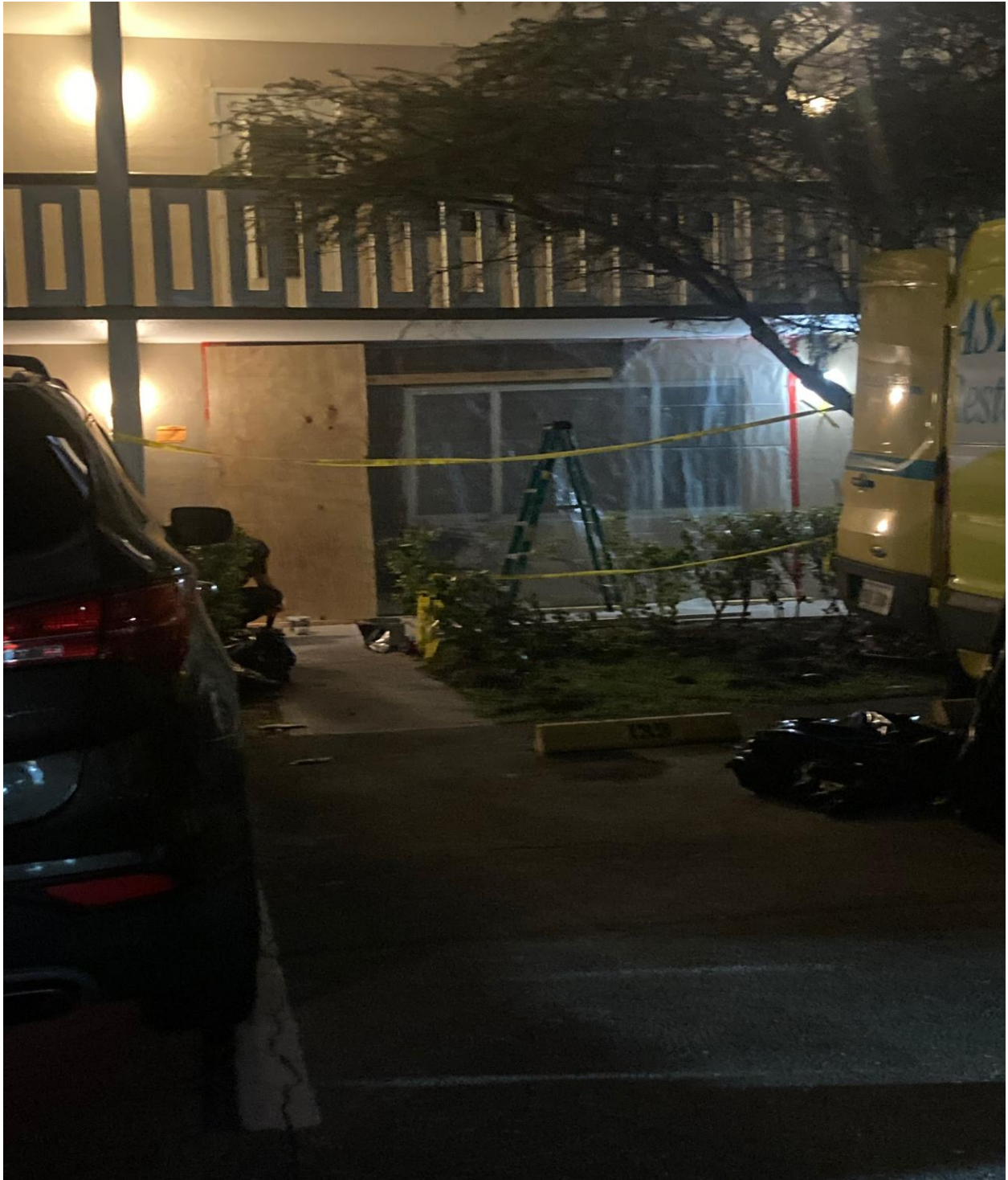
SERVICE MASTERS ARRIVED 8:00 PM TO BOARD UP THE FRONT OF THE UNIT.
