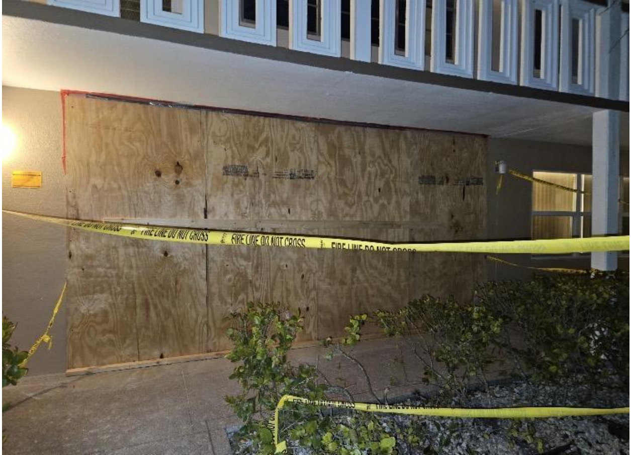
DOVER B- FRONT OF UNIT BOARDED UP 10:00 P.M. ON 2/7. PLASTIC SHEETING IN BACK OF THE PLYWOOD. THANKS SERVICE MASTERS.
