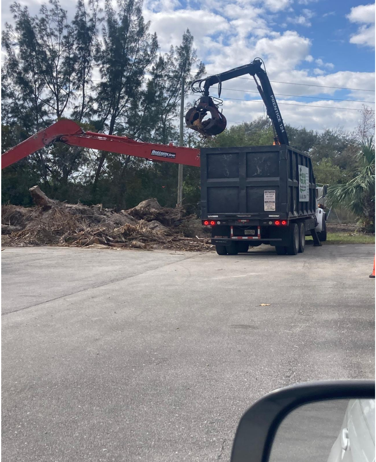
WELLINGTON E- CONSTRUCTION WORK AT SOUTH CANAL CONTINUES. LAST WEEK, GIANT PILES OF TREES, PALMS AND STUMPS WERE REMOVED FROM THE PROPERTY.
