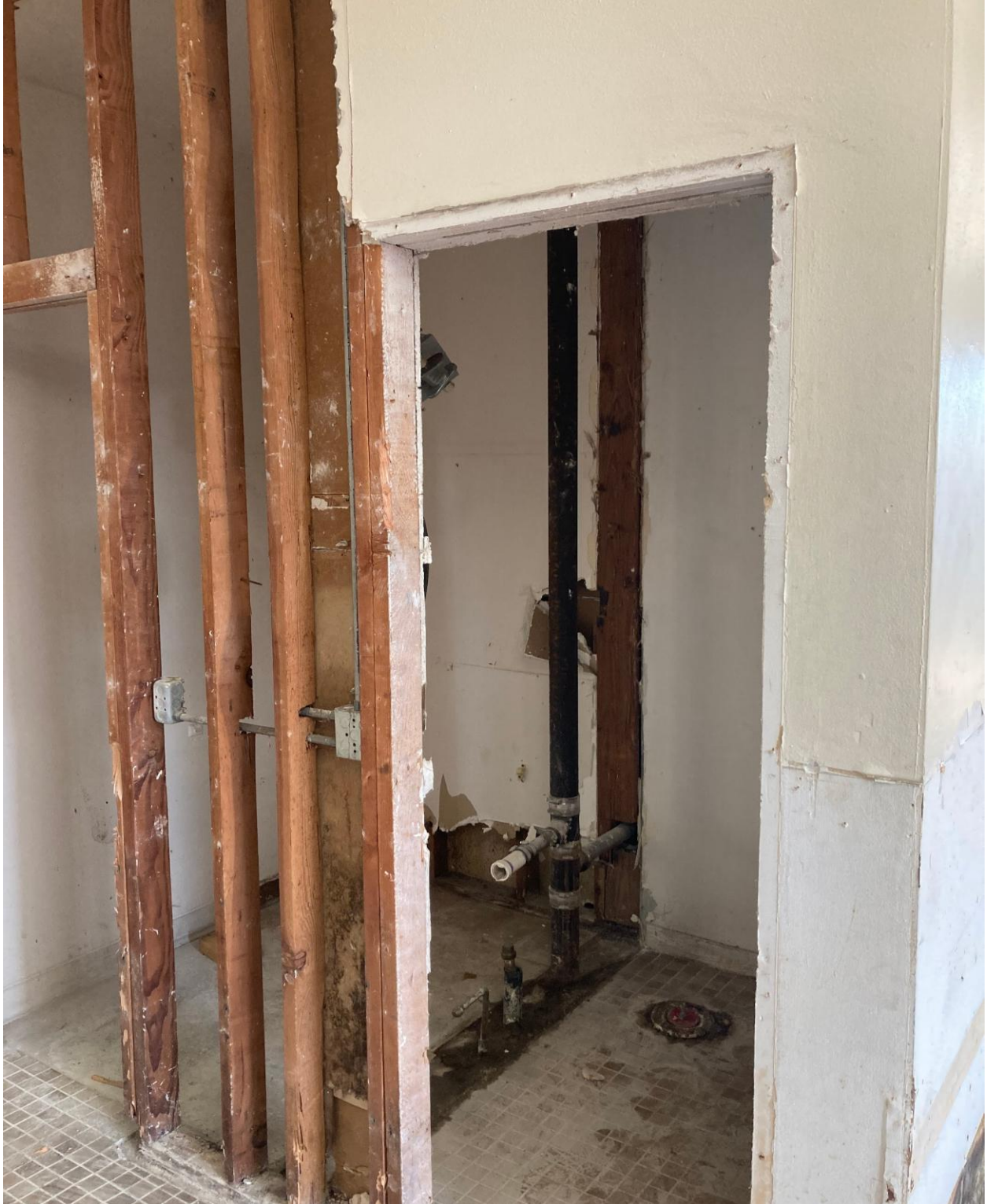
PLYMOUTH LAUNDRY- THIS WAS THE REST ROOM ON RIGHT AND SLOP SINK ROOM ON THE LEFT. THIS SPACE WILL BE MADE INTO A SINGLE ADA COMPLIANT REST ROOM.
