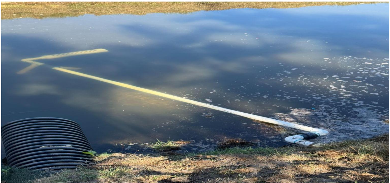
SOUTH CANAL- CHABOT IRRIGATION INSTALLED A NEW INTAKE PIPE FOR THE UCO OFFICE.
