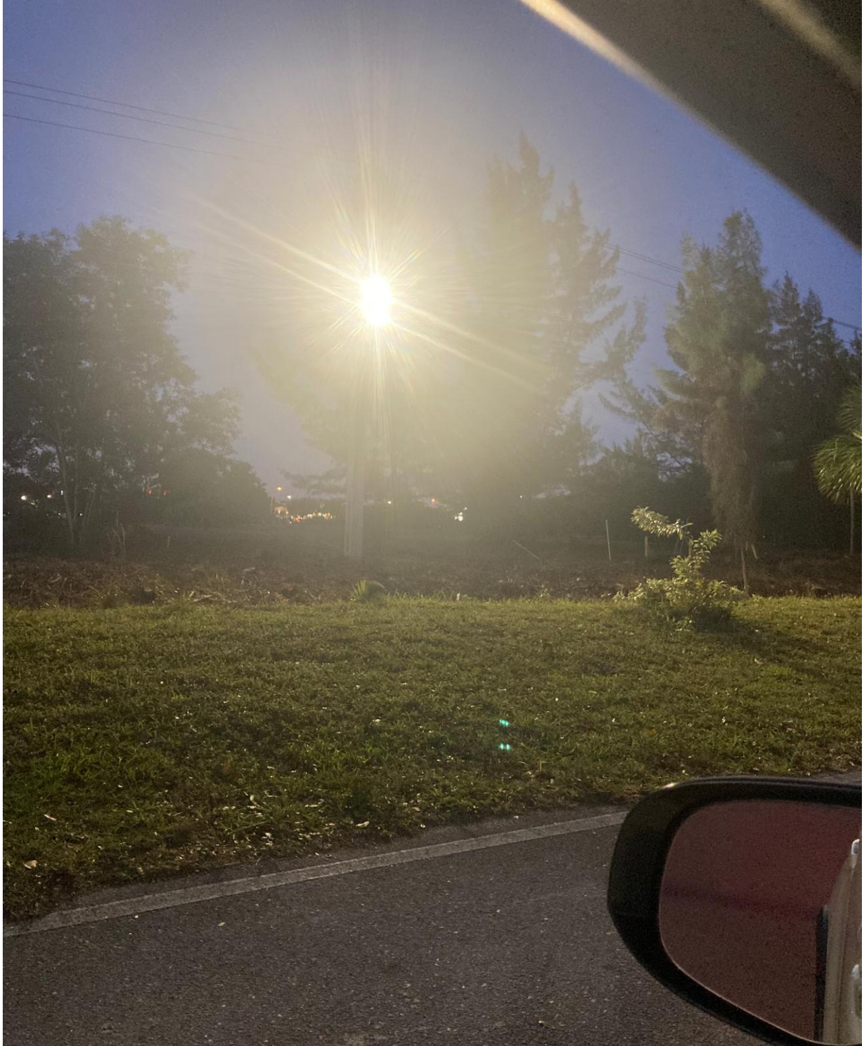
FARNHAM STREET- FPL REPAIRED SPOT LIGHTS ALONG THE SOUTH SIDE OF SOUTH CANAL. MORE STREET LIGHTS WILL BE REPAIRED SOON.
