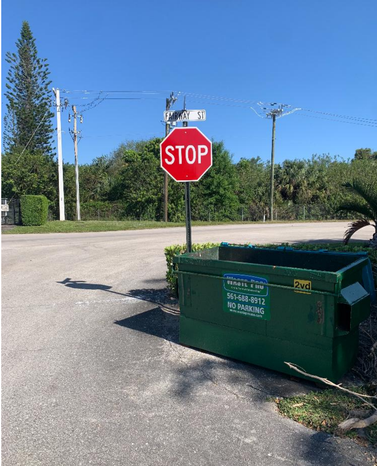
BEDFORD SECTION- HANDYMAN JOSE CONTINUES WITH REPLACEMENT OF WEATHERED AND NON-COMPLIANT STOP SIGNS.
