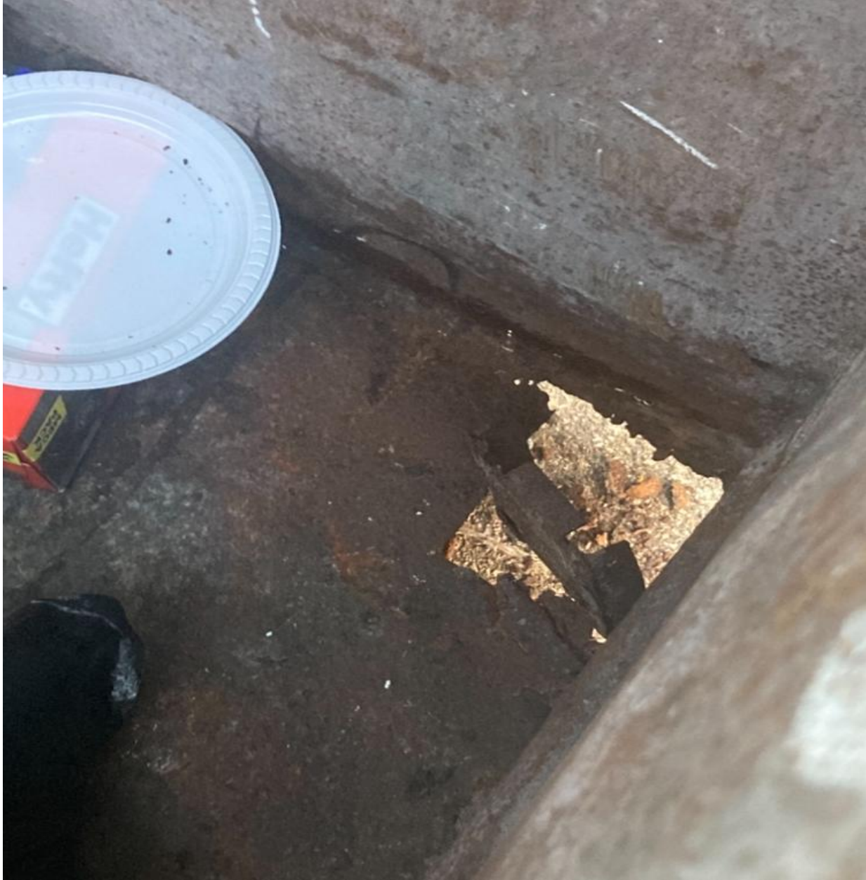
STRATFORD D- BIG HOLE AT THE BOTTOM OF THIS DUMPSTER. A REQUEST FOR REPLACEMENT WAS SENT TO WASTE PRO.
