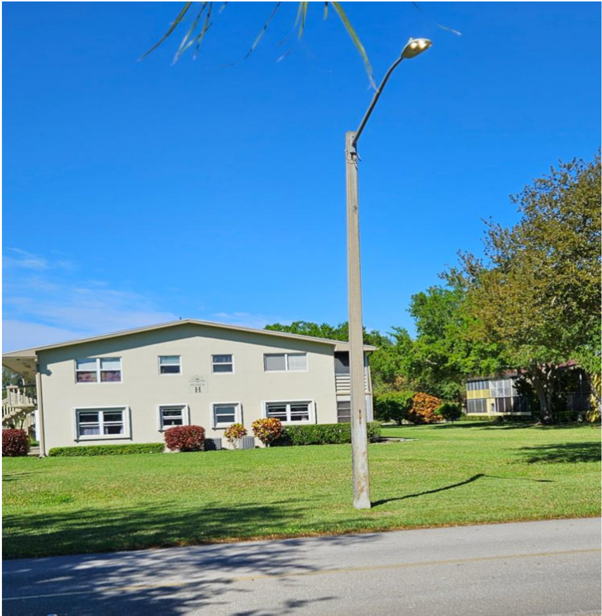
LINCOLN STREET- THIS IS A “DAYBURNER”, REPORTED IN BY A CV UNIT OWNER. A REQUEST FOR REPAIR WAS SENT TO FPL.
