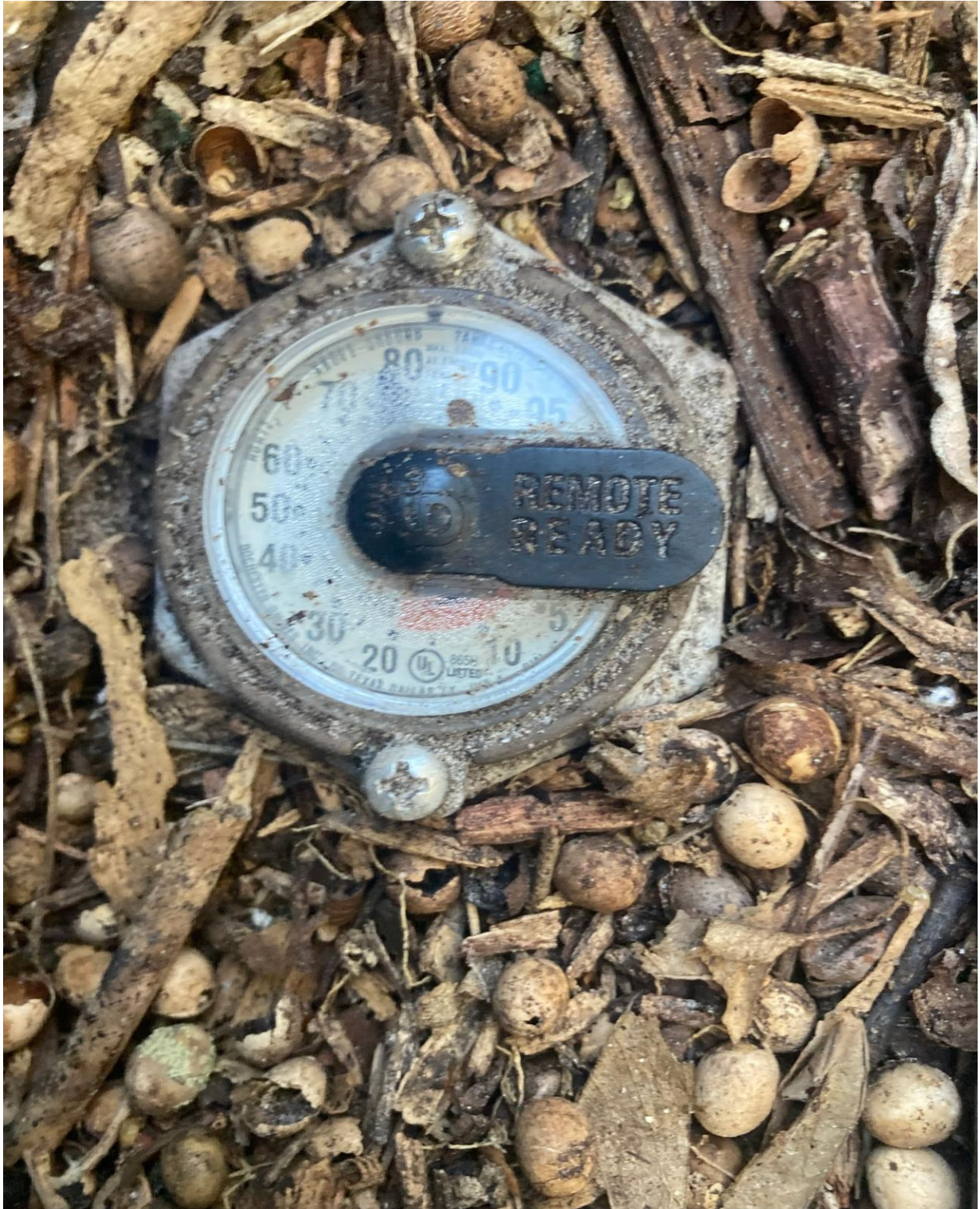
OKEECHOBEE BOULEVARD GUARDHOUSE- FUEL SUPPLY FOR THE EMERGENCY GENERATOR WAS CHECKED, 400 GALLONS.
