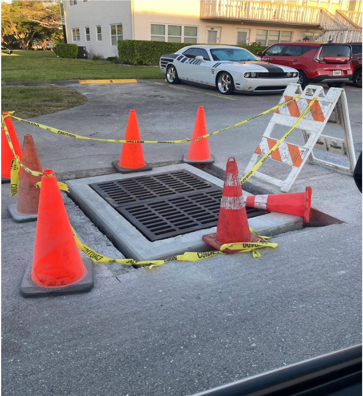
KENT SECTION- THIS DAMAGED STORM DRAIN CATCH BASIN WAS REPLACED BY FEDERAL MAINTENANCE ON 3/20.
