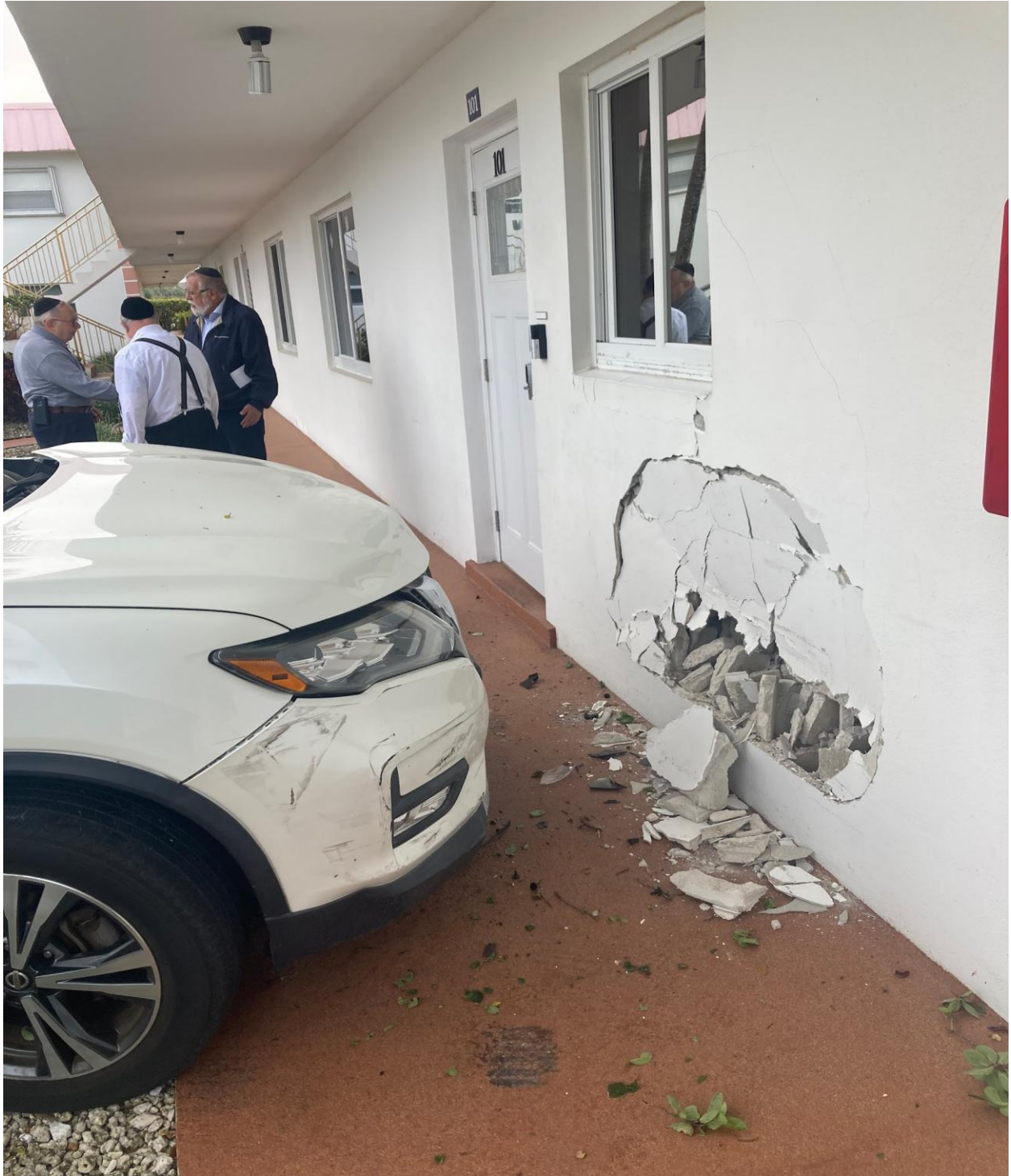
PLYMOUTH M- THIS CAR CRASHED INTO THE FRONT OF THE BUILDING ON 3/23.
