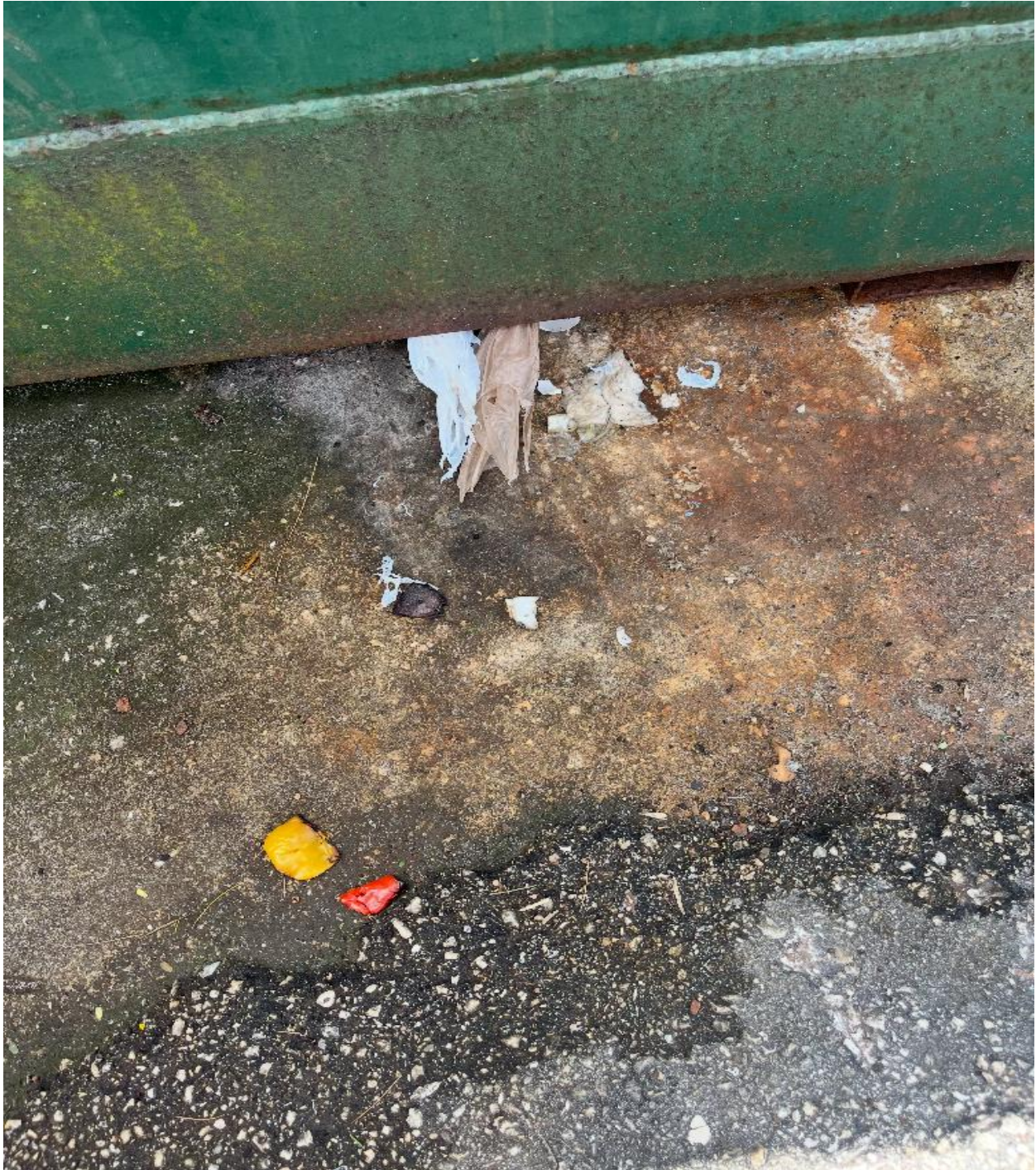
WINDSOR R/S- HOLEY DUMPSTER. REPORTED IN BY A CV UNIT OWNER. A REQUEST FOR REPLACEMENT WAS SENT TO WASTE PRO.
