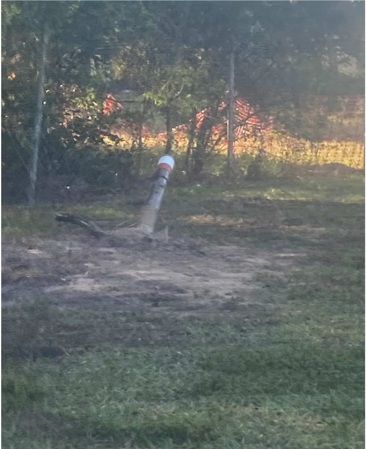
5400 FAIRWAY STREET- THIS IS WHERE THE NEW PIPE EMERGES NEXT TO THE BREEZELINE OFFICE. UNDERGROUND BORING MAKES CUTTING THE ROAD UNNECESSARY.
