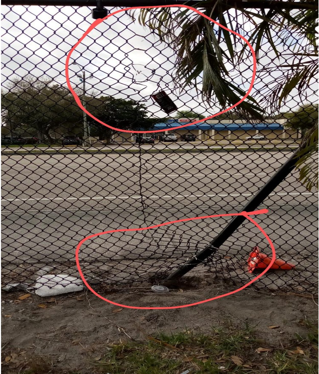
SOUTHAMPTON SECTION- THIS FENCE, DAMAGED BY AN UNKNOWN VEHICLE, WAS REPAIRED BY BUDGET FENCE AND GATE SYSTEMS.
