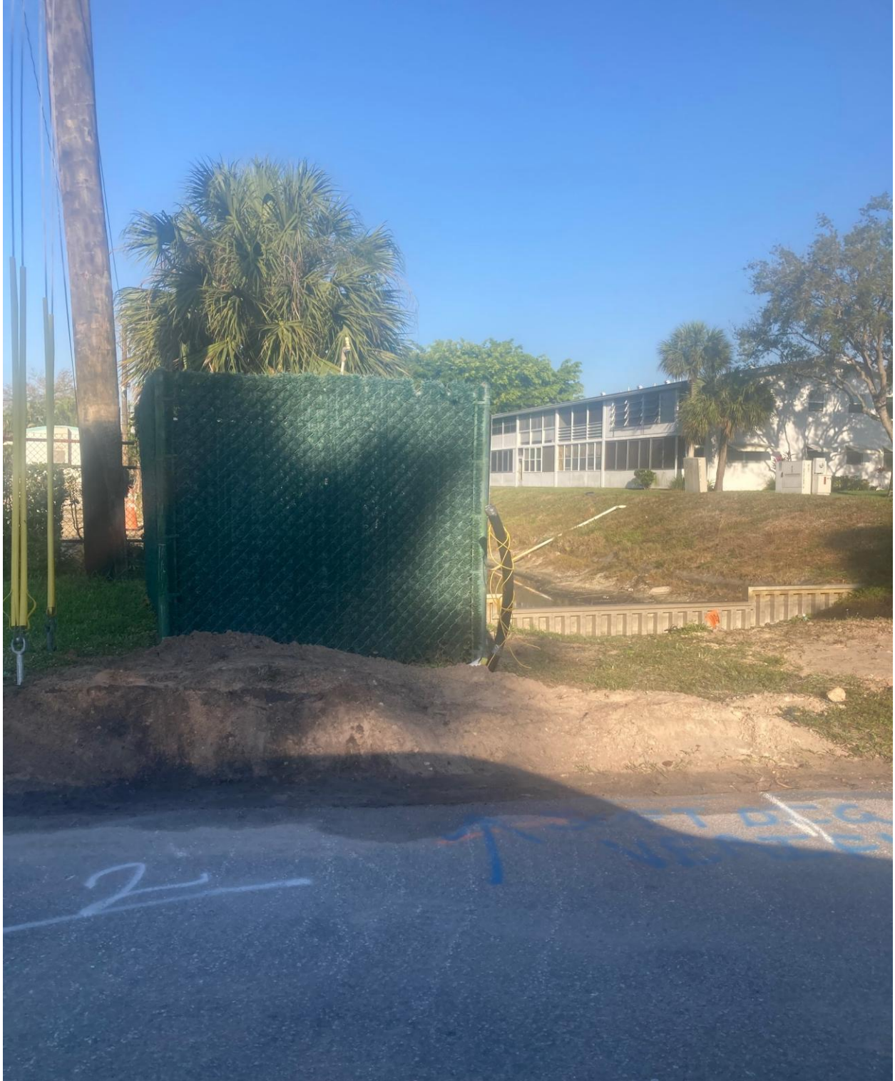
FAIRWAY STREET- A NEW IRRIGATION WATER SUPPLY PIPE WAS INSTALLED UNDER THE ROAD, BETWEEN THIS IRRIGATION PUMP STATION AND THE BREEZELINE OFFICE.
