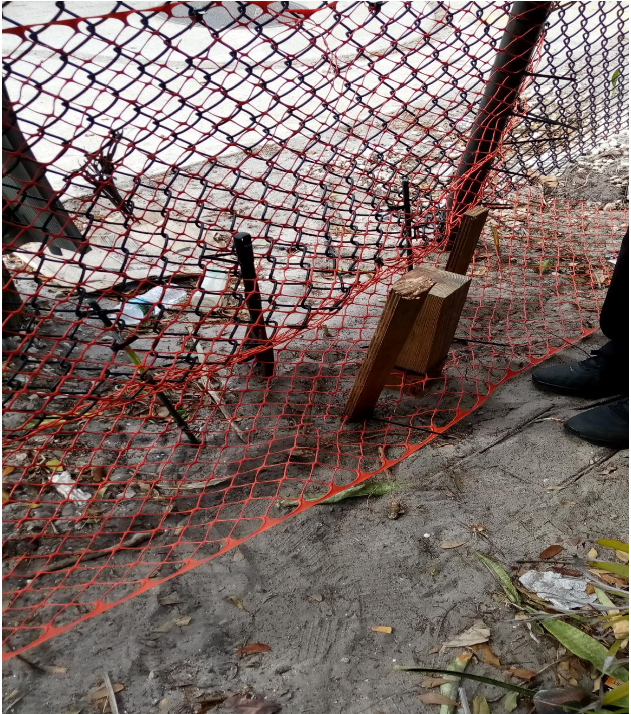
SOUTHAMPTON SECTION- TEMPORARY REPAIRS WERE MADE TO THIS FENCE, ALONG OKEECHOBEE BOULEVARD. THE FENCE WILL BE PERMANENTLY REPAIRED AND REINFORCED SOON.
