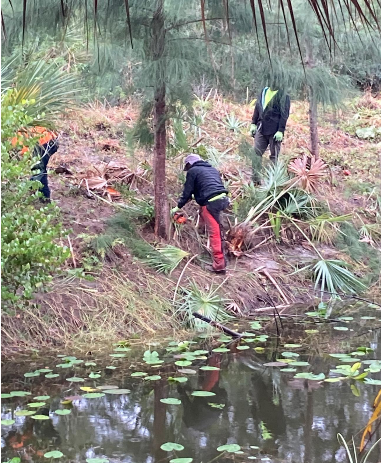
SOUTH CANAL- LAND CLEARING WORK ALONG BOTH SIDES OF THE CANAL BY SEACREST SERVICES CONTINUES. THIS SPOT IS ON THE SOUTH SIDE OF THE CANAL, NEAR ANDOVER H.
