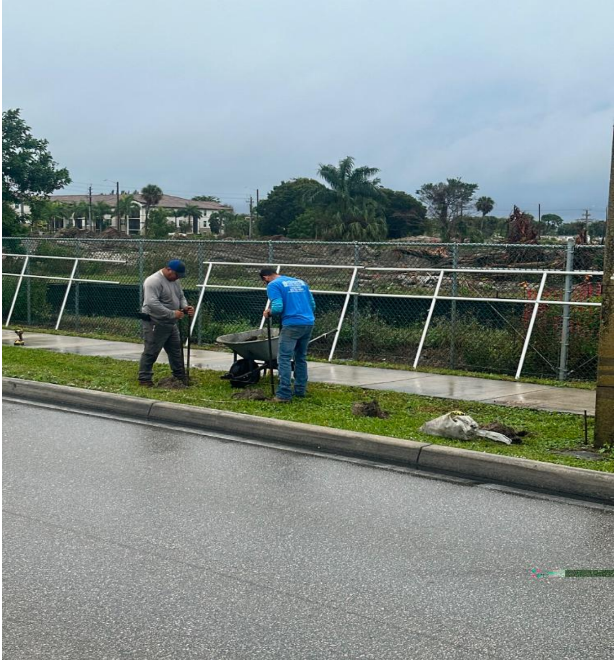
CENTURY BOULEVARD- NEW RAILINGS INSTALLED BY BUDGET FENCE AND GATE ON 1/21. THESE RAILINGS ARE INTENDED TO DETER PEDESTRIANS FROM WALKING IN THE VEHICLE TRAFFIC LANES.
