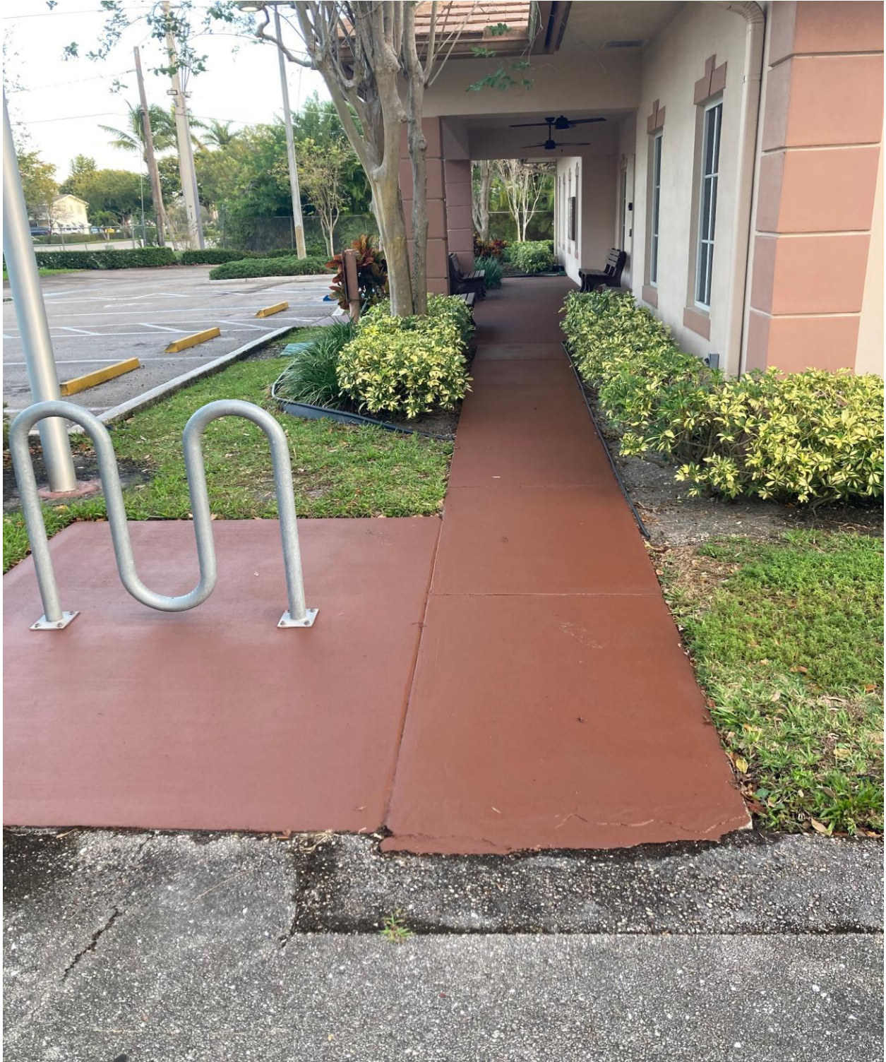
UCO OFFICE- WALKWAYS WERE PAINTED BY STRUCTURES PAINTING ON 1/6. AN ANTI-SLIP PRODUCT, SHARKGRIP, WAS ADDED TO THE PAINT TO MAKE THE WALKWAYS SLIP RESISTANT.
