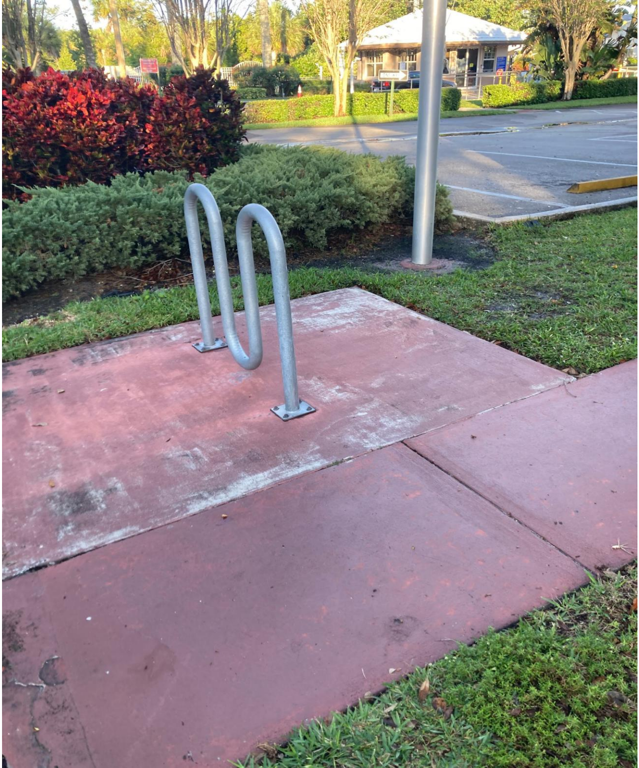
UCO OFFICE- WALKWAYS NEEDED PAINTING.
