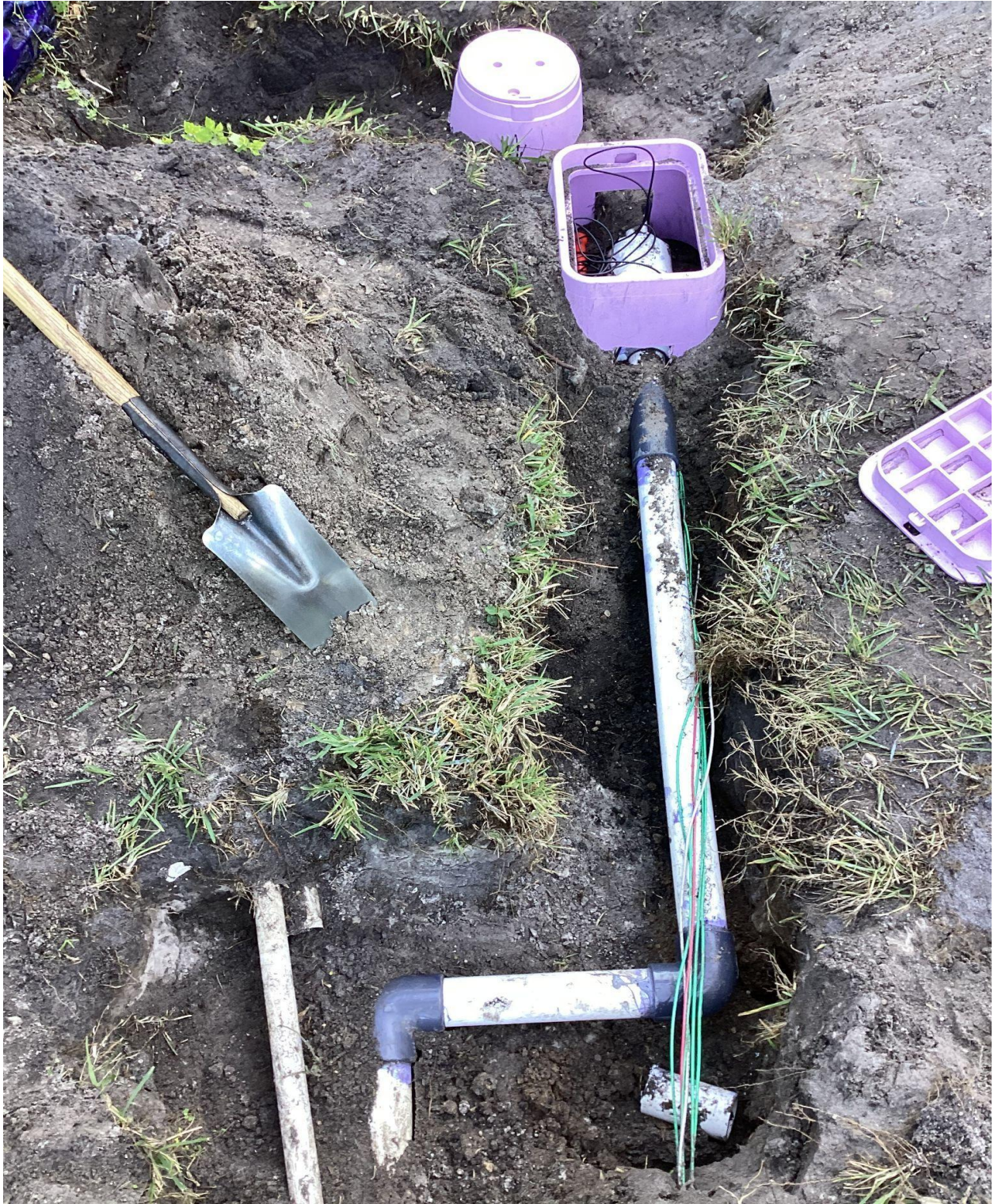
GOLFS EDGE- THE IRRIGATION REROUTE PROJECT IS NEARLY COMPLETE. THIS IS AN ELECTRIC TURN ON/OFF VALVE.
