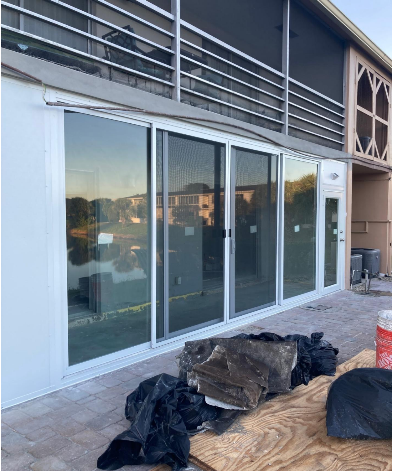
204 SOMERSET K- A PERMITTED, CODE COMPLIANT SCREENWALL, WITH HURRICANE RESISTANT GLASS, WAS INSTALLED BY BROWN'S ALUMINIUM ON 12/30/24.
