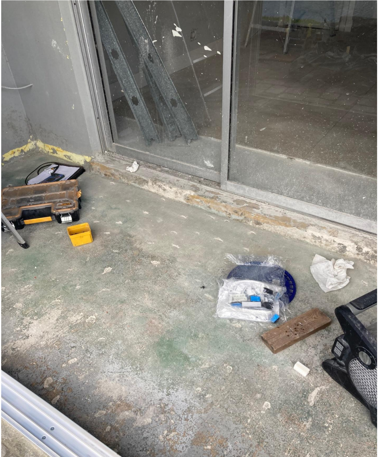
SOMERSET J- THIS UNIT OWNER REMOVED THE POORLY POURED CONCRETE SLAB, REPAIRED PREVIOUS STRUCTURAL DAMAGE, AND INSTALLED A CODE COMPLIANT REAR SCREENWALL.
