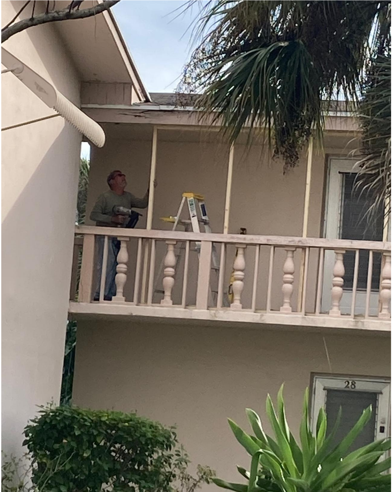
NORWICH B- EMERGENCY REPAIR WORK BEGAN ON 1/2. NOTE THE ROTTING FASCIA BOARD AND ROOF EAVES.
