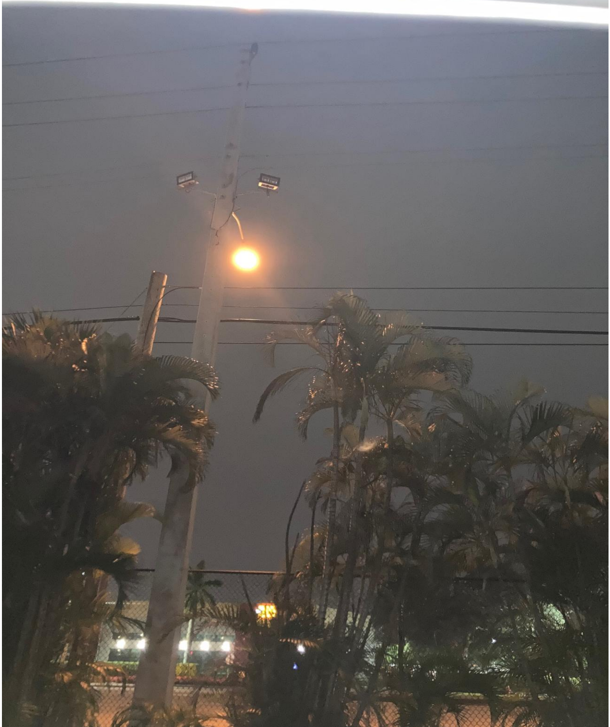
FAIRWAY STREET- DARK SPOT LIGHTS ALONG OKEECHOBEE BOULEVARD. REPORTED TO FPL, W.O. #41955.
