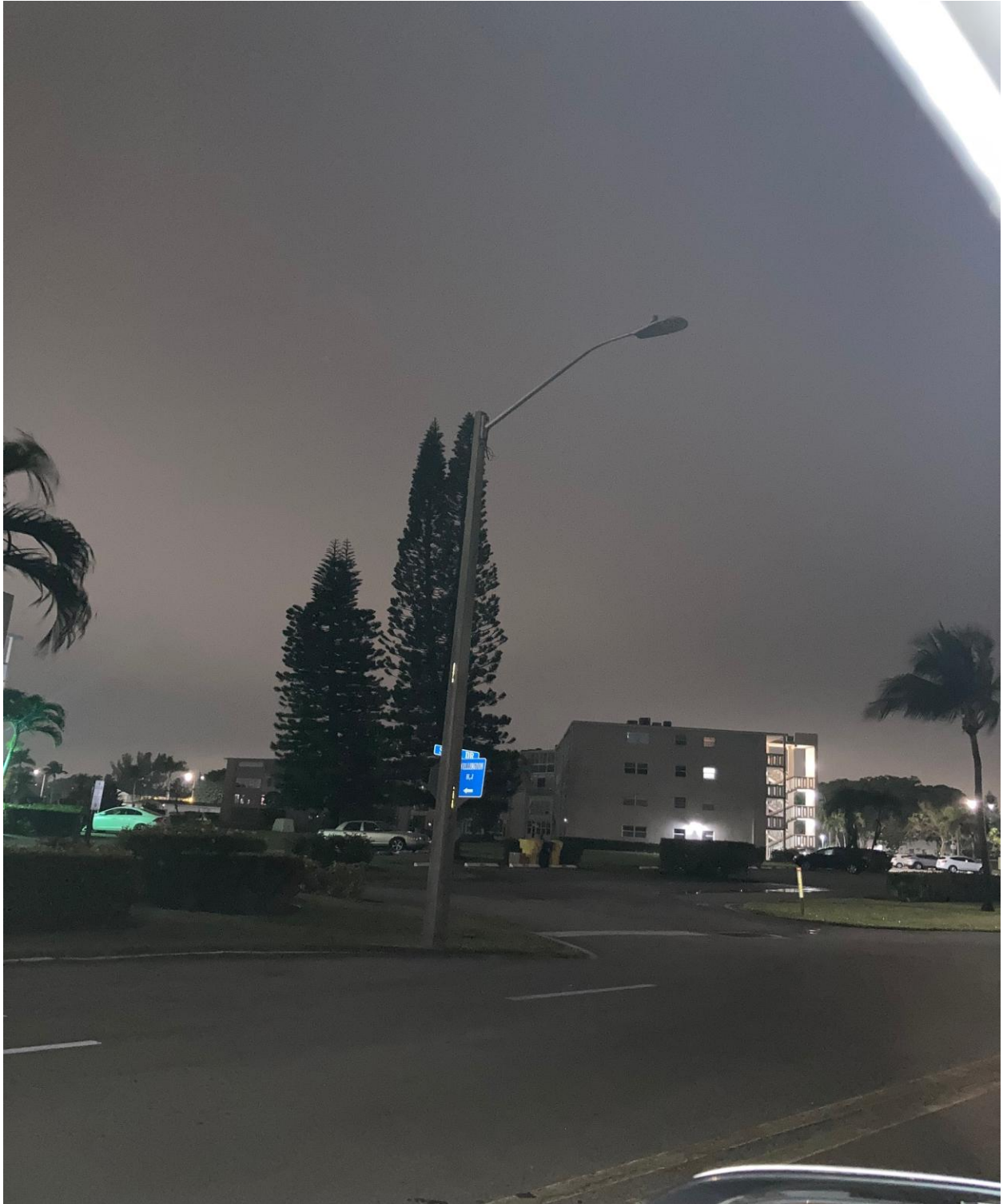
SOUTH DRIVE- DARK STREET LIGHT. REPORTED TO FPL, W.O. #41948.
