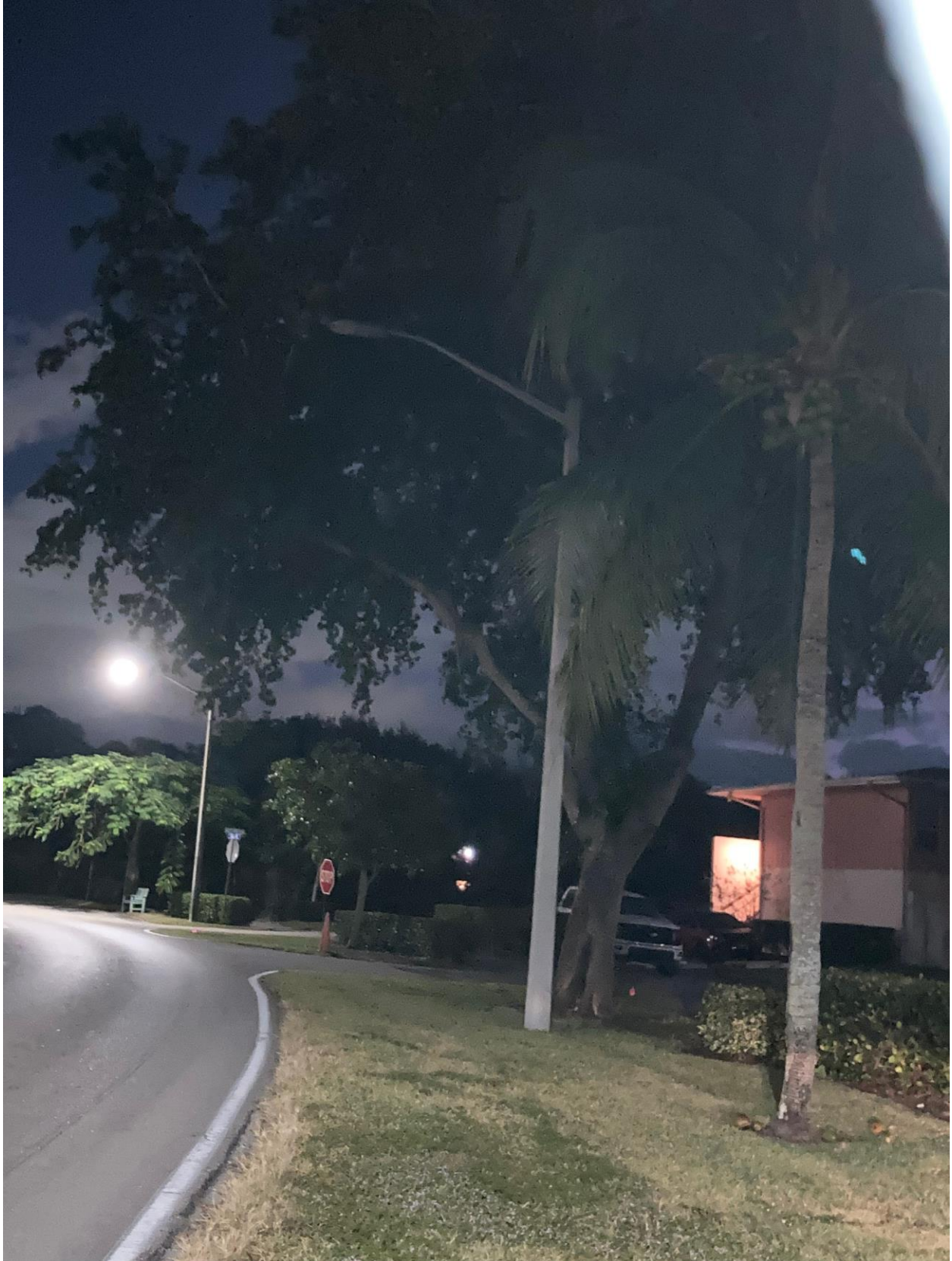
EAST DRIVE- DARK STREETLIGHT. REPORTED TO FPL, W.O. #49596.
