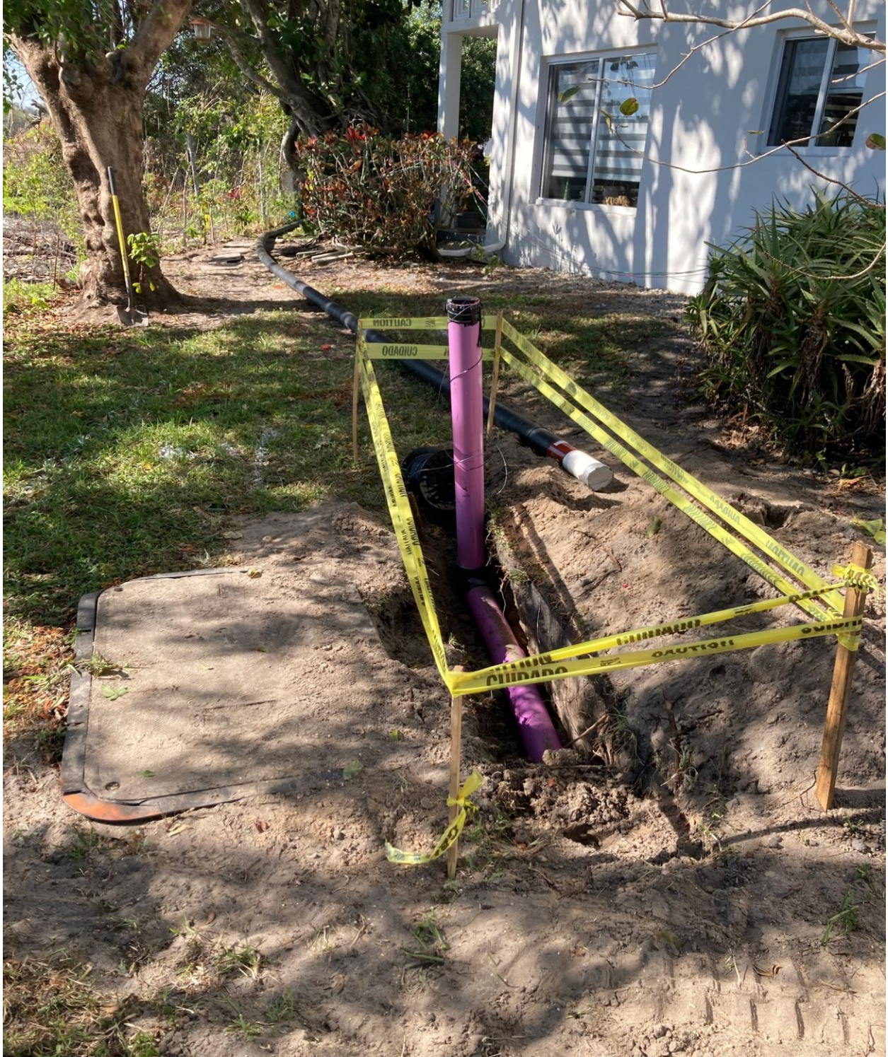
GREENBRIER C- INSTALLATION OF NEW UNDERGROUND IRRIGATION PIPES CONTINUES. THE LILAC COLORED PIPES INDICATE RECLAIMED, NON POTABLE WATER, WHICH IS SUPPLIED TO CV BY PBC WATER.
