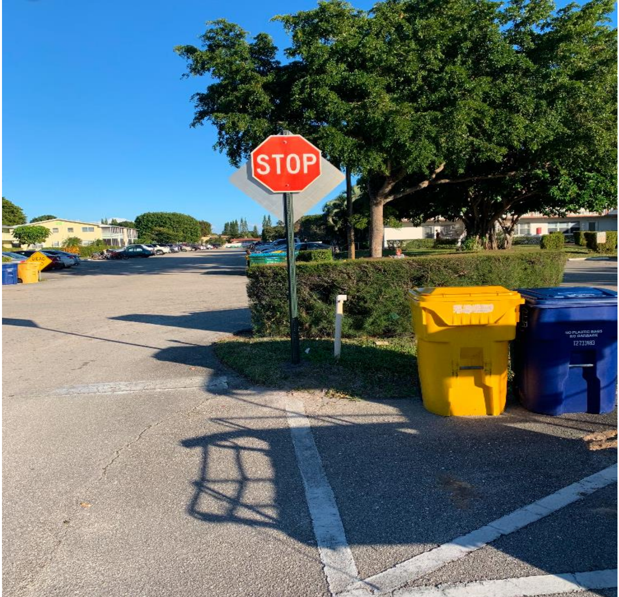
CAMBRIDGE SECTION- HANDYMAN JOSE CONTINUES WITH INSTALLING NEW, CODE COMPLIANT STOP SIGNS AND REPAINTING STOP BARS.
