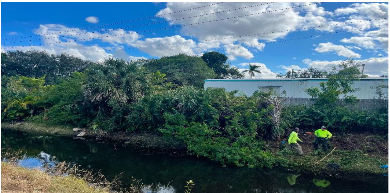
SOUTH CANAL- SEACREST SERVICES HAS BEGUN LAND CLEARING WORK ALONG THIS CANAL, WHICH STRETCHES FROM SOUTHAMPTON TO WINDSOR SECTIONS.
