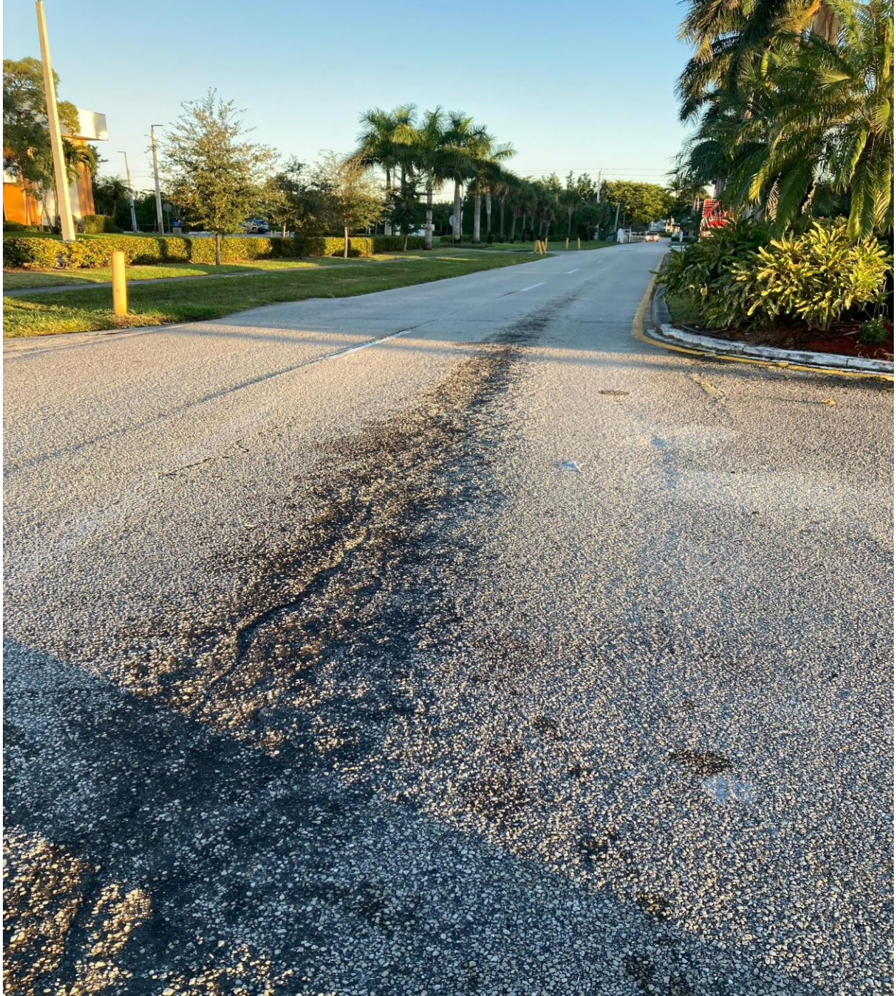
WEST DRIVE- THIS IS ONE OF TWENTY LOCATIONS THAT WILL BE REPAIRED BY SUNSHINE SERVICES UNLIMITED NEXT MONTH.
