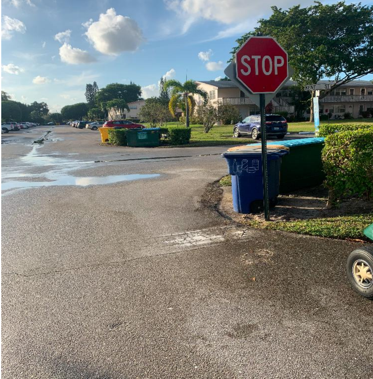
DORCHESTER SECTION- HANDYMAN JOSE CONTINUES WITH REPLACEMENT OF MIDGET STOP SIGNS. WHITE STOP BARS WILL BE PAINTED AS WELL.
