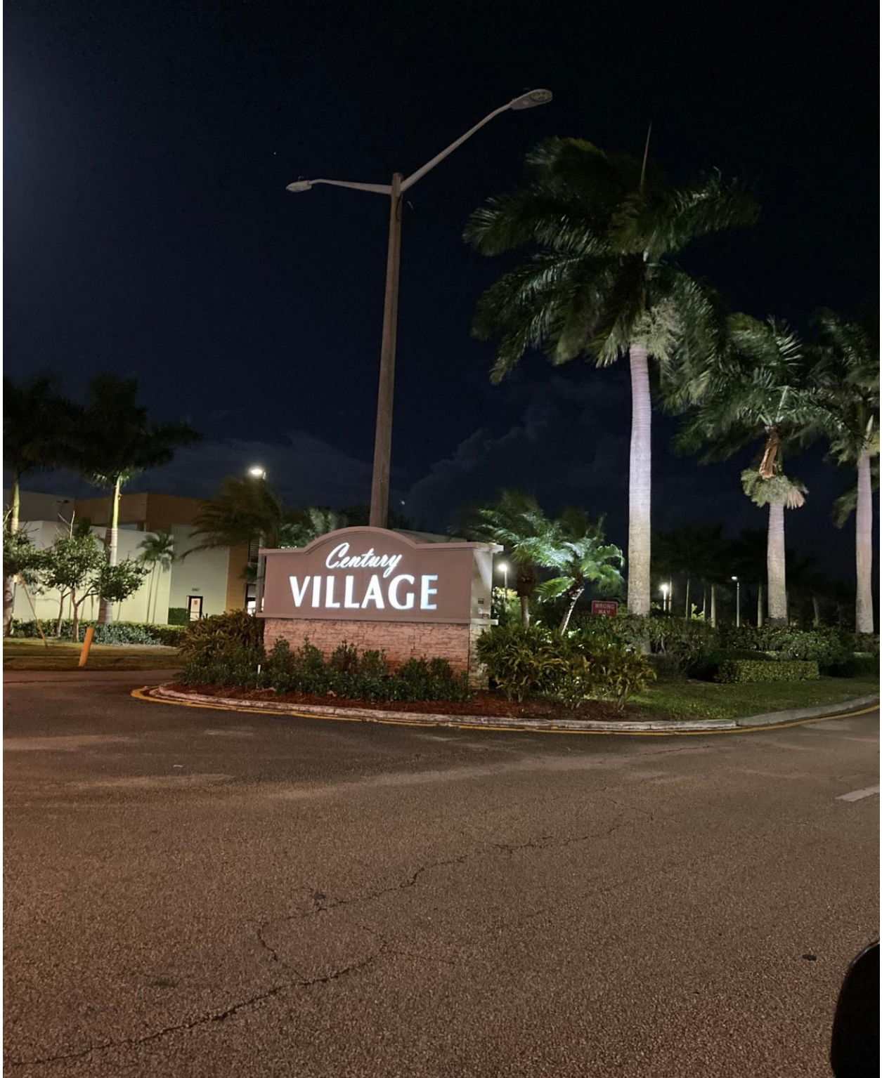
CENTURY BOULEVARD- THREE STREET LIGHT FIXTURES WENT DARK ON 12/13. THIS WAS REPORTED TO FPL, TICKET #40116.
