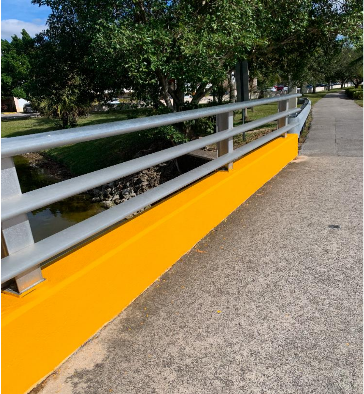
EAST DRIVE- DOT TRAFFIC YELLOW PAINT IS USED FOR THESE BRIDGES, PER THE DOT TRAFFIC MANUAL.
