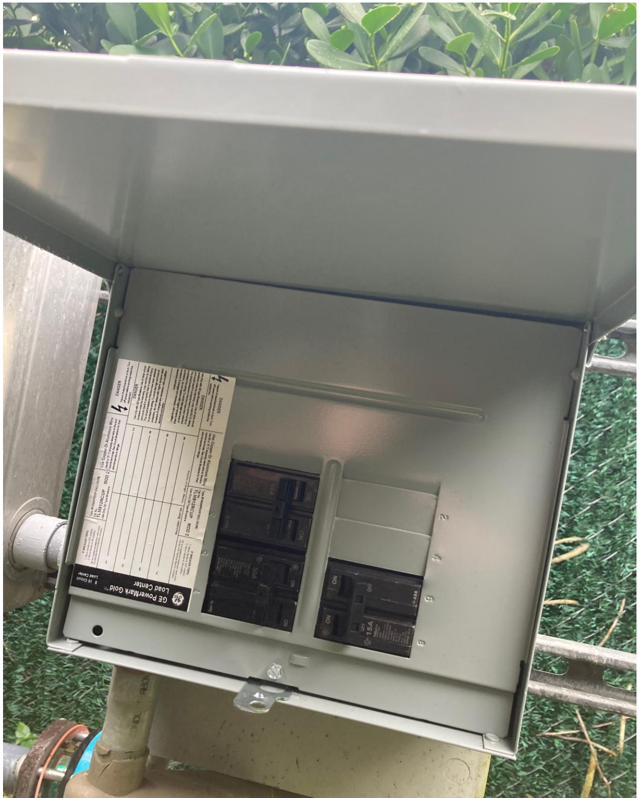
STRATFORD E- NEW ELECTRICAL PANEL INSTALLED AT THE IRRIGATION PUMP STATION BY T.S.I. ELECTRIC ON 12/12
