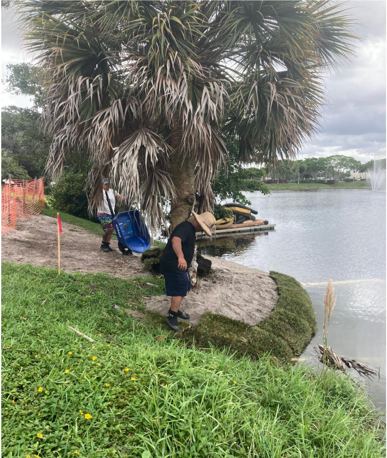
CV MEDICAL BUILDING- THE GEOTUBE AND SOIL ARE COVERED WITH NEW SOD.
