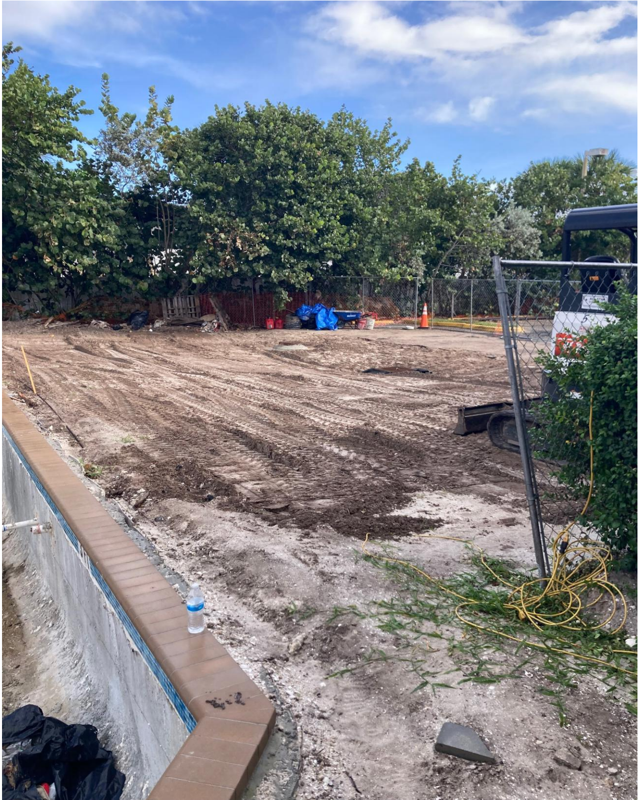
100 CENTURY BOULEVARD- CONSTRUCTION WORK FOR TWO SWIMMING POOLS AT THE CV MEDICAL BUILDING HAS RESUMED.
