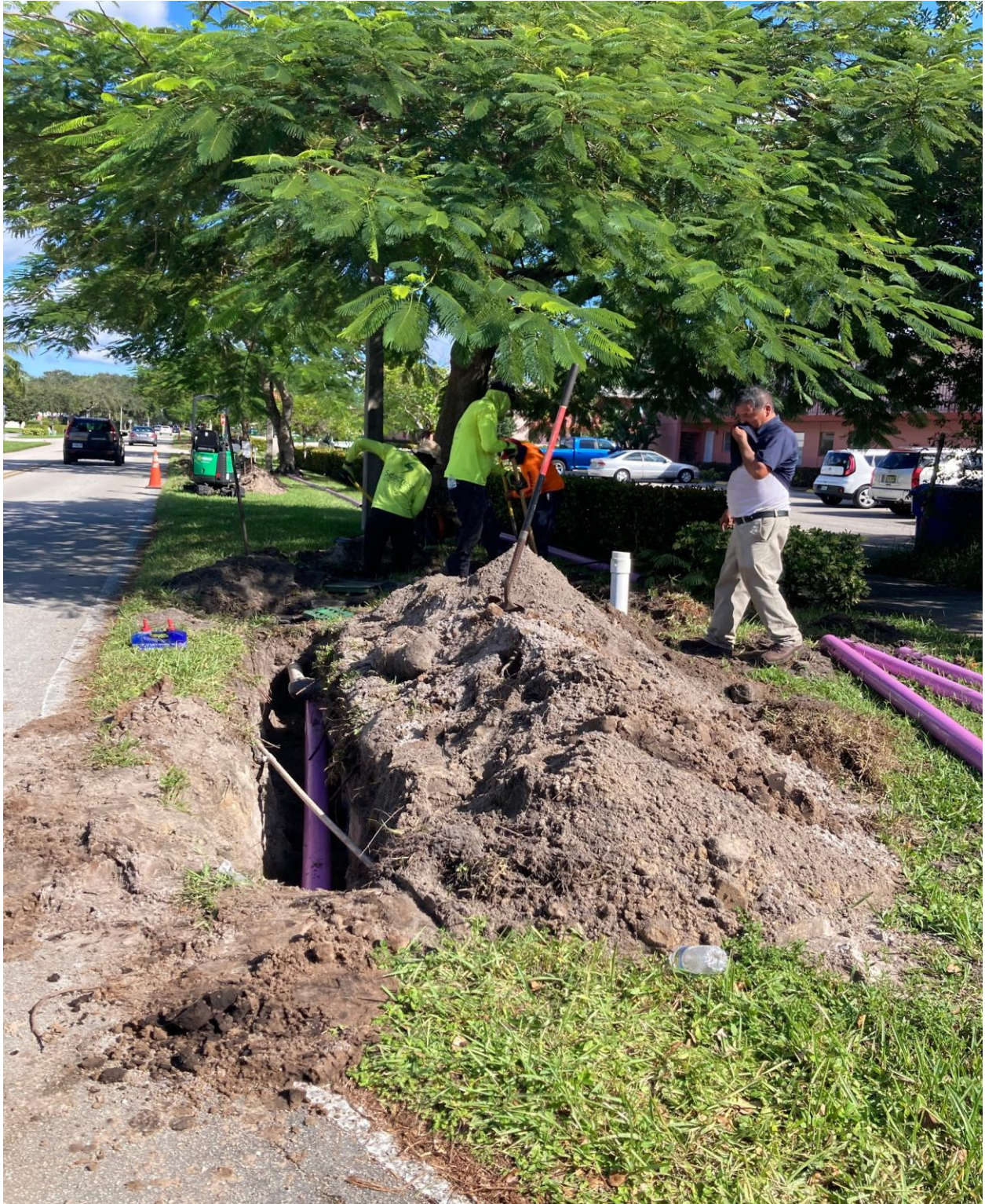
EAST DRIVE, GOLFS EDGE SECTION- SEACREST SERVICES CONTINUES WITH THIS IRRIGATION REROUTE PROJECT. LILAC COLOR PIPES INDICATE RECLAIMED WATER.
