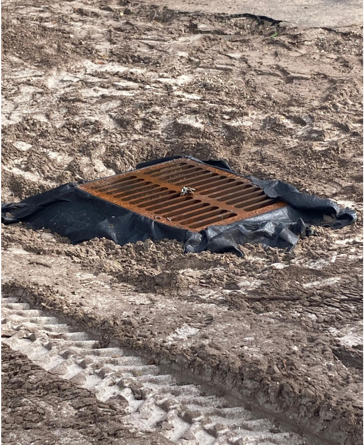
100 CENTURY BOULEVARD- P.B. COUNTY REQUIRED THE PROPERTY OWNER TO INSTALL A NEW STORMWATER CATCH BASIN, MANHOLE BOX, AND UNDERGROUND CULVERT PIPES.
