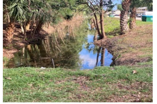
NORTH CANAL- KEEPING THIS CANAL CLEAR OF TREES AND PALM FRONDS IS THE FIRST STEP IN MAKING THIS CRITICAL PIECE OF INFRASTRUCTURE DO A BETTER JOB OF HANDLING STORM WATER.
