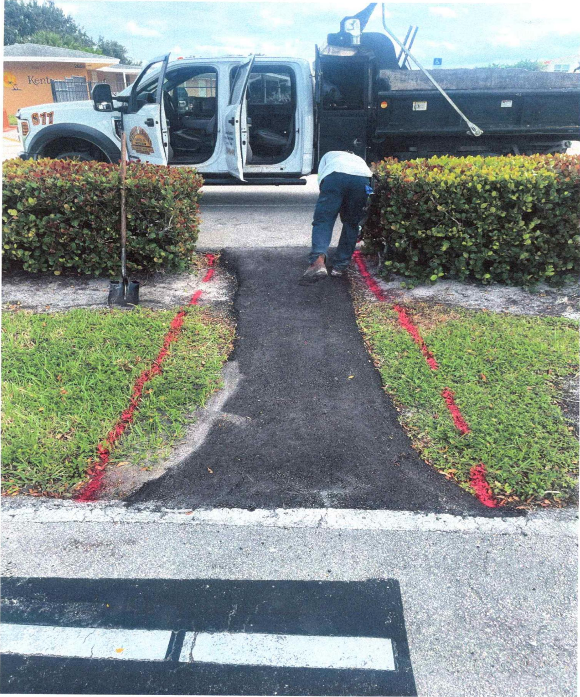
WEST DRIVE- THIS WALKWAY, NEAR KENT POOL, NEEDED TO BE WIDENED TO FIVE FEET, WITH STRAIGHT EDGES.
