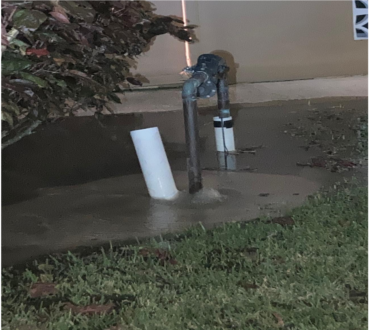
CAMDEN POOL- POTABLE WATER LEAK AT BACKFLOW VALVE. CALLED IN BY A CV UNIT OWNER ON 10/19. PBC WATER WAS CALLED AT 9:00 PM. REPAIR CREW ARRIVED 9:57 PM.
