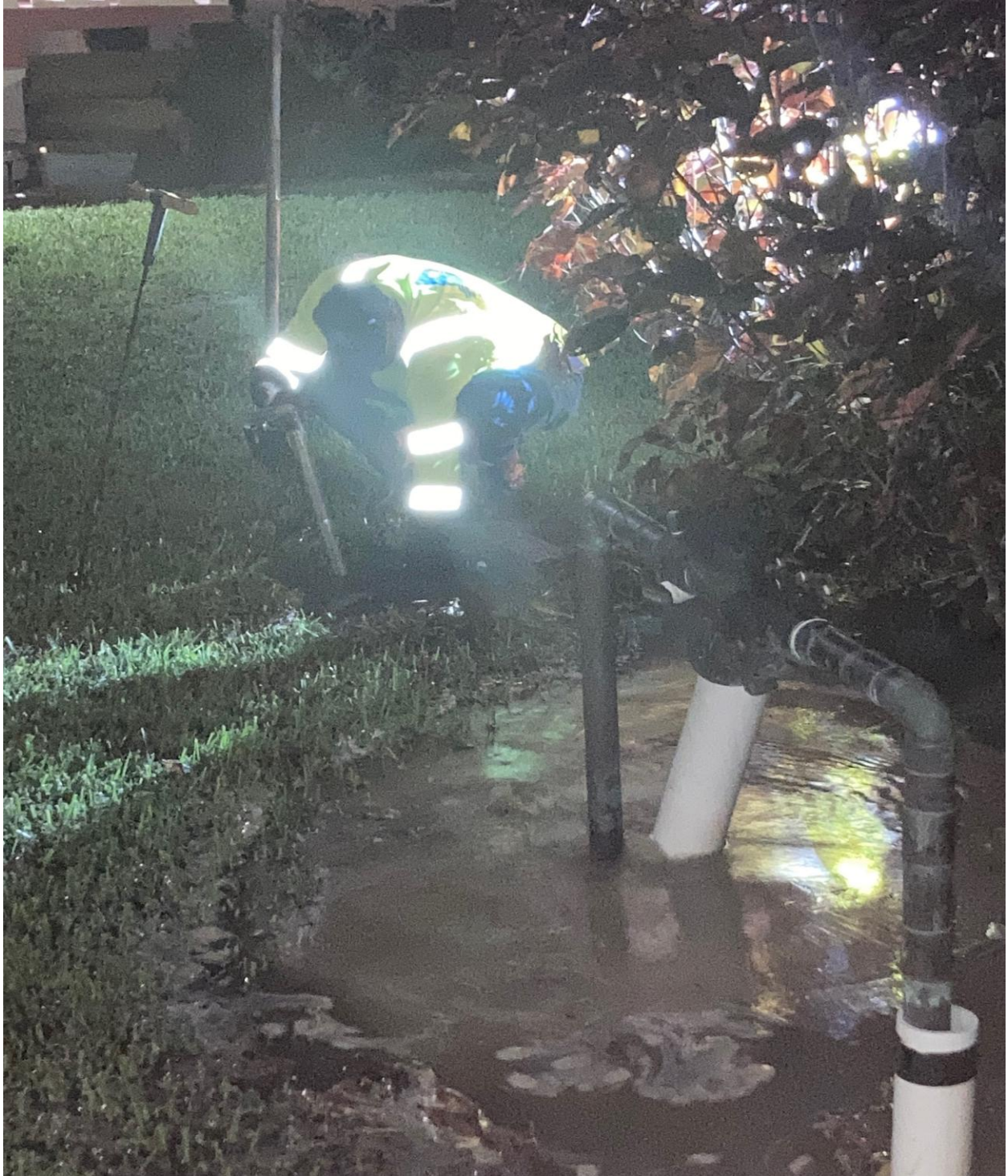
CAMDEN POOL- THE SHUT OFF VALVE FOR THE POOL HOUSE WAS TURNED OFF BY PBC WATER TO STOP THE LEAK. CAMDEN POOL IS CLOSED UNTIL THE LEAK CAN BE REPAIRED.
