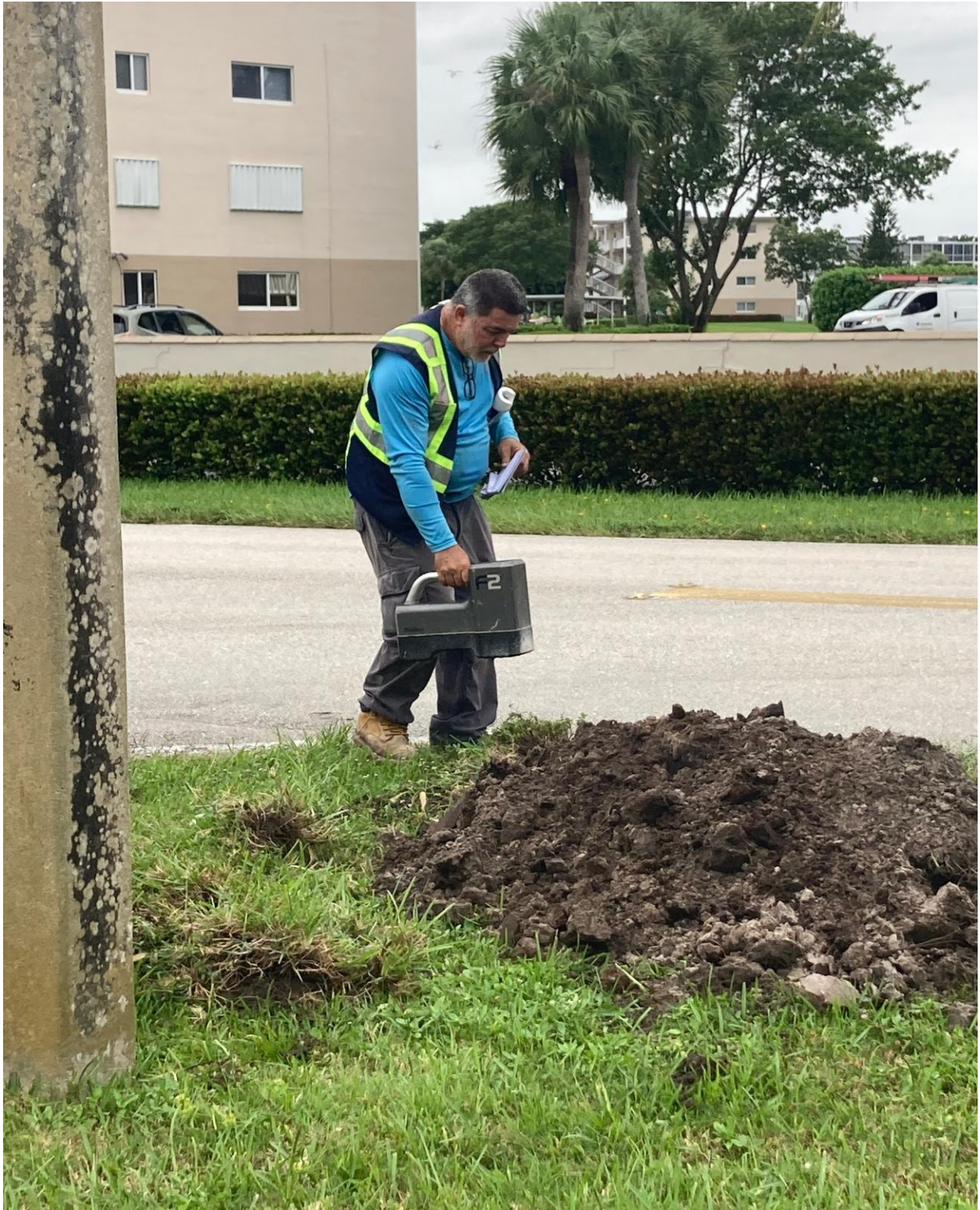
WEST DRIVE, GOLFS EDGE- THIS WORKER IS USING A DOPPLER RADAR DEVICE TO CONFIRM THE LOCATION AND DEPTH OF THE NEW UNDERGROUND IRRIGATION LINE.
