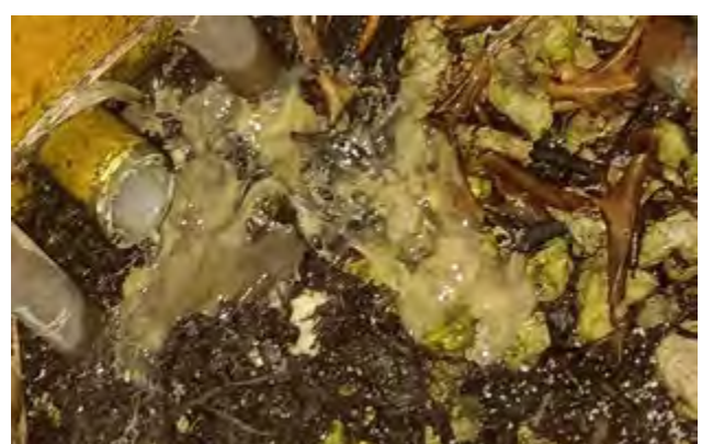
OXFORD SECTION- THIS IS THE “GUNK” THAT BUILDS UP INSIDE AN AC CONDENSATE DRAIN LINE. TO AVOID BACKUPS AND LEAKS, ASSOCIATIONS SHOULD SCHEDULE CLEANOUTS FOR THESE LINES AT LEAST ANNUALLY. IF LEFT TO THE UNIT OWNERS, THE JOB WON'T BE DONE, AND THERE WILL BE LEAKS. AND CLAIMS.
