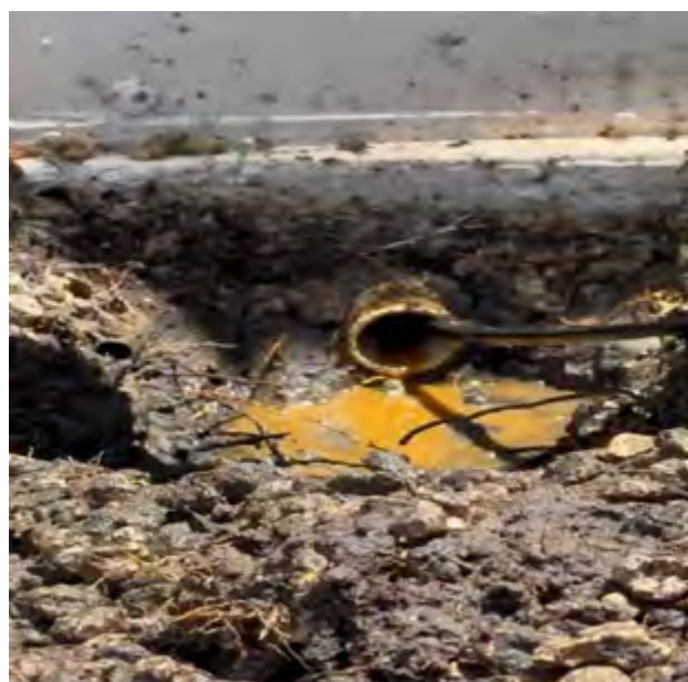
GREENBRIER C- THESE COMMON AC CONDENSATE DRAIN LINES NEED TO BE JETTED OUT AT LEAST ANNUALLY, TO PREVENT BACKUPS AND LEAKS.
