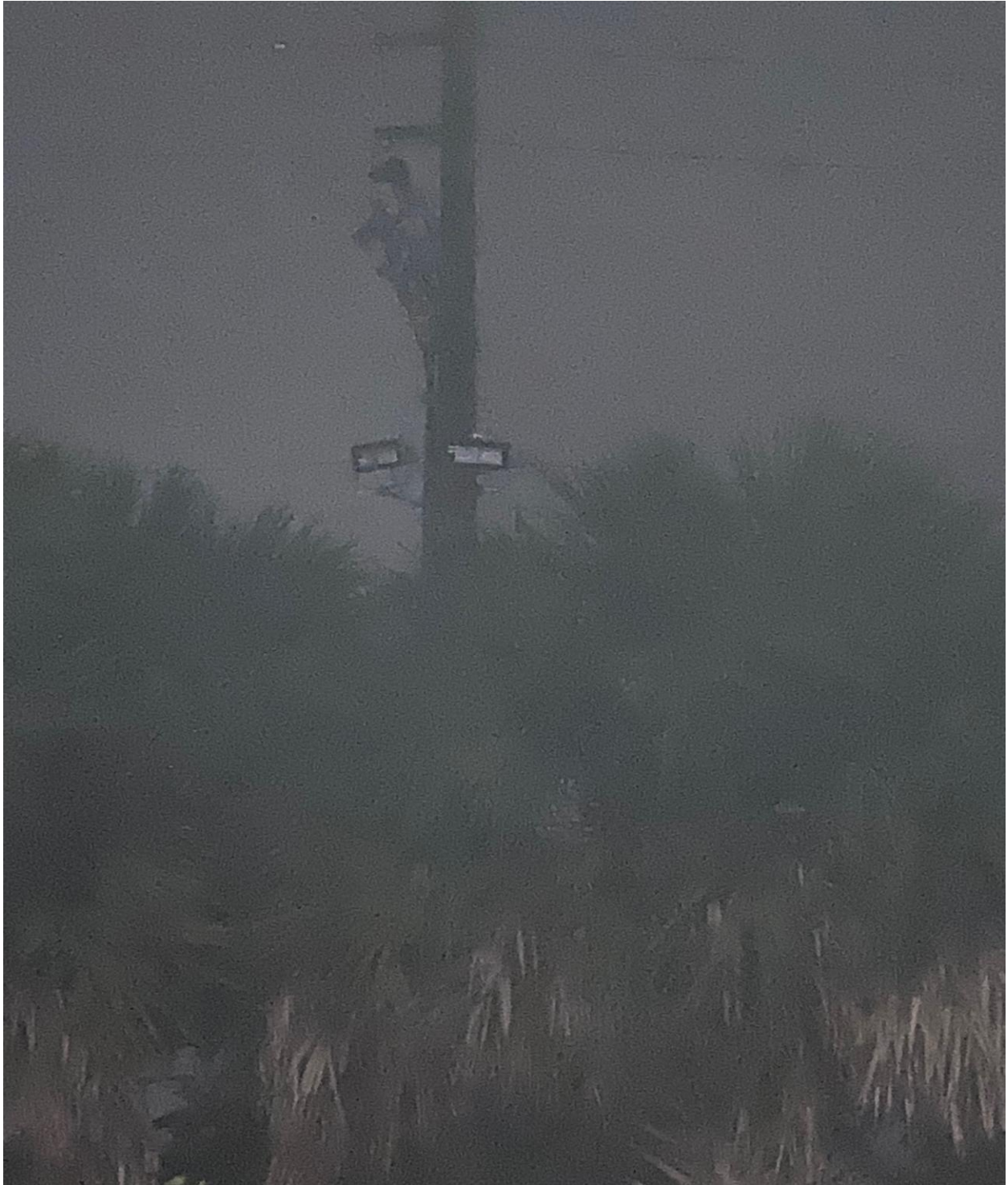
NORTH HAMPSHIRE STREET, ANDOVER SECTION. DARK FLOODLIGHTS. REPORTED TO FPL FOR REPAIR, TICKET #44154.
