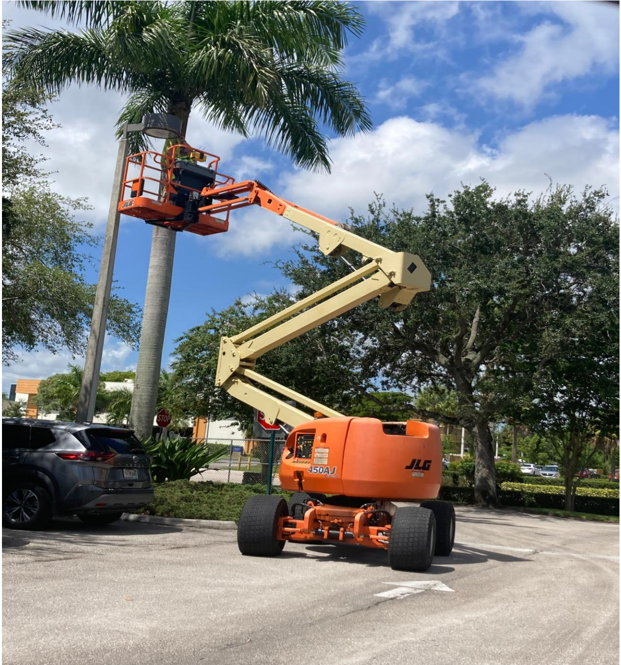
UCO OFFICE- SEACREST SERVICES REPAIRED STREET LIGHTS AT THE UCO OFFICE PARKING LOT ON 9/11.
