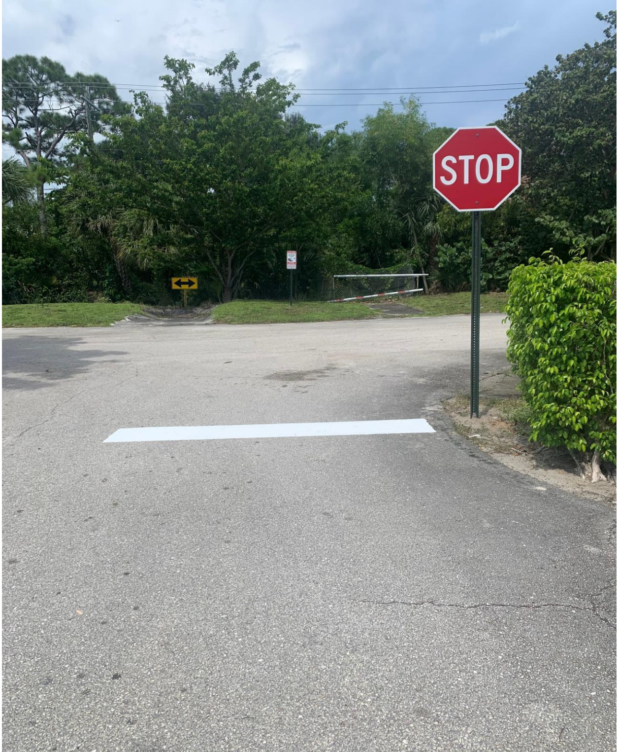
COVENTRY SECTION- NEW STOP SIGN AND STOP BAR. HANDYMAN JOSE IS WORKING ON THIS PROJECT, A FEW EACH WEEK.
