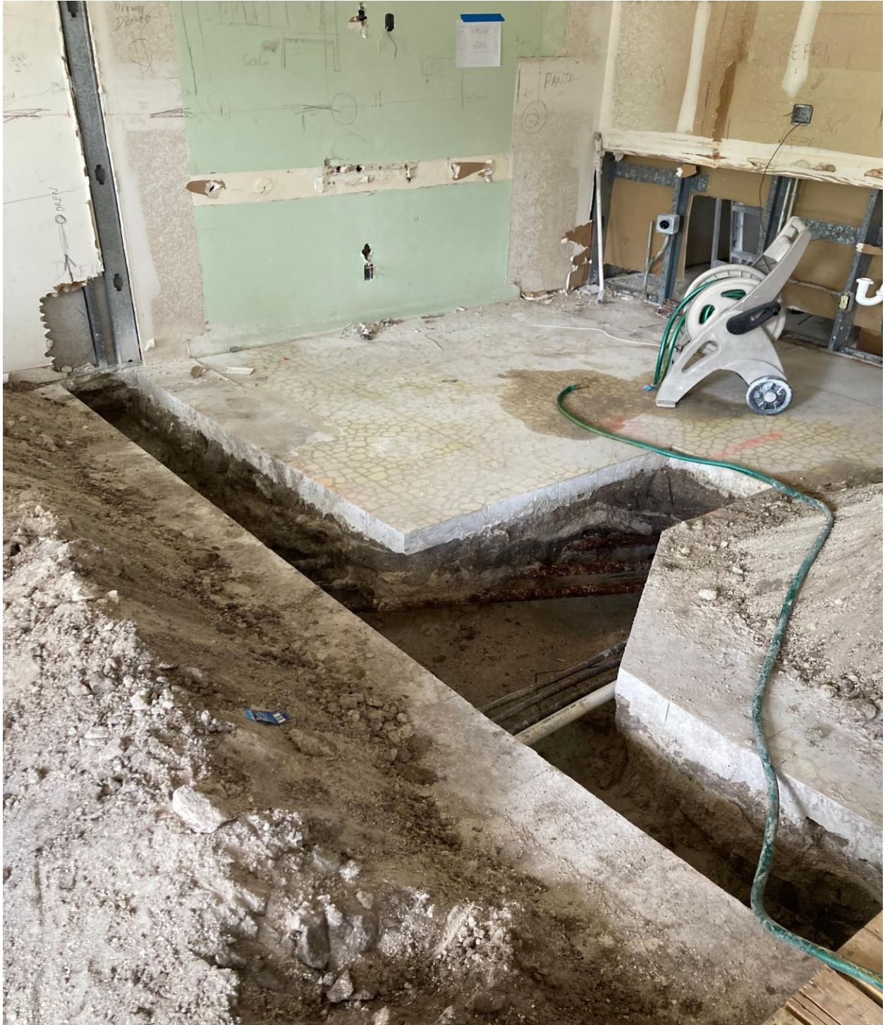
112 WELLINGTON E- THIS UNIT OWNER CUT AND REMOVED SECTIONS OF THE CONCRETE SLAB FLOOR, A STRUCTURAL ELEMENT OF THE BUILDING, AND DUG TRENCHES ACROSS THE KITCHEN AND DINING ROOM AREAS OF THE UNIT.
