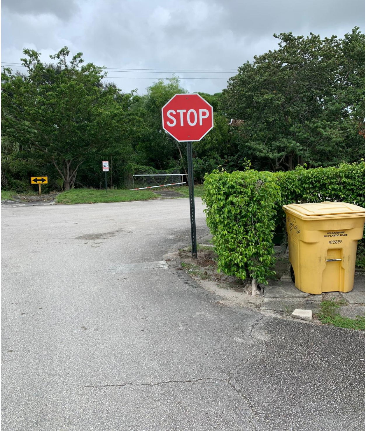
COVENTRY SECTION- NEW, MANUAL COMPLIANT STOP SIGN INSTALLED BY HANDYMAN JOSE. FADED STOP BAR WILL BE PAINTED AS WELL.
