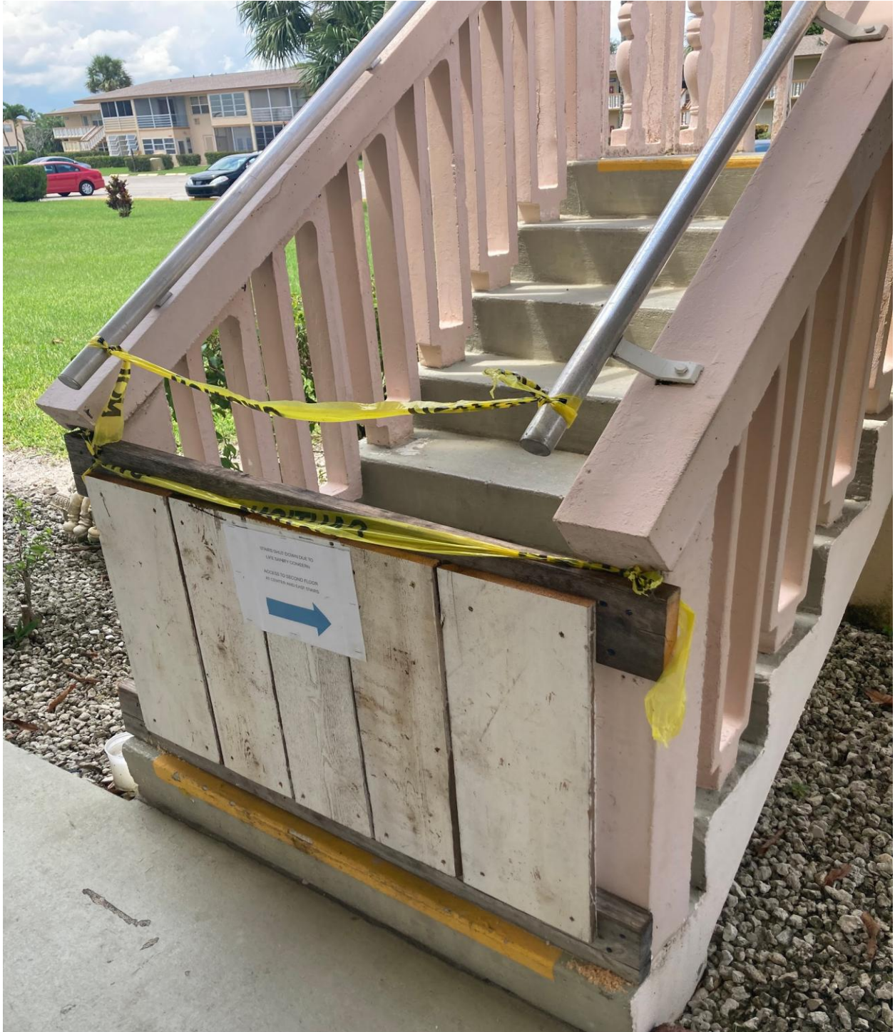
NORWICH B- THE PZB SPECIAL MAGISTRATE ORDERED THAT THIS STAIRWAY BE BARRICADED TO KEEP PEOPLE OFF.
