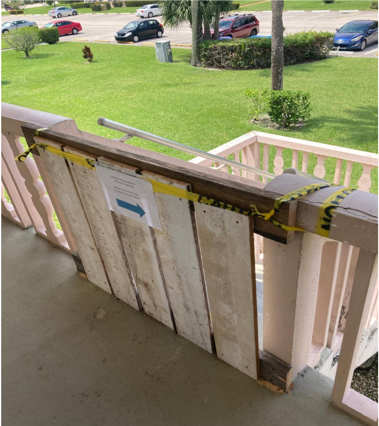
NORWICH B- THE SECOND FLOOR RESIDENTS OF THIS BUILDING MUST WALK OVER TO THE OTHER TWO STAIRCASES TO GET OUT OF THE BUILDING.
