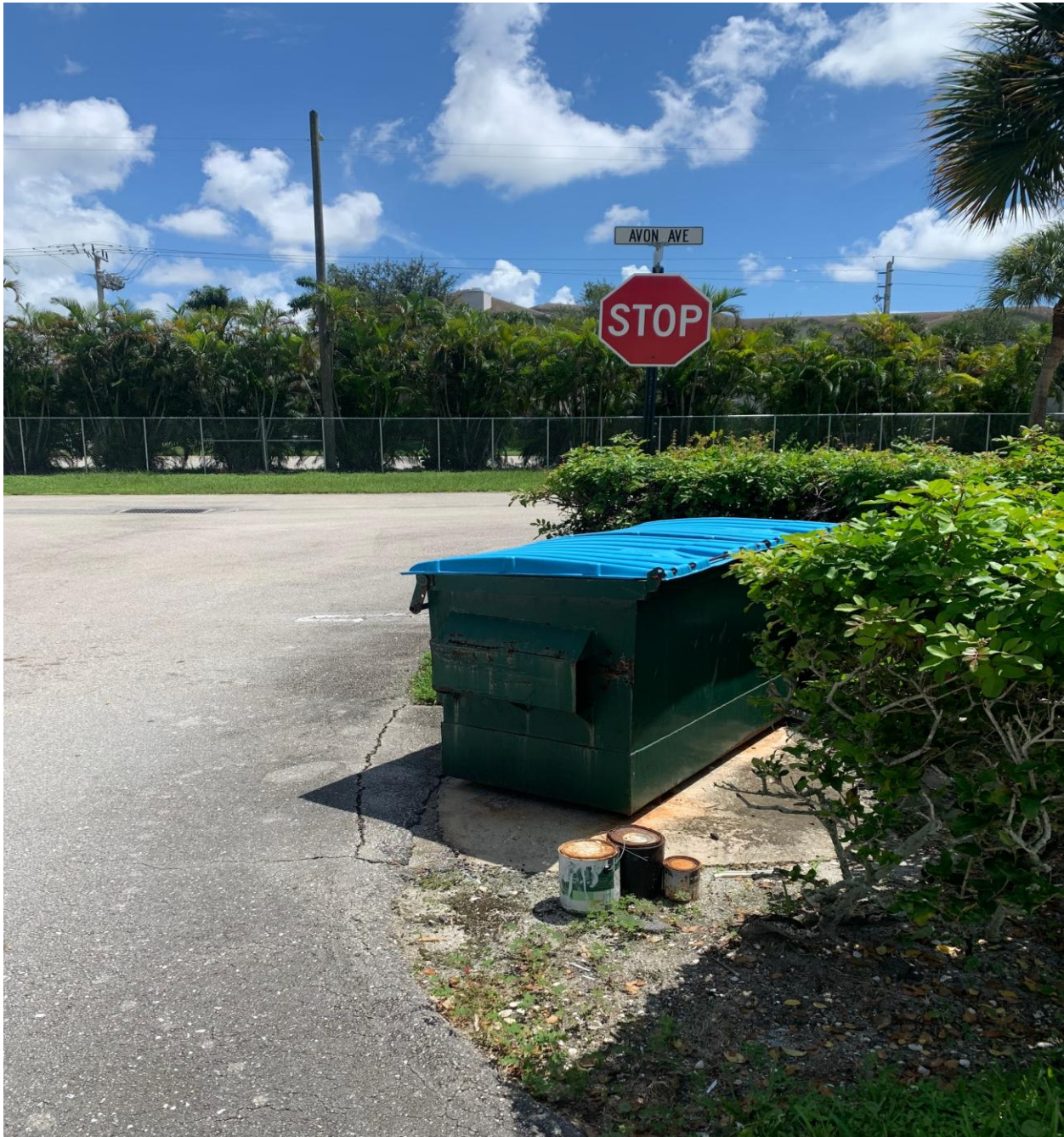
NORWICH SECTION- NEW, MANUAL COMPLIANT STOP SIGN INSTALLED BY HANDYMAN JOSE. FADED STOP BAR WILL BE PAINTED AS WELL.
