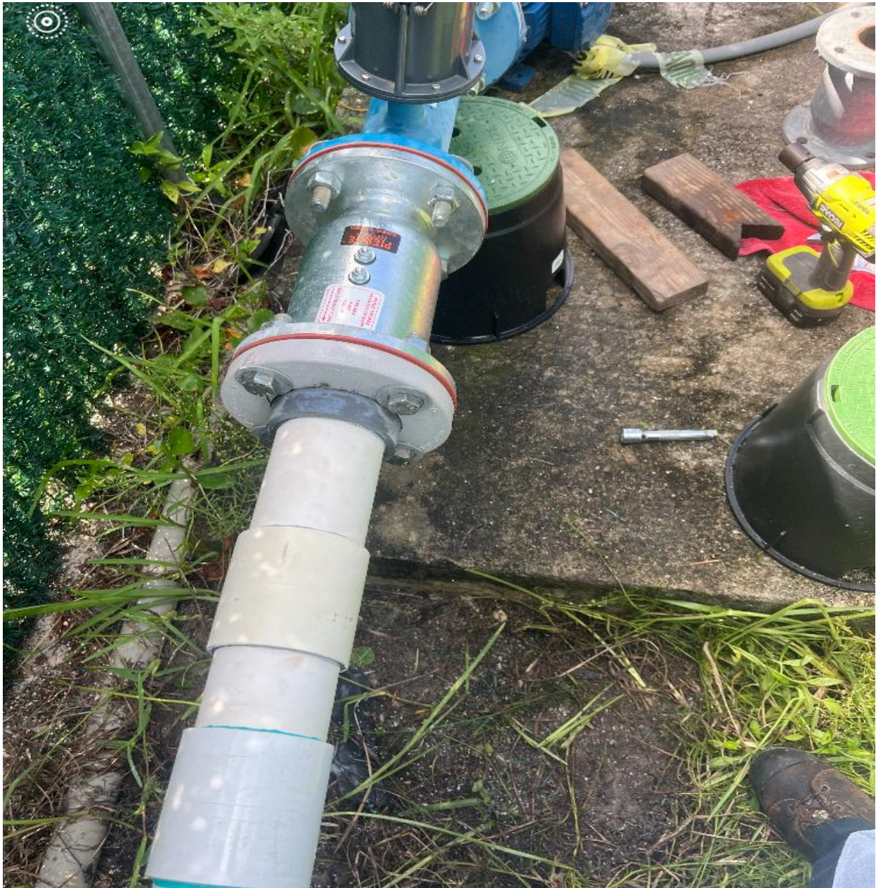
KENT SECTION- NEW CHECK VALVE INSTALLED AT THE KENT IRRIGATION BY CHABOT IRRIGATION ON 8/26.
