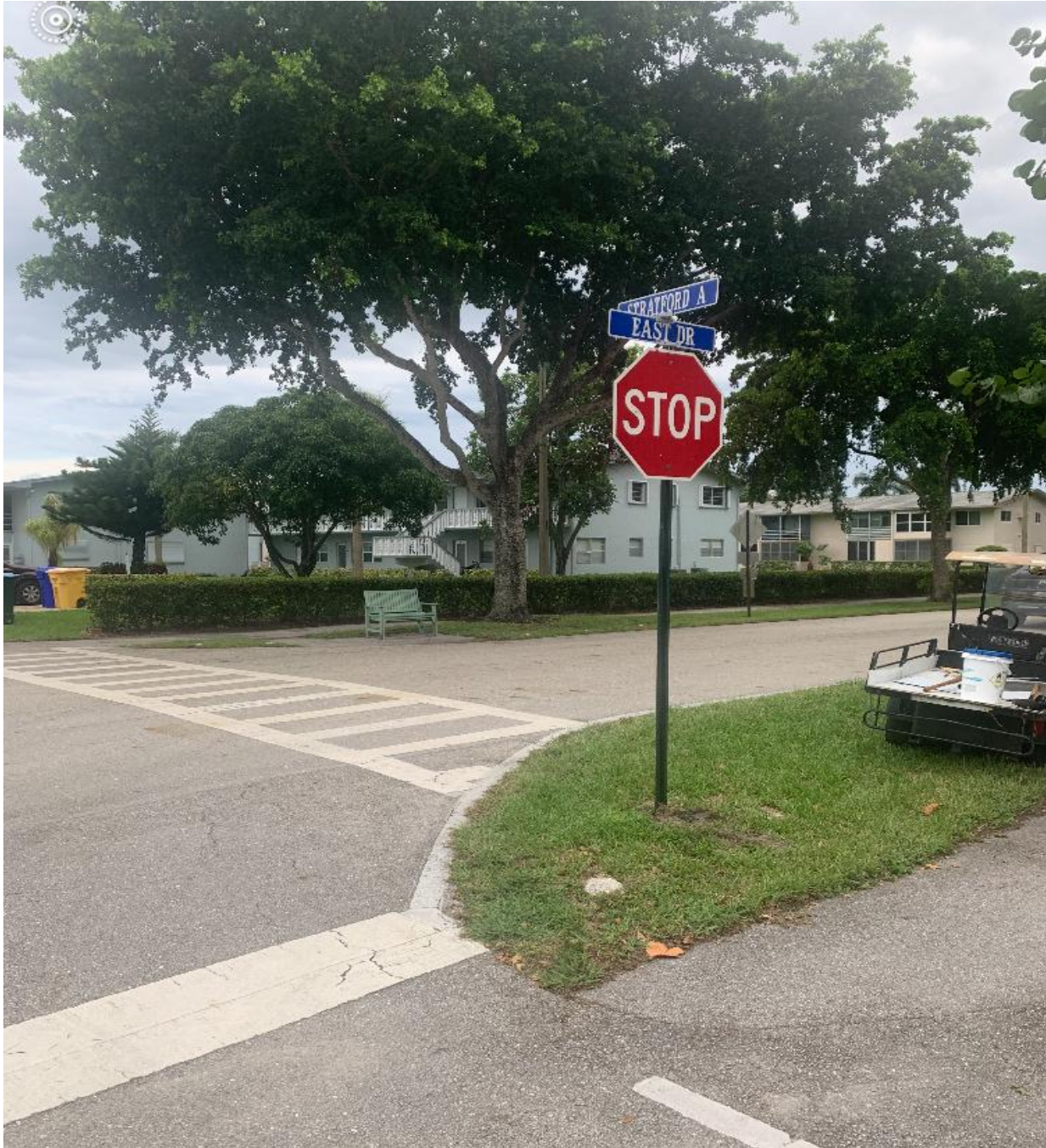
EAST DRIVE, STRATFORD A- NEW STOP SIGN AND POLE INSTALLED BY HANDYMAN JOSE.
