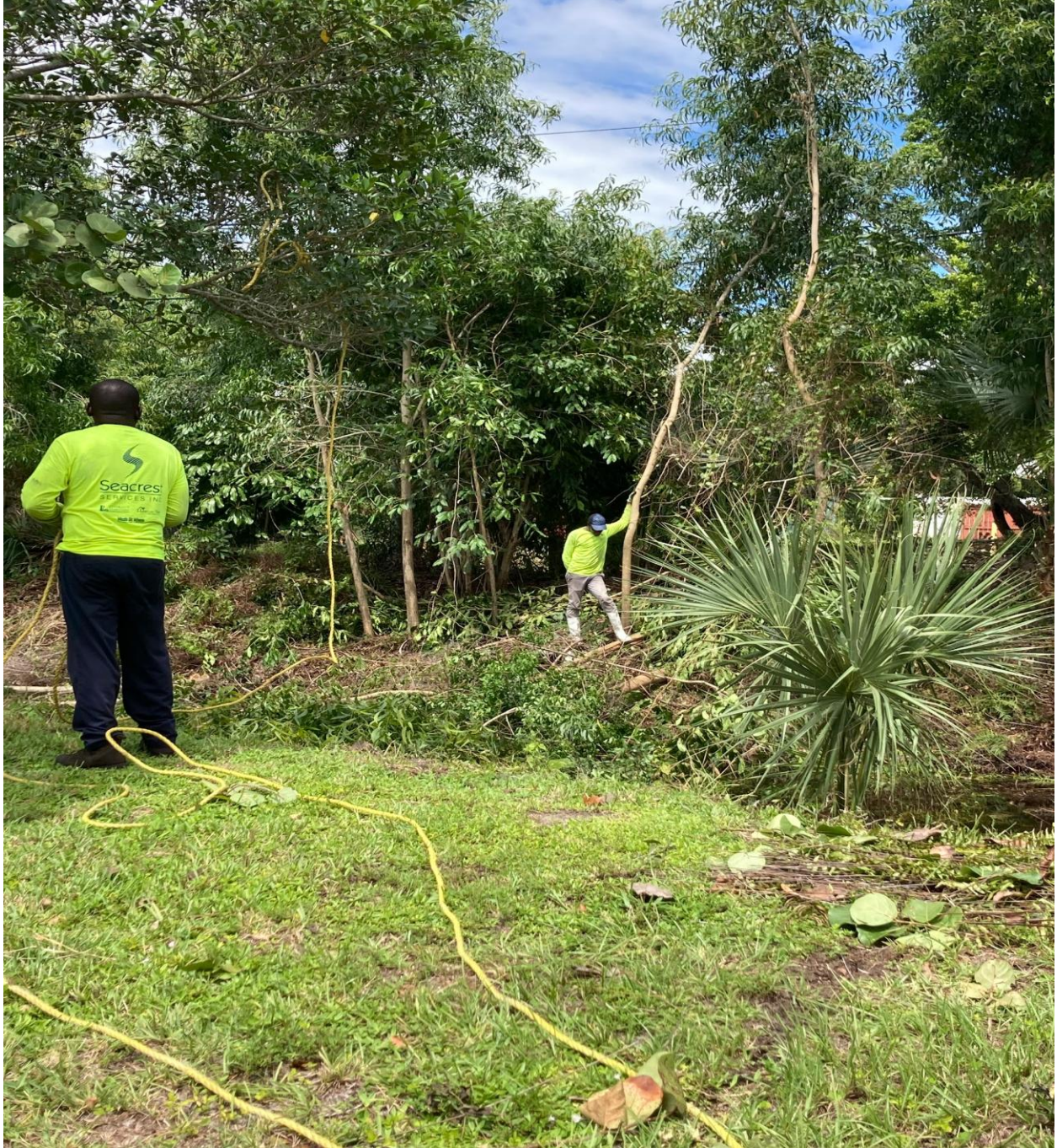
NORTH CANAL, NORWICH SECTION- REMOVING TREES FROM THE FAR SIDE OF THE CANAL IS TRICKY- THIS FELLOW ON THE FAR SIDE IS TYING ROPE TO THE CUT TREES, AND THE OTHER GUY IS PULLING THE CUT TREES OUT WITH A TRACTOR.
