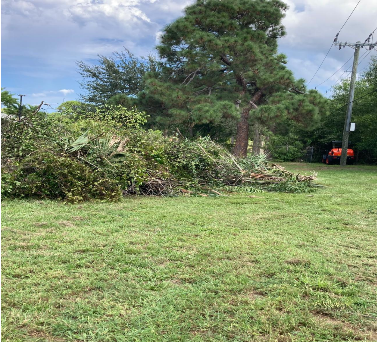
NORTH CANAL- SEACREST SERVICES HAS BEGUN REMOVING TREES, PALMS AND OTHER OVERGROWTH FROM THE NORTH CANAL.
