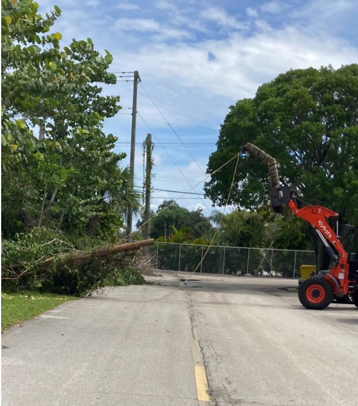
NORTH CANAL- NORWICH SECTION. TREES FROM THE FAR SIDE OF THE CANAL ARE PULLED OUT WITH A TRACTOR. SEACREST WILL CONTINUE WITH THIS WORK THIS WEEK.
