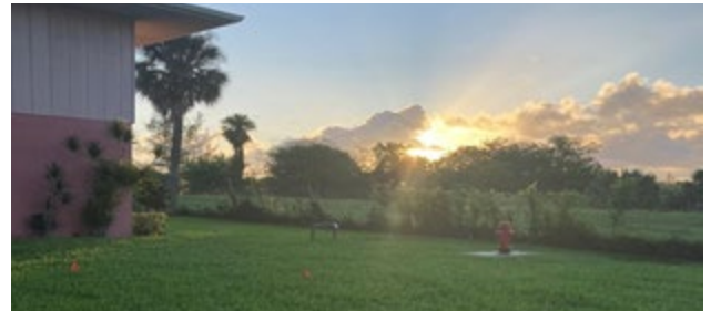
GOLFS EDGE- THE MAIN PIPE THAT BRINGS IRRIGATION WATER TO GOLFS EDGE, KINGSWOOD, AND GREENBRIER IS ON THE FAR SIDE OF THE CONSTRUCTION FENCE. THE RE-ROUTE WILL BRING THE MAIN BACK ONTO CV PROPERTY. NOTICE THE FIRE HYDRANT, BACKFLOW VALVE, AND THE LITTLE FLAGS STICKING OUT FROM THE GRASS: THESE THINGS MARK POTABLE WATER PIPES, CABLE AND TELEPHONE WIRES, AND SANITARY SEWER PIPES. THERE IS AN ELECTRIC POWER MAIN BACK THERE AS WELL. THE NEW IRRIGATION MAIN WILL NEED TO BE CAREFULLY INSTALLED TO AVOID THESE OTHER INFRASTRUCTURES.
