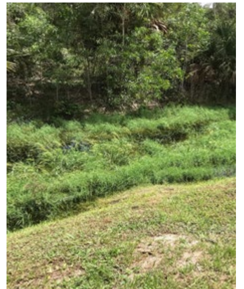
NORTH CANAL- I TOOK THIS PICTURE AT THE BACK OF THE DORCHESTER POOL IN 2017. SEDIMENT ACCUMULATION HAS ALLOWED GRASS TO GROW IN THE CANAL.
