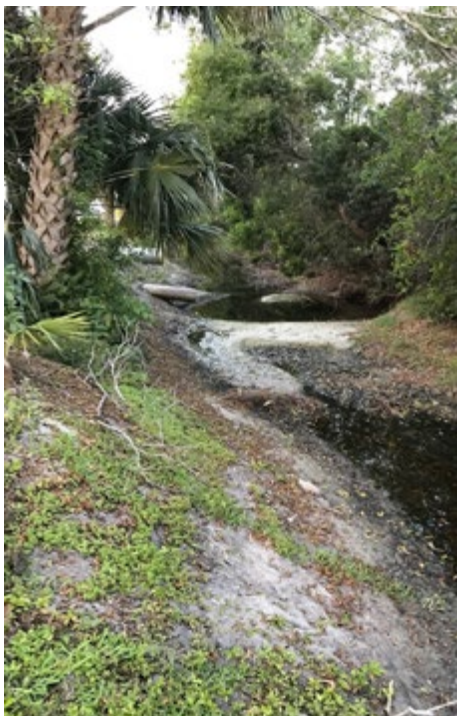
NORTH CANAL- SEDIMENT ACCUMULATION HAS CAUSED "SAND-BARS" TO GROW ALONG THE LENGTH OF THE CANAL. THIS CANAL OBVIOUSLY NEEDS TO BE DREDGED AND REGRADED, BUT SOME TRICKY LEGAL ISSUES NEED TO BE WORKED OUT FIRST.
