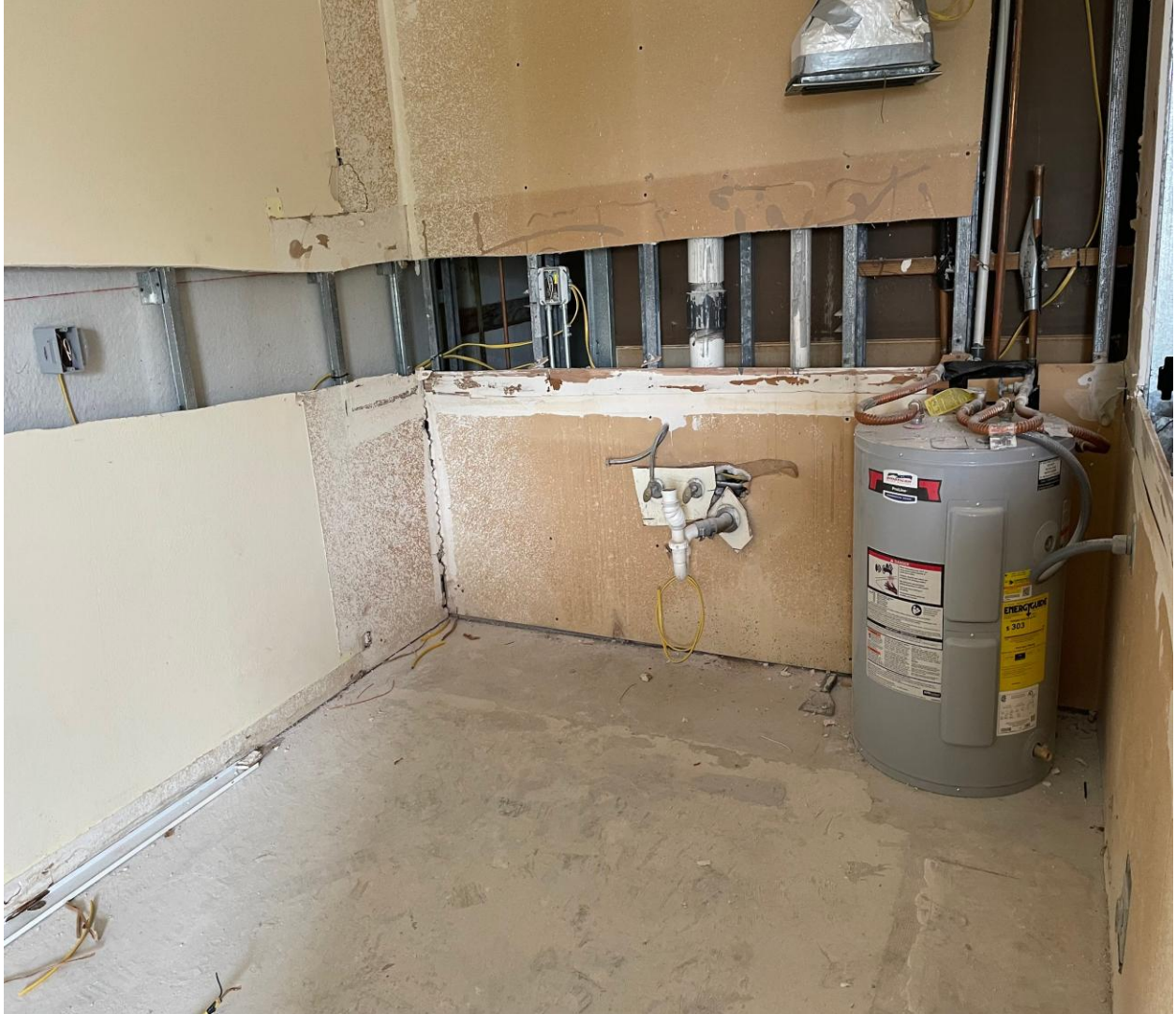
#5 HASTINGS A- UNPERMITTED PLUMBING AND ELECTRICAL WORK.
