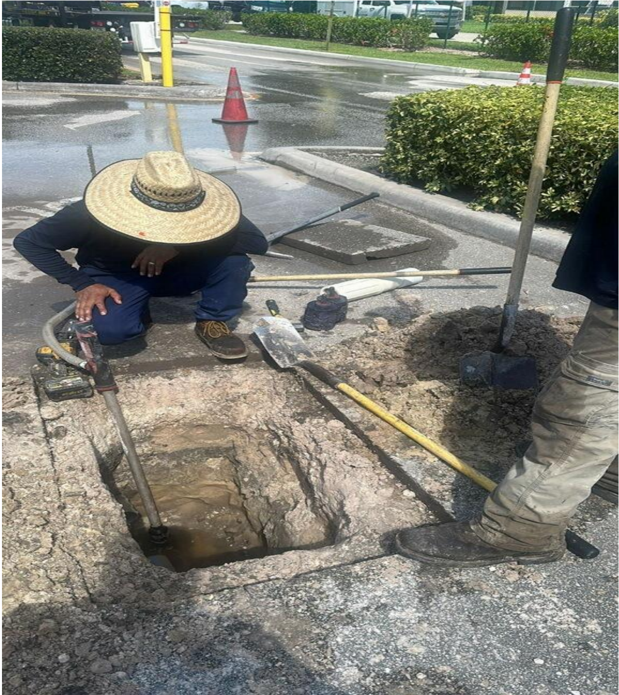
CENTURY BOULEVARD- LEAKING IRRIGATION PIPE UNDER ROADWAY REPAIRED BY SEACREST SERVICES ON 8/22.
