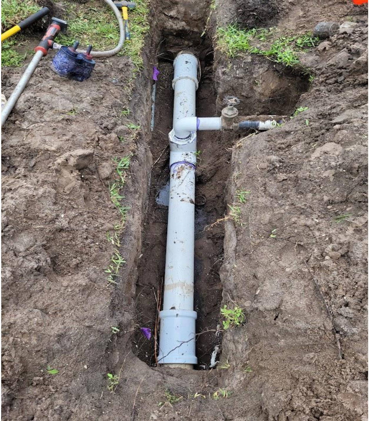
NORTH DRIVE- SEACREST SERVICES REPAIRED A SIX INCH IRRIGATION MAIN LINE ON 8/16/24.
