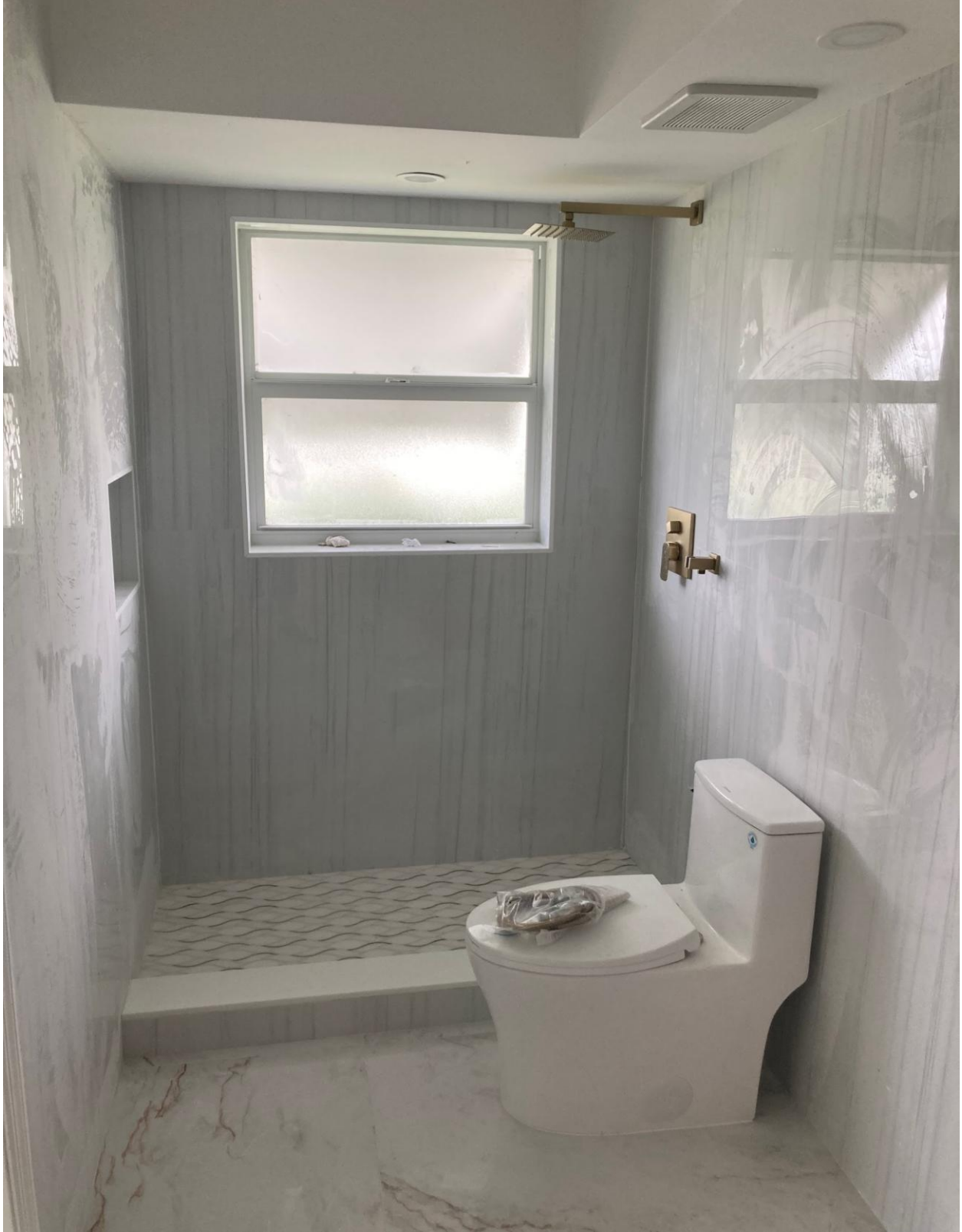
81 SOMERSET E- TUB TO SHOWER CONVERSION. NO PERMIT.
