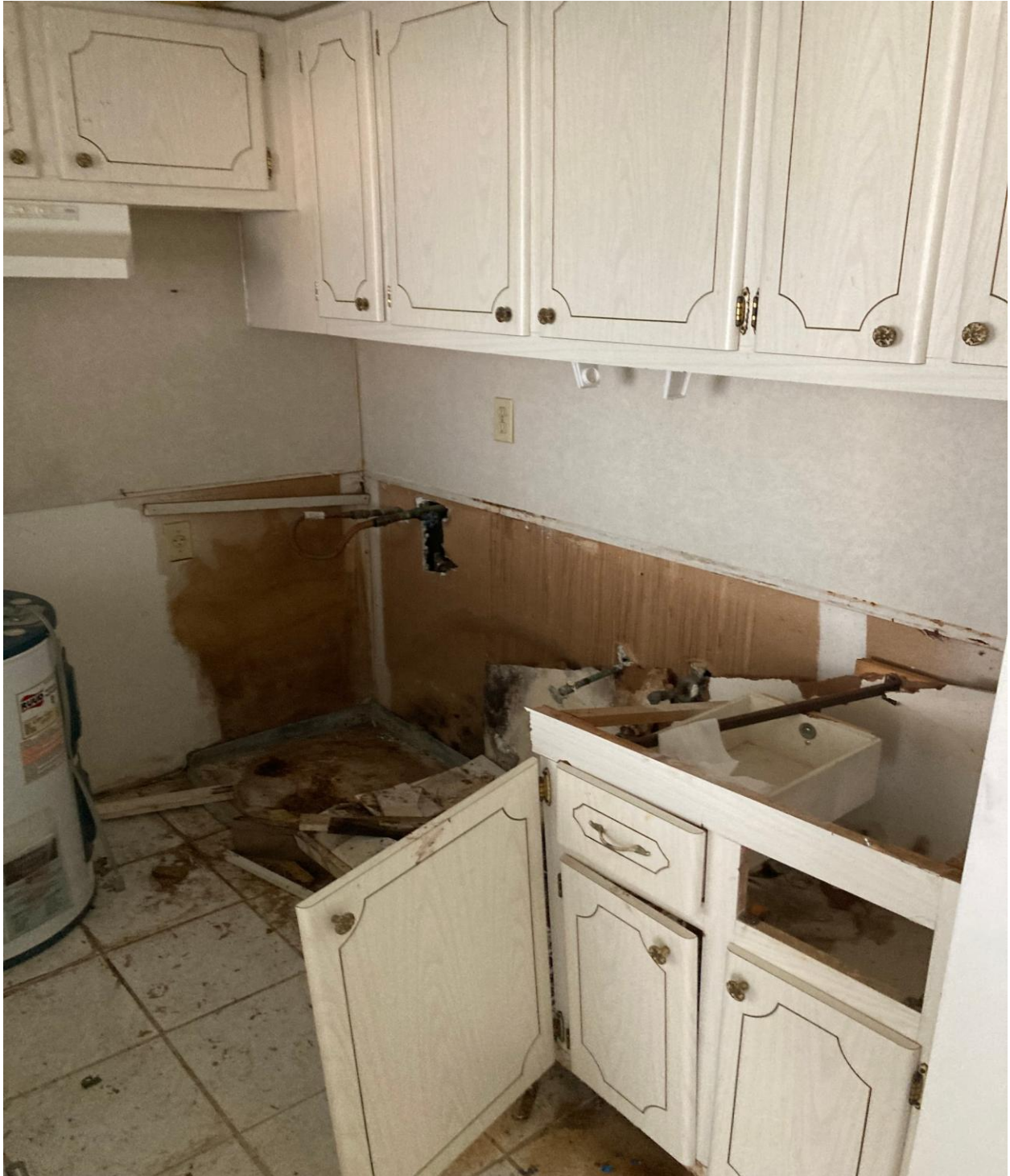
180 COVENTRY H- DAMAGE FROM A LEAK AT THIS UNIT IS LIMITED TO KITCHEN, BATHROOMS. AND FOYER. GUT WORK STARTED 8/23.
