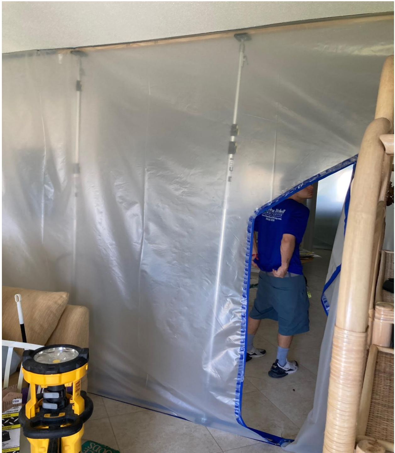
180 COVENTRY H- DEAN MITCHELL INSTALLED PLASTIC DUST WALLS TO SEPARATE THE UNDAMAGED LIVING ROOM AND BEDROOM FROM THE DAMAGED KITCHEN, BATHROOMS, AND FOYERS.
