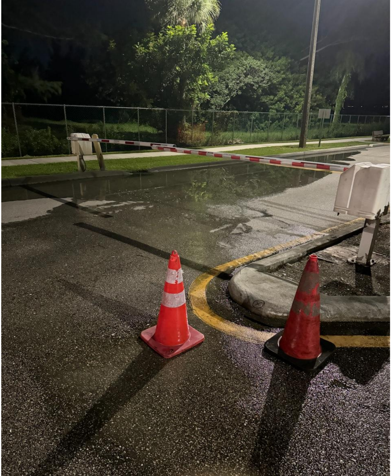
CENTURY BOULEVARD- IRRIGATION LEAK. LIKELY UNDER THE ASPHALT. SEACREST WILL FIX.
