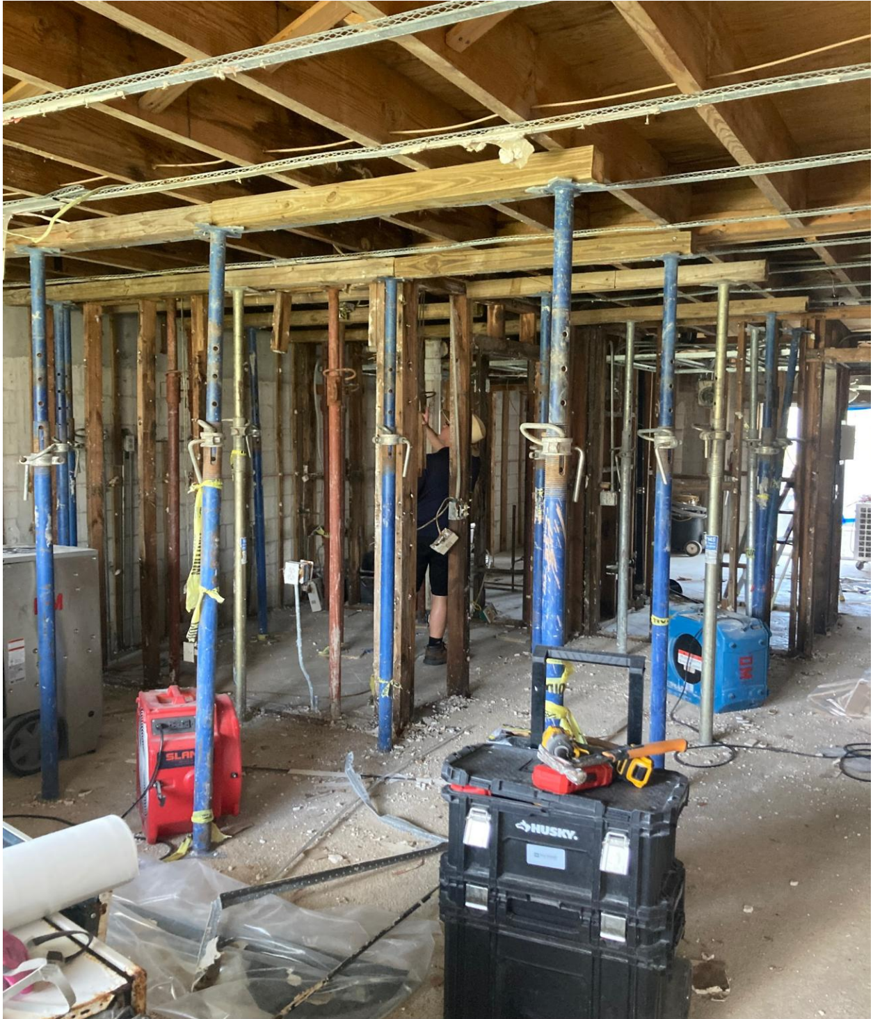
170 COVENTRY H- GUT WORK CONTINUES. ADDITIONAL POST SHORES WERE INSTALLED TO KEEP THE CEILING FROM COLLAPSING.
