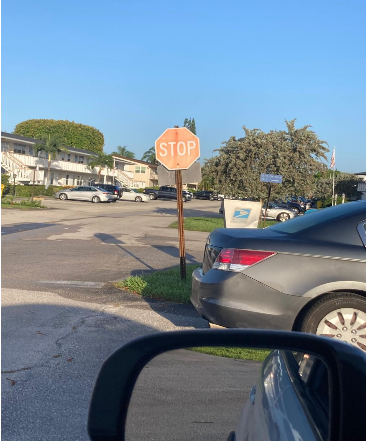
ASTOR STREET, KENT SECTION- FADED STOP SIGN, CROOKED SIGNPOST, FADED STOP BAR. JOSE WILL FIX.
