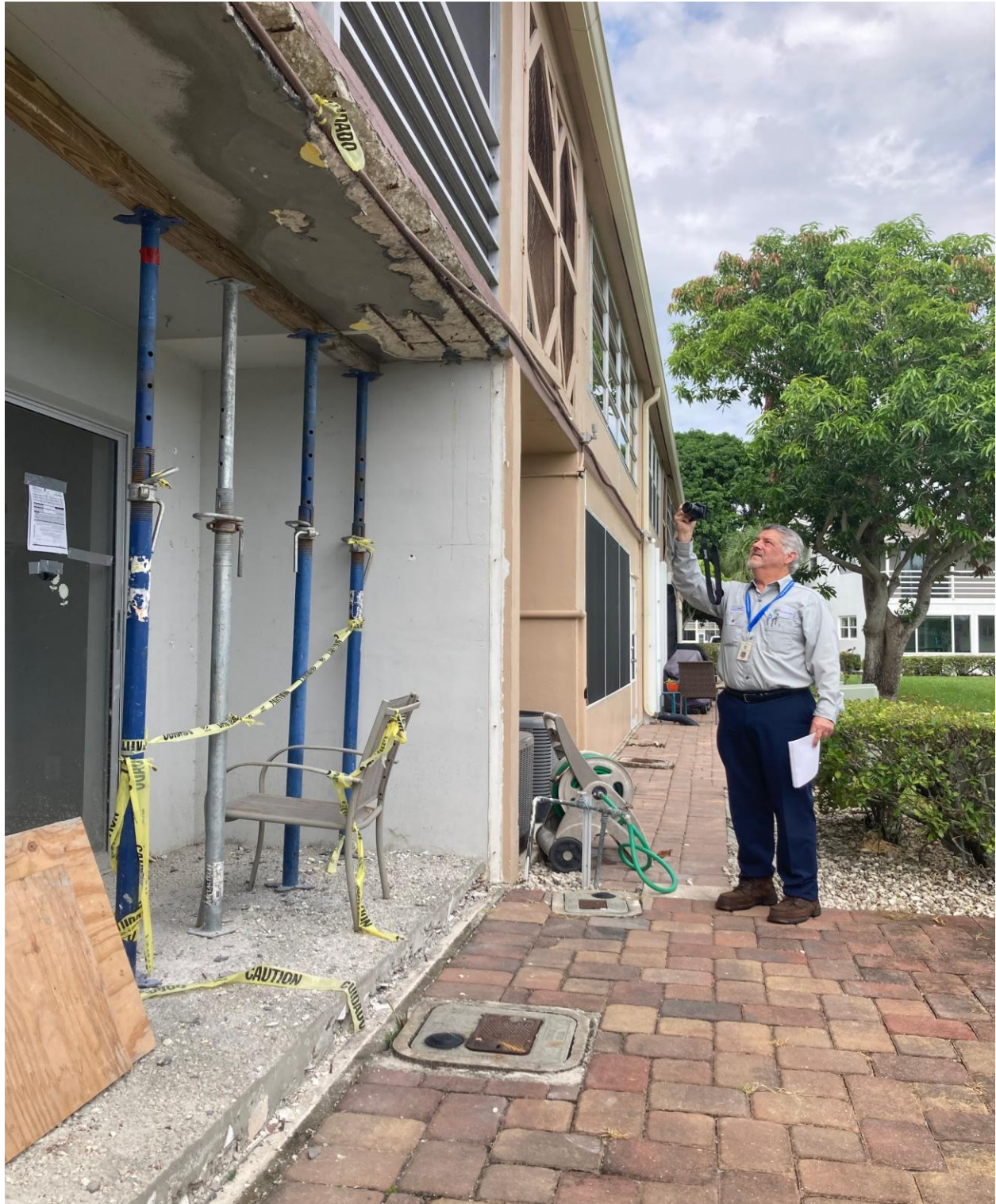
204 SOMERSET K- PZB INSPECTOR TOM BANZHAF DOCUMENTS THE ADDITIONAL STRUCTURAL DAMAGE CAUSED BY ACD INST CORP. CONTRACTORS ON 8/15.
